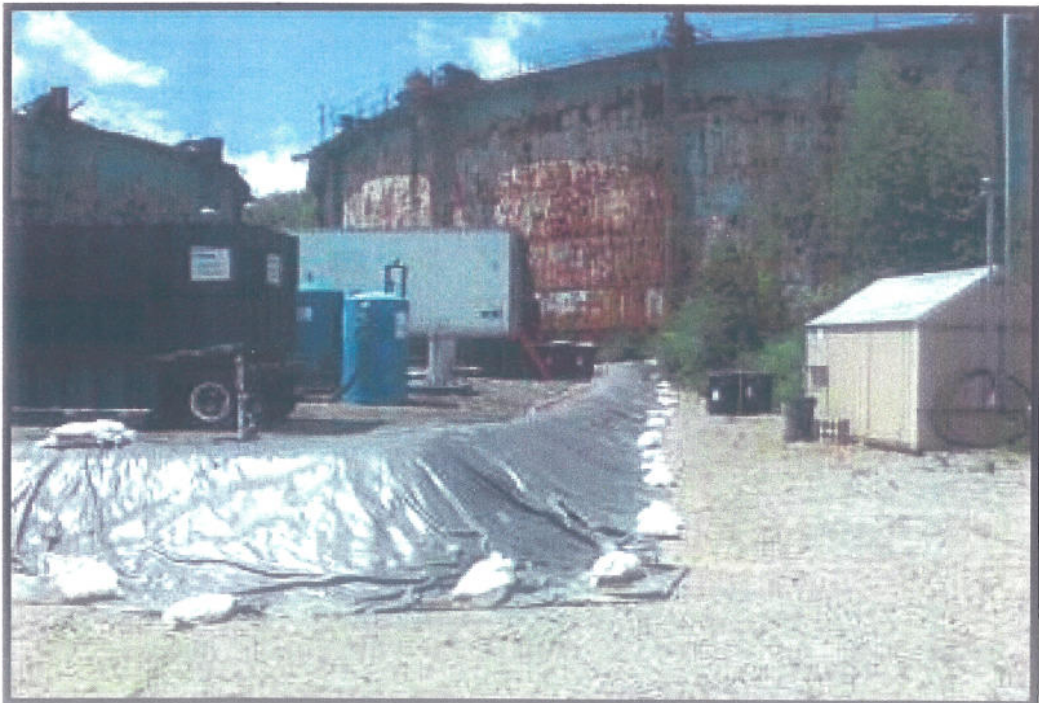
Photo 2: Frac-Tank 2 with Discharge Line Removed and Carbon Trailer With Discharge Line Removed and Electric Service Disconnected
