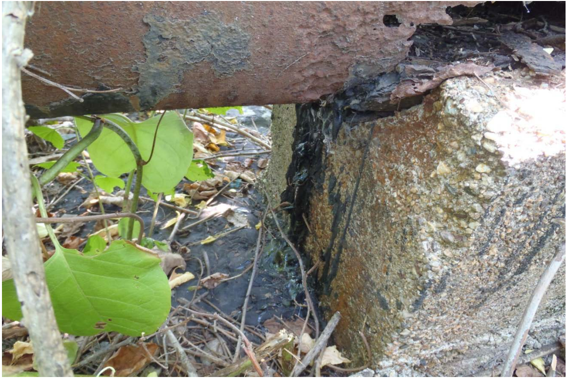
Photo 3: Close-up of damaged pipe and associated pipe leak.
