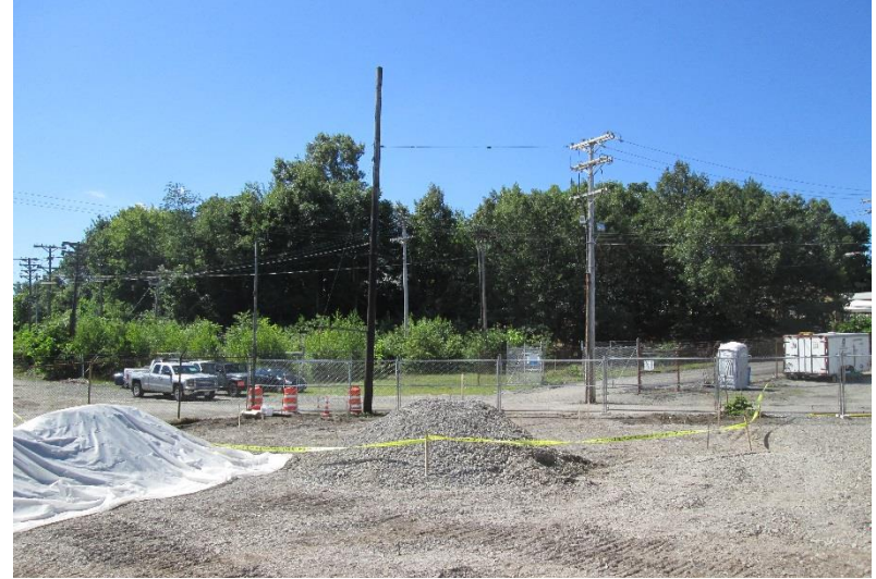
PHOTOGRAPH 6 – Looking southwest, after hydraulic fluid excavation clean-up
