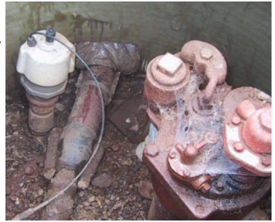
Sumps with missing entry fittings causing leaks
