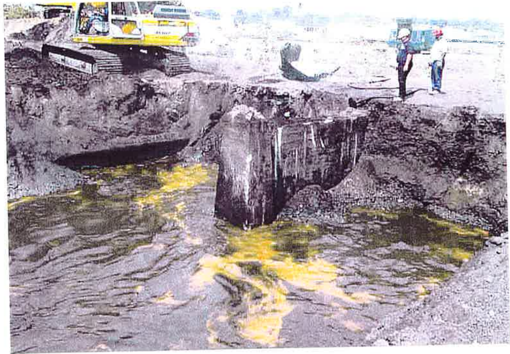
Northeast wall of Area 3 subsurface soil excavation. Note approximately 12 inch pipe below excavator, presumed to be a water pipe.
