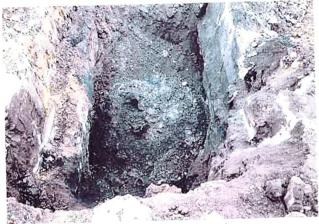
Soil conditions proximate to knockdown pipe.
