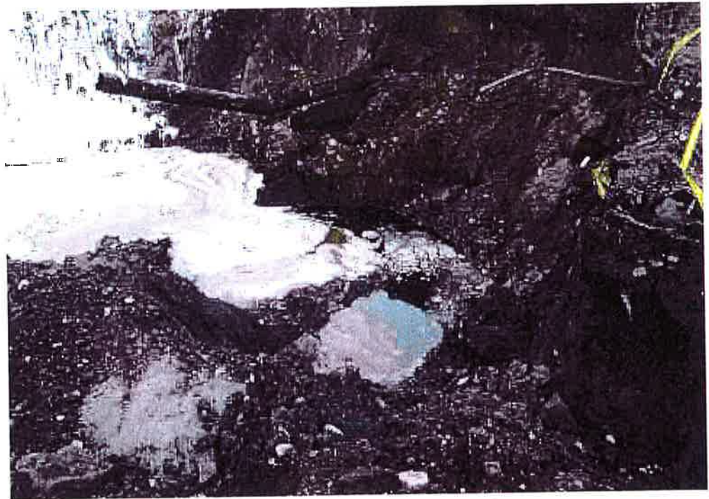
LNAPL from north wall of Area 2 excavation.
