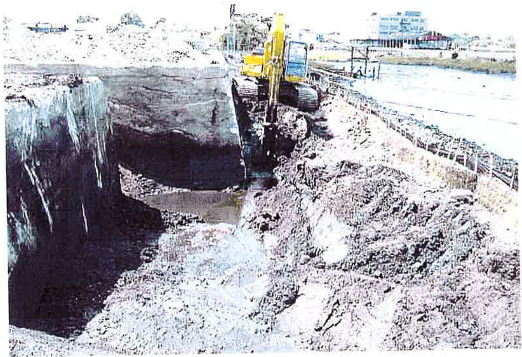
Seep area excavation with north sides of Structure 14A in foreground and Structure 17 next to excavator.
