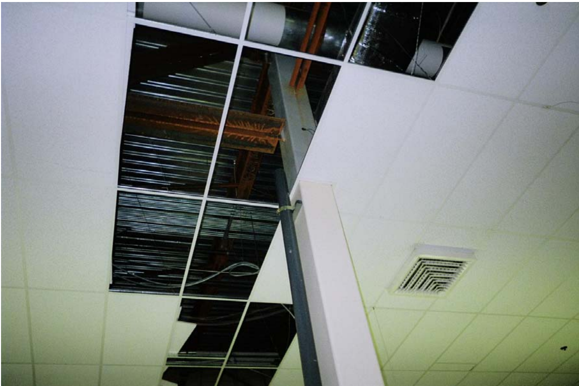
Drop Ceiling Penetration
