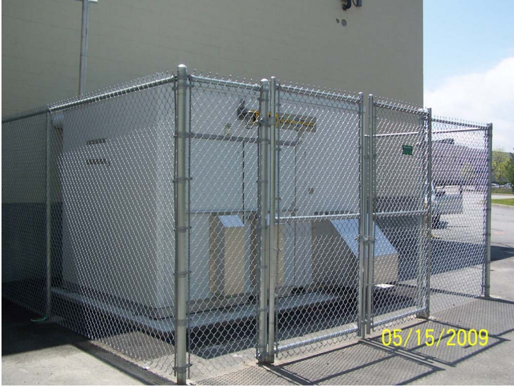
ASD Enclosure Inside 8 ft Chain Link Fence
