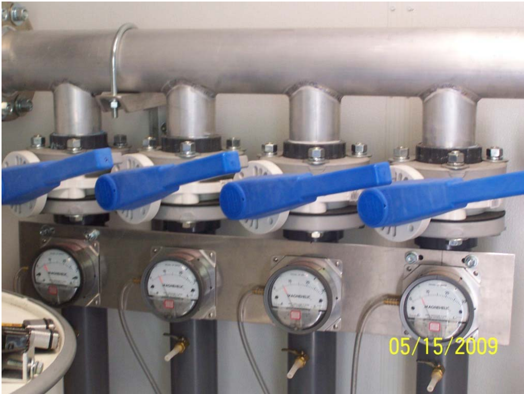
Extraction Well Piping at Manifold Inside ASD Enclosure
