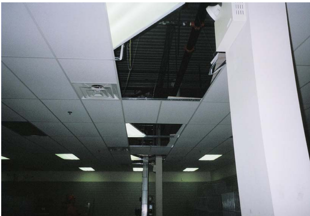
EW-6 Above Drop Ceiling
