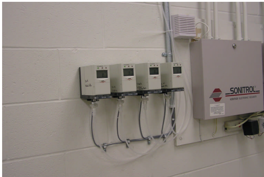
Photo 8: View of 4 methane sensors located in east wing maintenance office.
