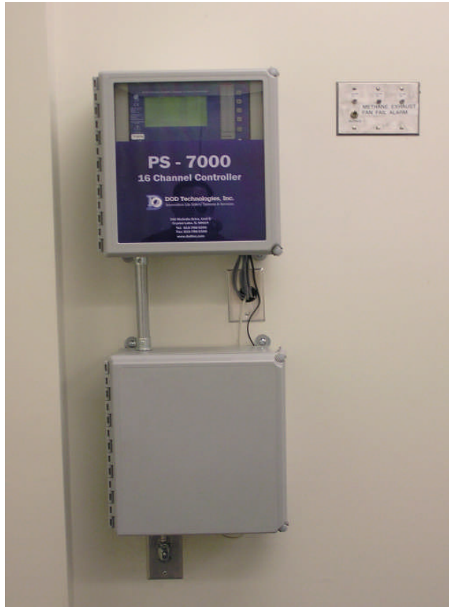
Photo 7: View of indoor methane monitoring system controller. Auto dialer is located in the grey control box. Integrated rooftop fan alarm panel is seen in the upper right corner of photo.
