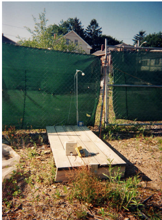
Photo 2: View of dust sampling and field monitoring apparatus used during intrusive activities.
