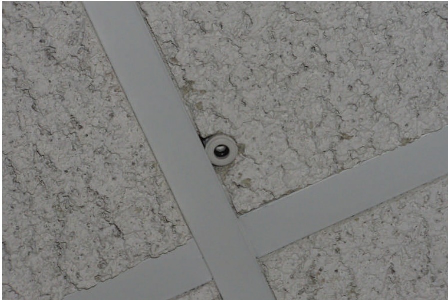
Photo 10: Typical view of interior sampling port located within acoustical ceiling tile and connected to one of the continuous methane sensors.
