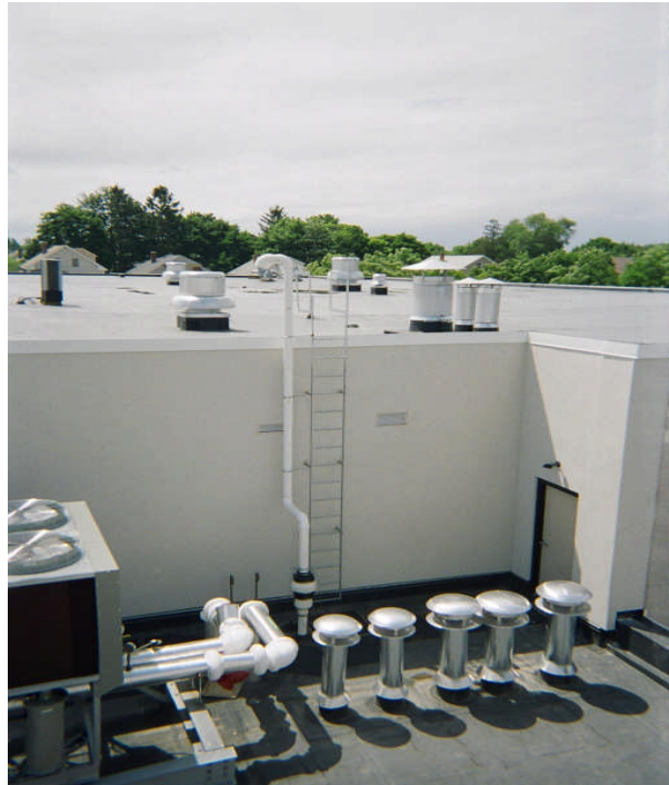
Photo 14: View of roof-top fan #2 above lower roof. Vertical exhaust pipe with discharge above elevated roof line.
