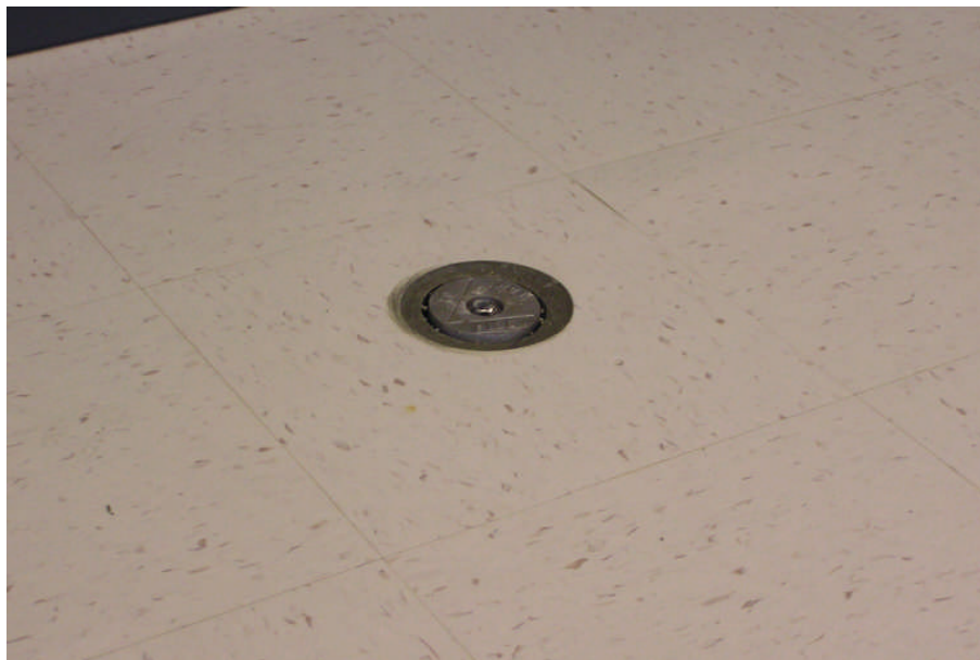
Photo 34: Typical interior monitoring probe completion photo illustrating concrete surface seal and small diameter protective road box with rubber gasketed cover.
