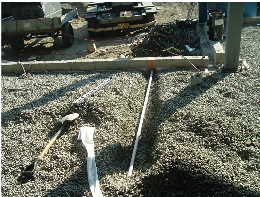
Photo 6: Typical sub-slab monitoring point progress photo. White filter fabric material to be installed over screened portion of monitoring point is visible to the left of the PVC piping.
