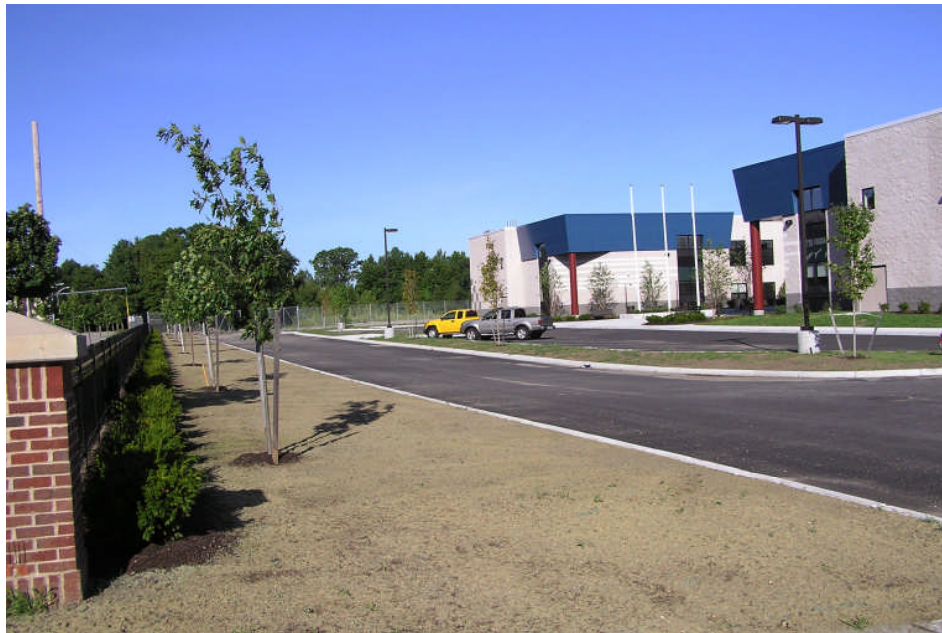
Photo 26: Cap completion photo illustrating loamed, landscaped, and paved areas south of building.
