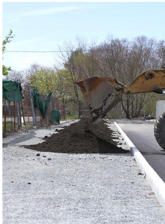
Photo 24: Cap construction progress photo in the vicinity of the southern property line illustrating loam placement on top of dense graded base fill material.
