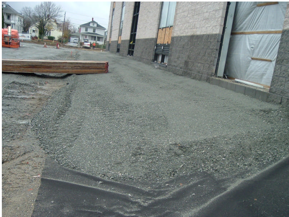
Photo 16: Cap construction progress photo along east side of building illustrating clean fill over ProPex geotextile fabric in future landscaped area.
