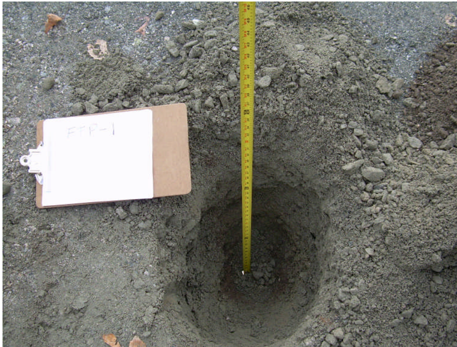
Photo 21: Photo of measured cap thickness prior to loam placement in the vicinity of the northern property fence line illustrating compliance with minimum fill thickness requirements.
