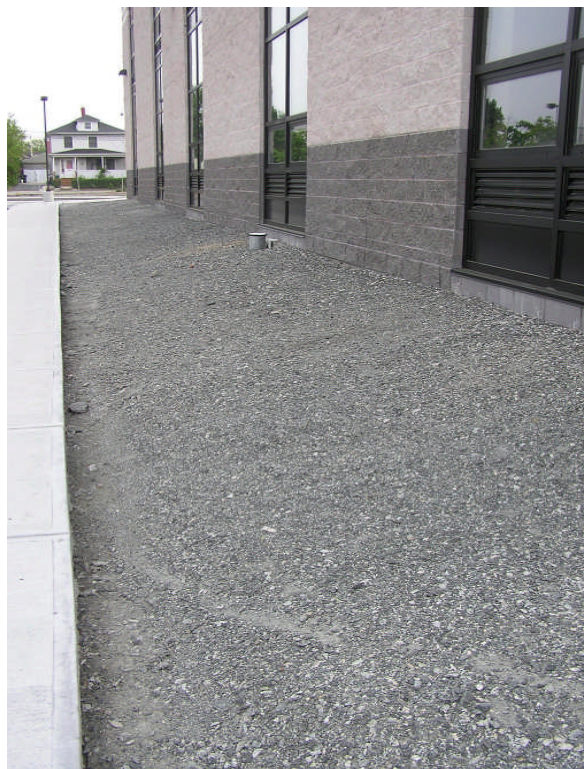
Photo 20: Cap construction progress photo of east side of building illustrating graded clean fill material prior to loam placement. Protective road box associated with MP-8 is visible near the base of the building.
