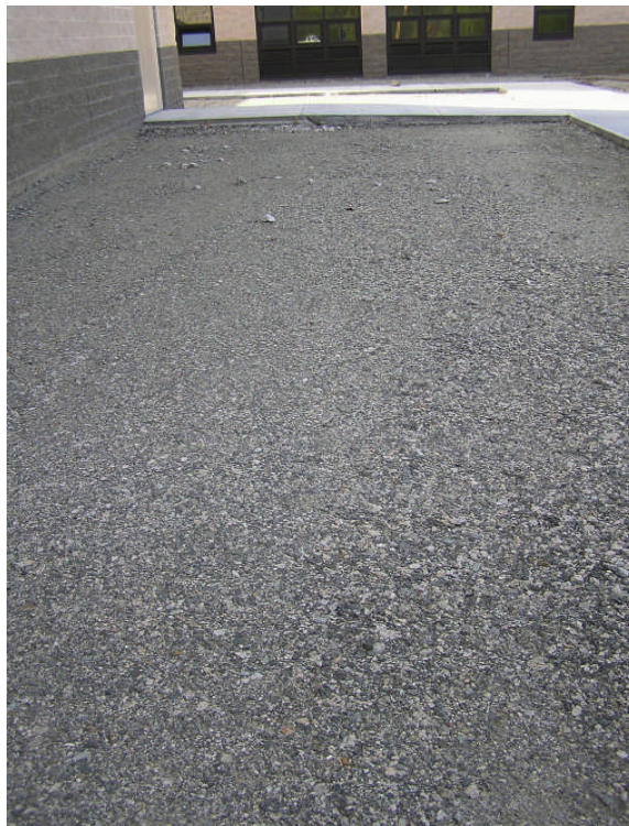
Photo 18: Cap construction progress photo of west side of building illustrating graded clean fill material prior to loam placement.
