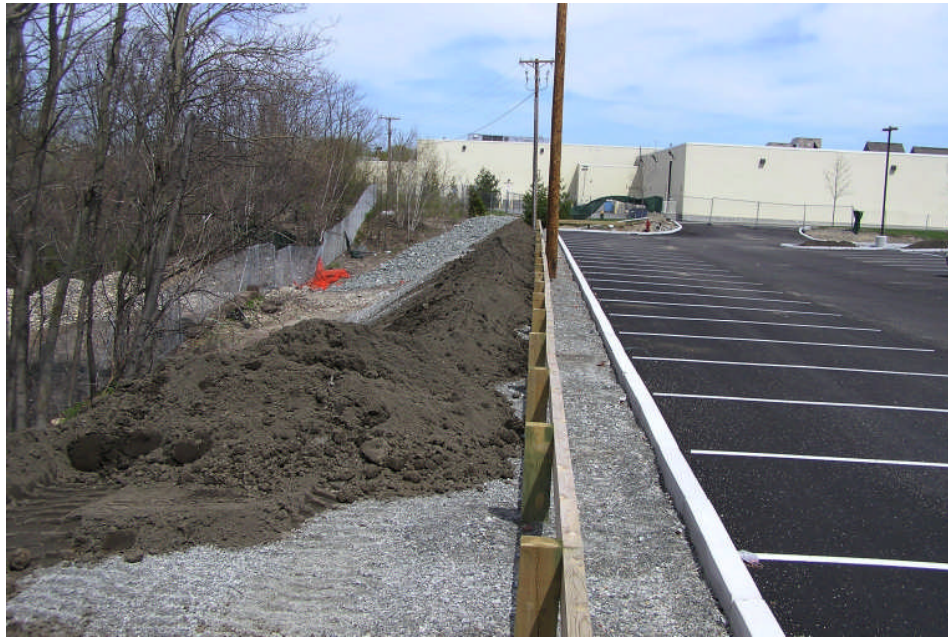
Photo 23: Cap construction progress photo in the vicinity of the northern property line illustrating loam placement on top of dense graded base fill material, and paved surfaces.
