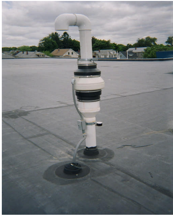
Photo 13: Close-up view of roof top suction fan associated with sub-slab depressurization system.
