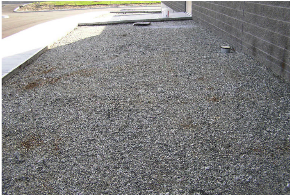
Photo 19: Cap construction progress photo of north side of building illustrating graded clean fill material prior to loam placement. Protective road box associated with MP-2 is visible near the base of the building.
