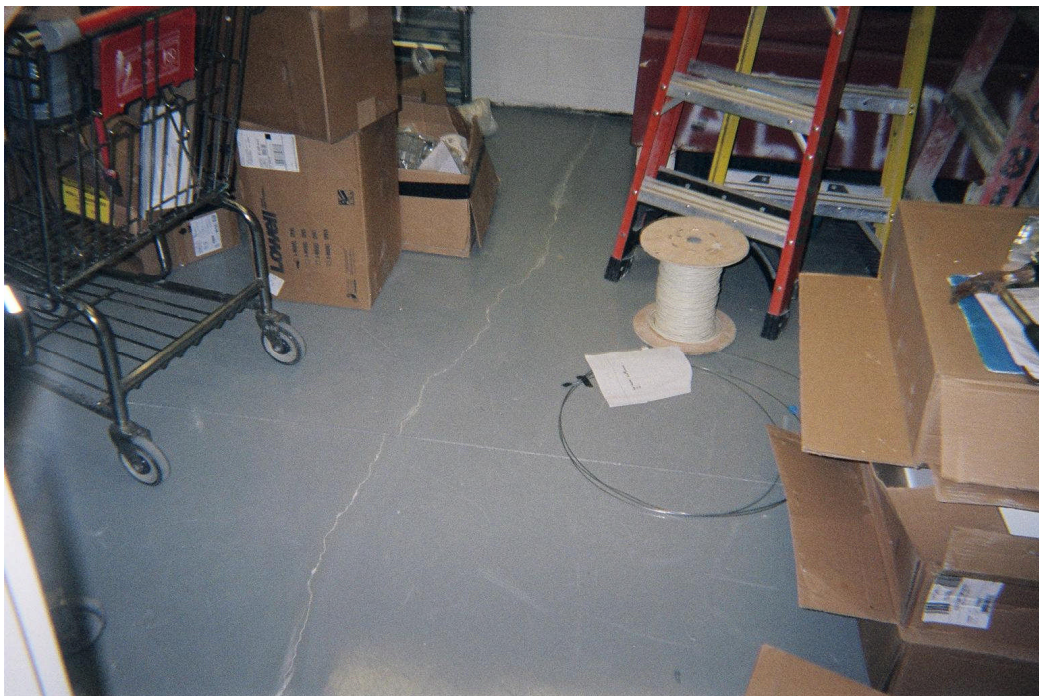
Photo 12: Typical view of sealed crack in concrete slab.
