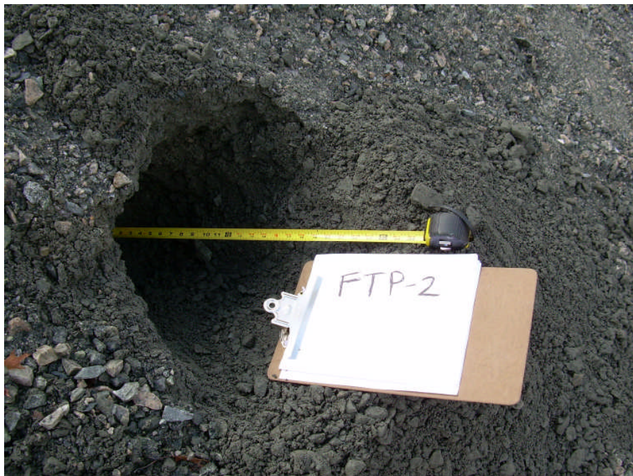
Photo 22: Photo of measured cap thickness prior to loam placement in the vicinity of the northern property line at the base of the sloped cap illustrating compliance with minimum fill thickness requirement.
