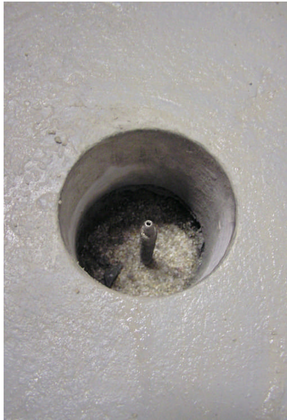
Photo 33: Progress photo of interior monitoring probe installation prior to installation of surface seal.
