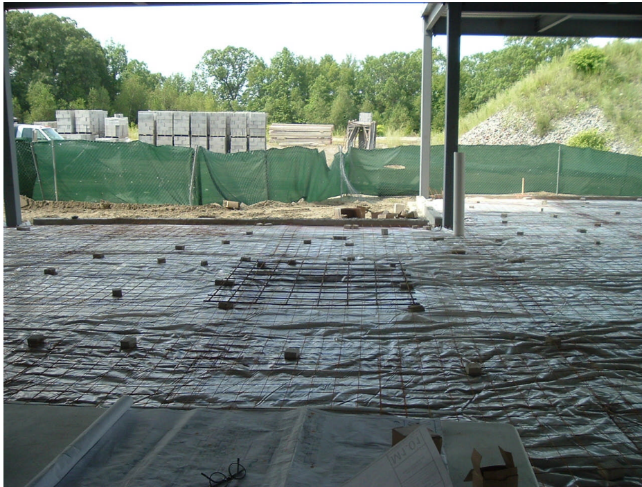
Photo 5: Typical suction pit progress photo illustrating final stage of construction just prior to pouring of concrete floor. Rebar has been installed over top of suction pit, and 6-mil polyethylene barrier shown beneath steel mesh used to strengthen concrete..
