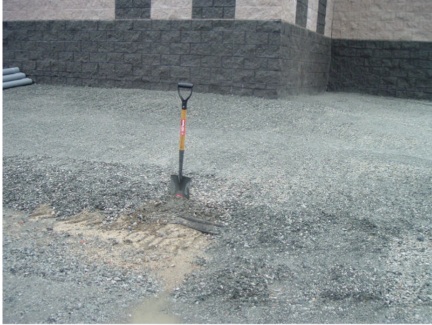
Photo 17: Cap construction progress photo in vicinity of southeast corner of building illustrating clean fill over ProPex geotextile fabric in future landscaped area.
