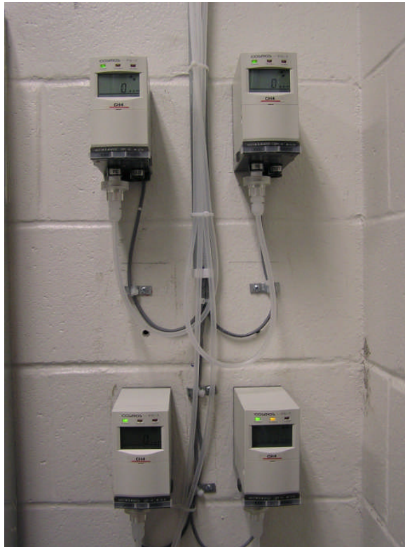
Photo 9: View of 4 methane sensors located in west wing electrical room.
