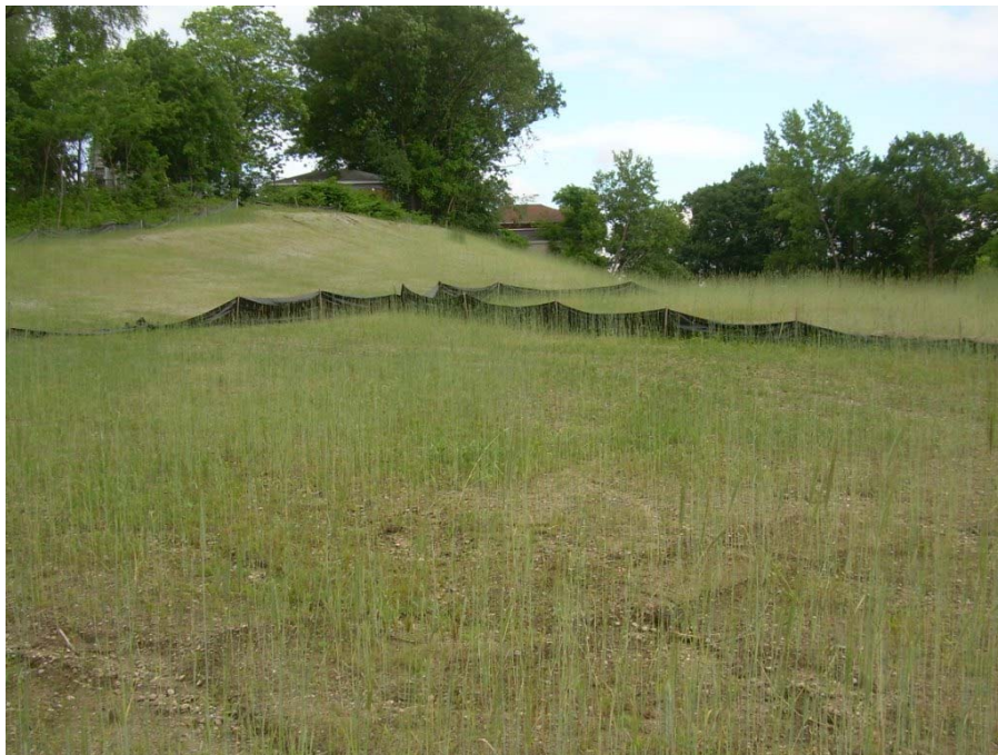
Photo 10: View of landfill cap with demonstrating establishment of vegetative cover. (Photo taken June 2007)
