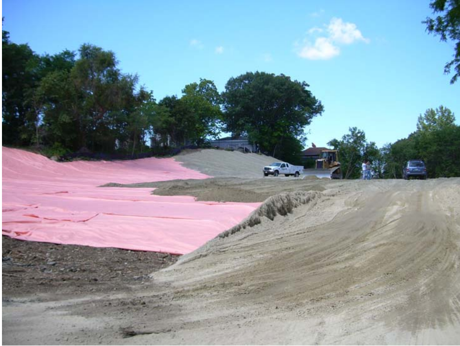
Photo 3: View of landfill cleared of vegetation. Subgrade has been prepared and geotextile fabric is being installed over the subgrade.
