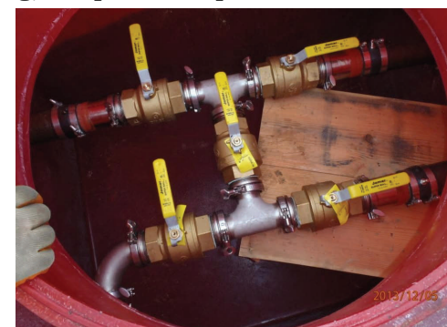
Plumbing observed within a newly installed sump. Storm water collecting in the sump during construction is removed before the sump goes into service.
