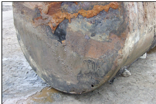
The fuel oil UST shown in the photograph to the left demonstrates the poor condition in which many USTs are found. Corrosion and holes are easily observed, with pitting visible on closer inspection. Based on the condition of the tank and the presence of stained soils, RIDEM required a closure assessment for this UST.
