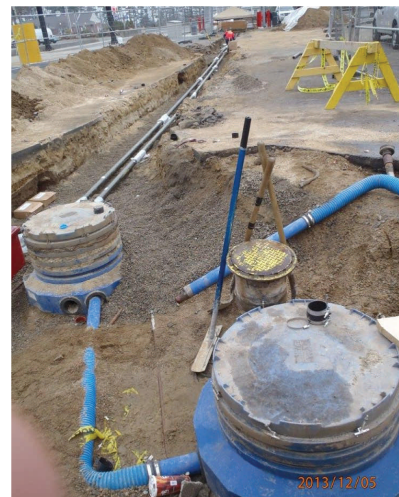
Upgrades at the Travel Center facility included the installation of a diesel tank, piping, sumps and dispenser units.
