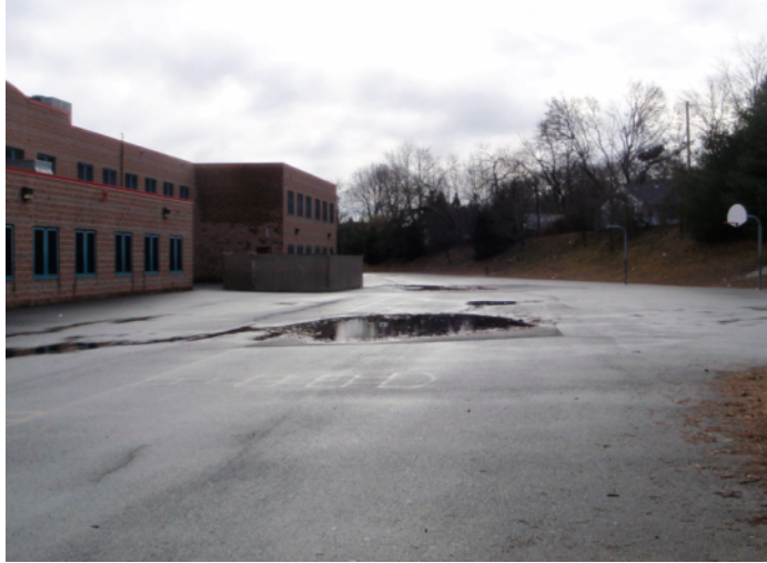
#7: Pooled water in the parking lot behind the elementary school.
