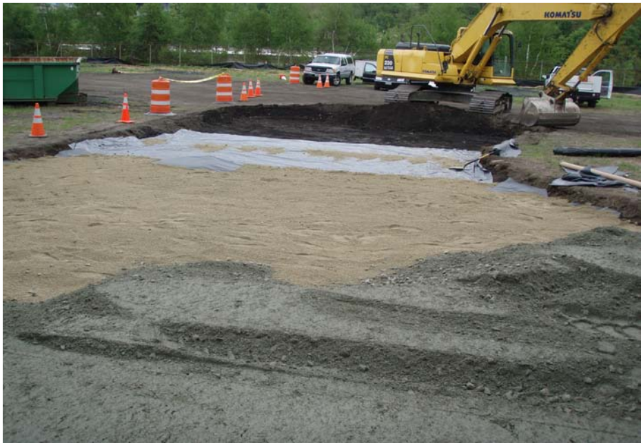
Photo No. 9 - T-Ford placing poly liner, bedding sand and processed material within eastern portion of work area in May 2010.
