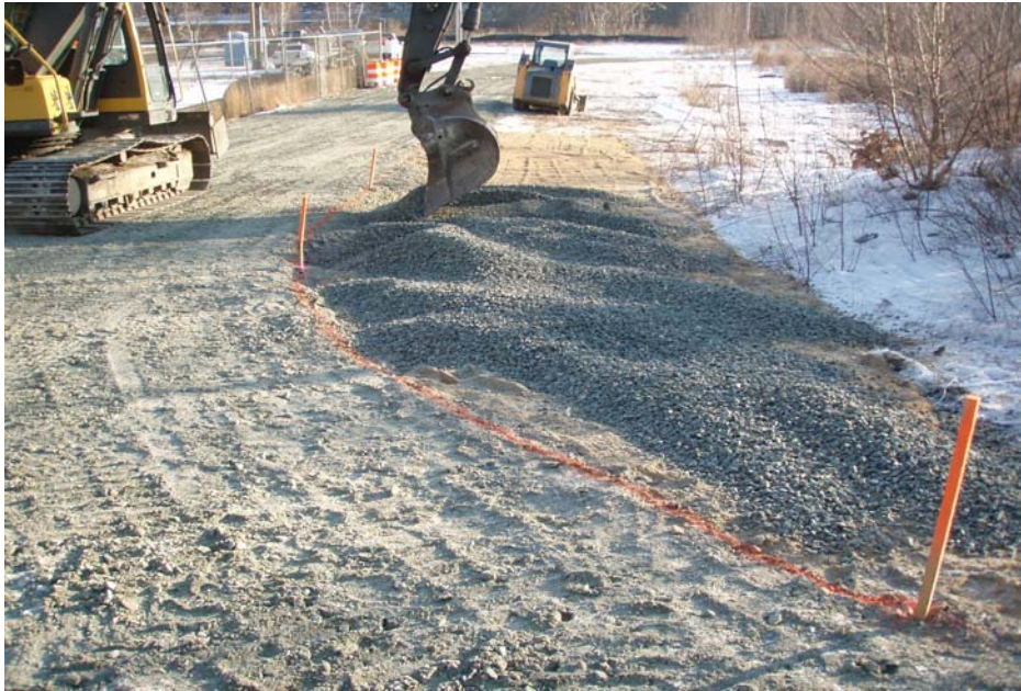
Photo No. 5 - T-Ford spreading lift of trap rock over the low lying area located on the southern side of the roadway (January 2010)
