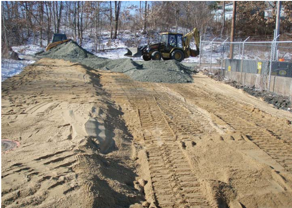
Photo No. 4 - T-Ford spreading out processed gravel layer above bedding sand (January 2010).
