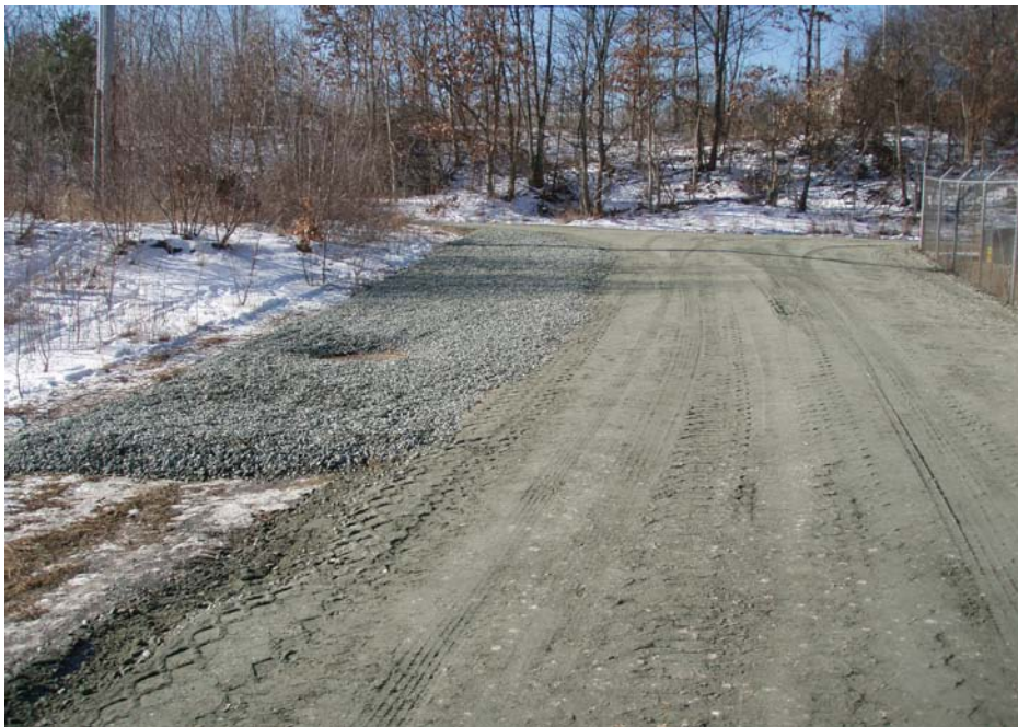
Photo No. 6 - Restored roadway and low lying cap area at completion of work in January 2010.
