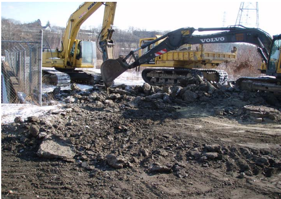
Photo No. 2 - T-Ford breaking up frost in roadway in western portion of work area (January 2010).
