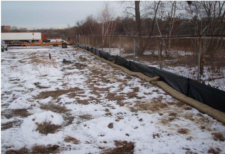
Photo No. 1 - Silt fence and hay bales installed down gradient of work area along fence adjacent to Seekonk River.
