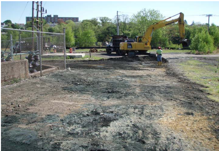
Photo No. 8 - T-Ford continues excavating roadway in May 2010. Blue stained ash-organic like material within 2 to 3 inches ground surface within roadway area.
