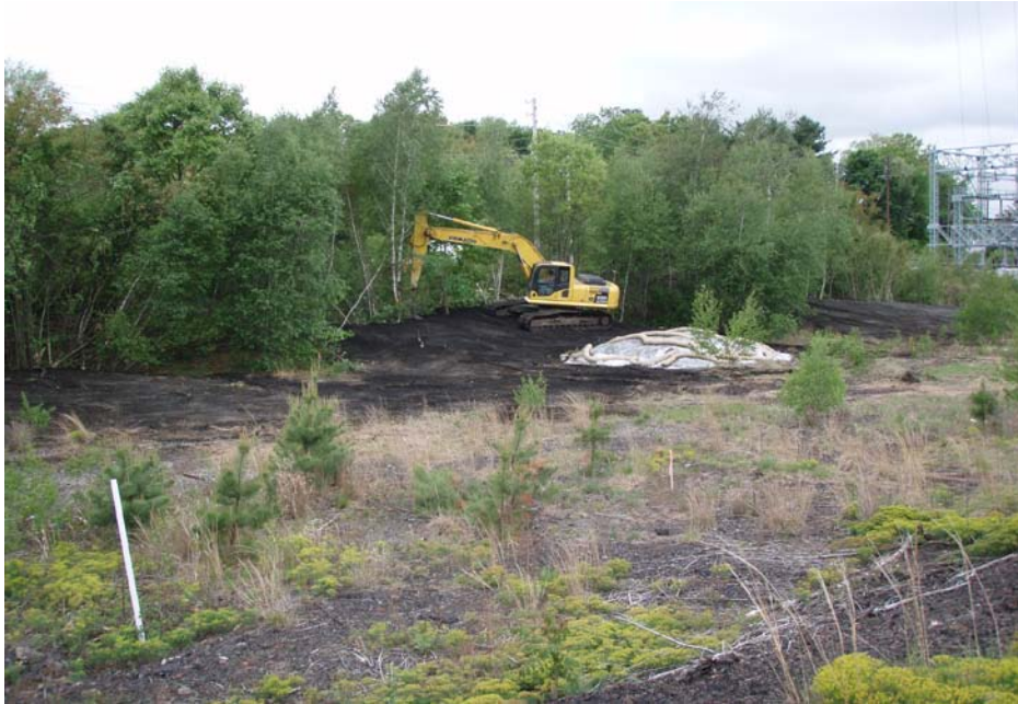
Photo No. 13 - T-Ford regrading excavated roadway and parking area material within relocation area (May 2010). Blue-stained material stockpile from January 2010 work is located in the foreground.
