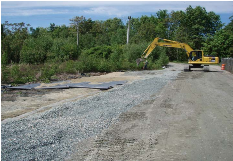
Photo No. 11 - T-Ford extending low lying area cap south and east of original work limits (May 2010).
