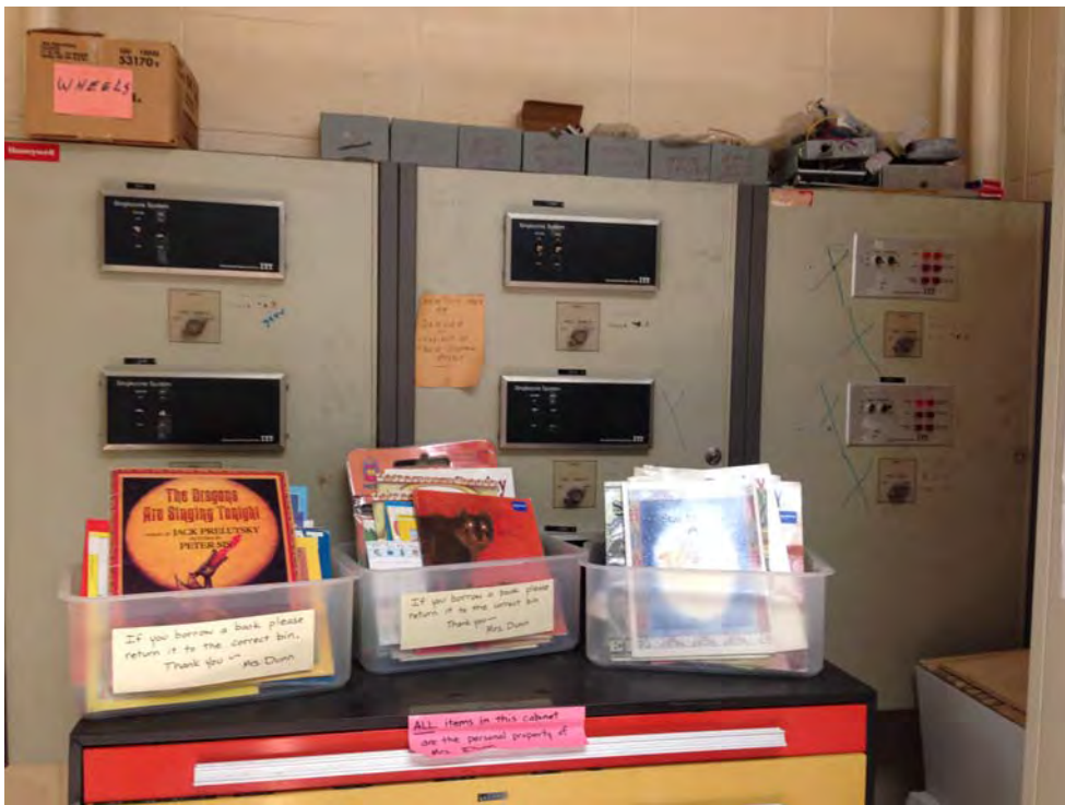
Photograph No. 18 Inactive circuit breakers from heating system before forced hot water heating system was installed.
