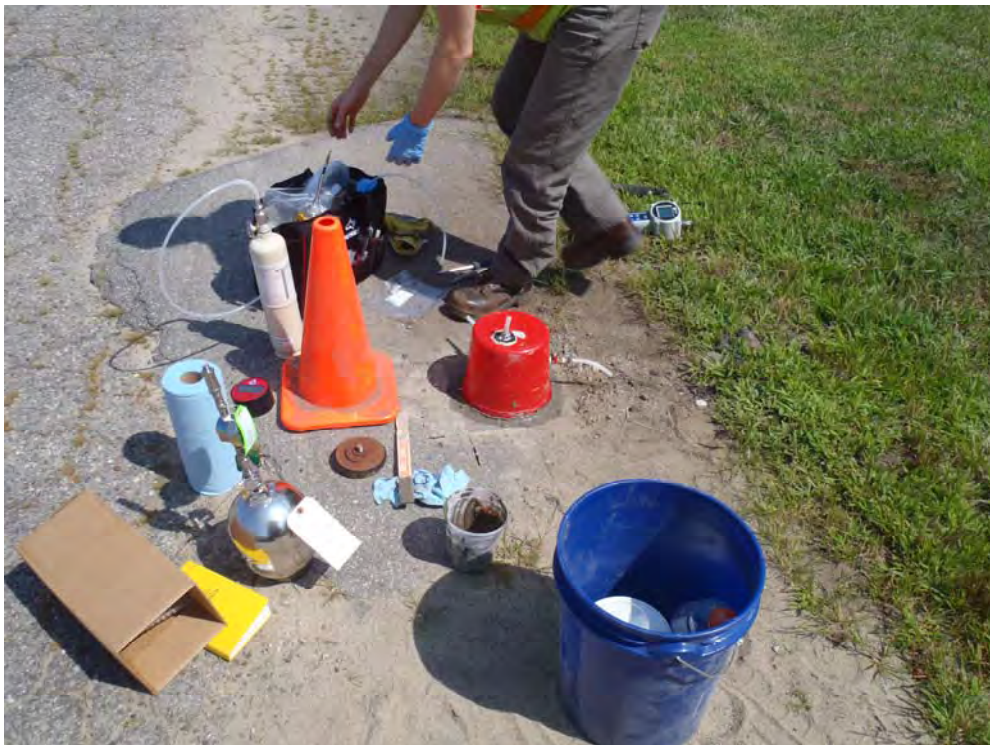
Photograph No. 35 Setup on SVP-3S for leak testing with helium tracer prior to sampling.
