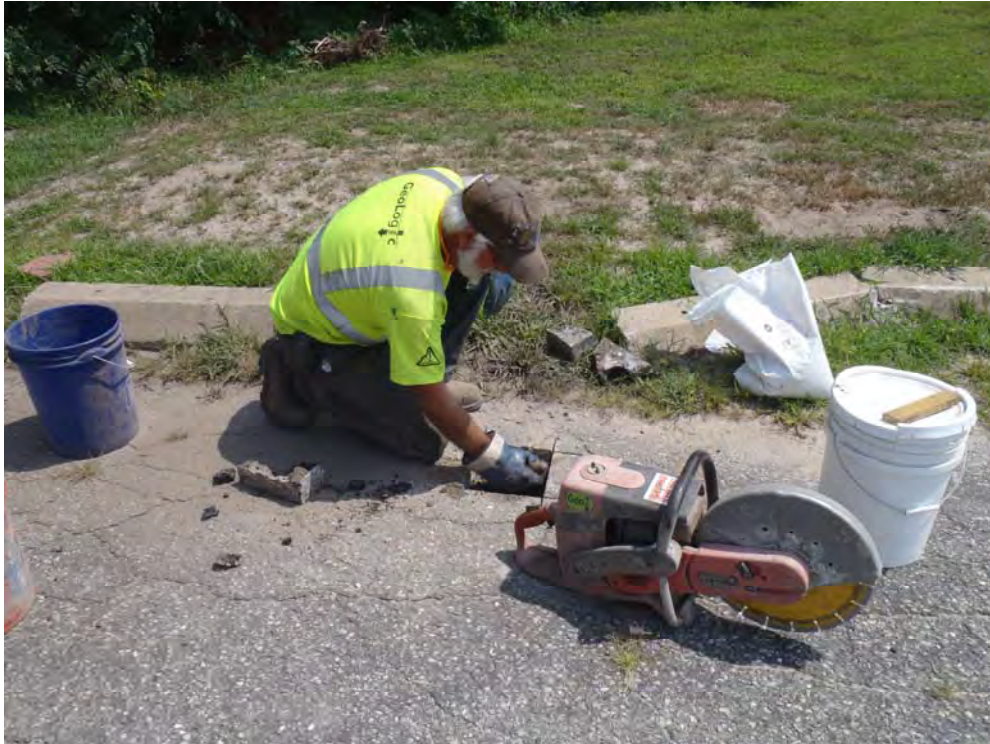
Photograph No. 34 Installation of a concrete pad and protective roadbox on SVP-2S.
