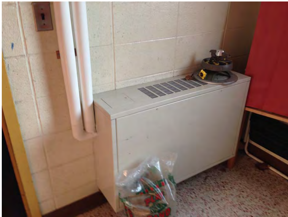
Photograph No. 16 Heat provided by natural gas fired forced hot water.
