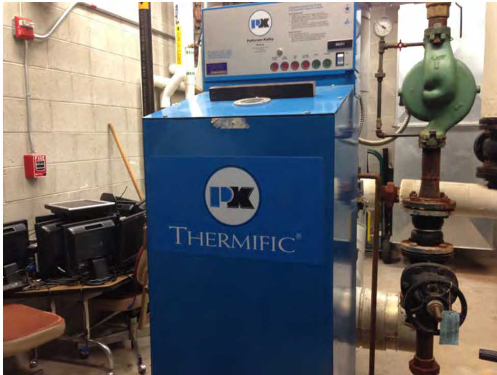
Photograph No. 21 Boiler #1 of two in the boiler room.
