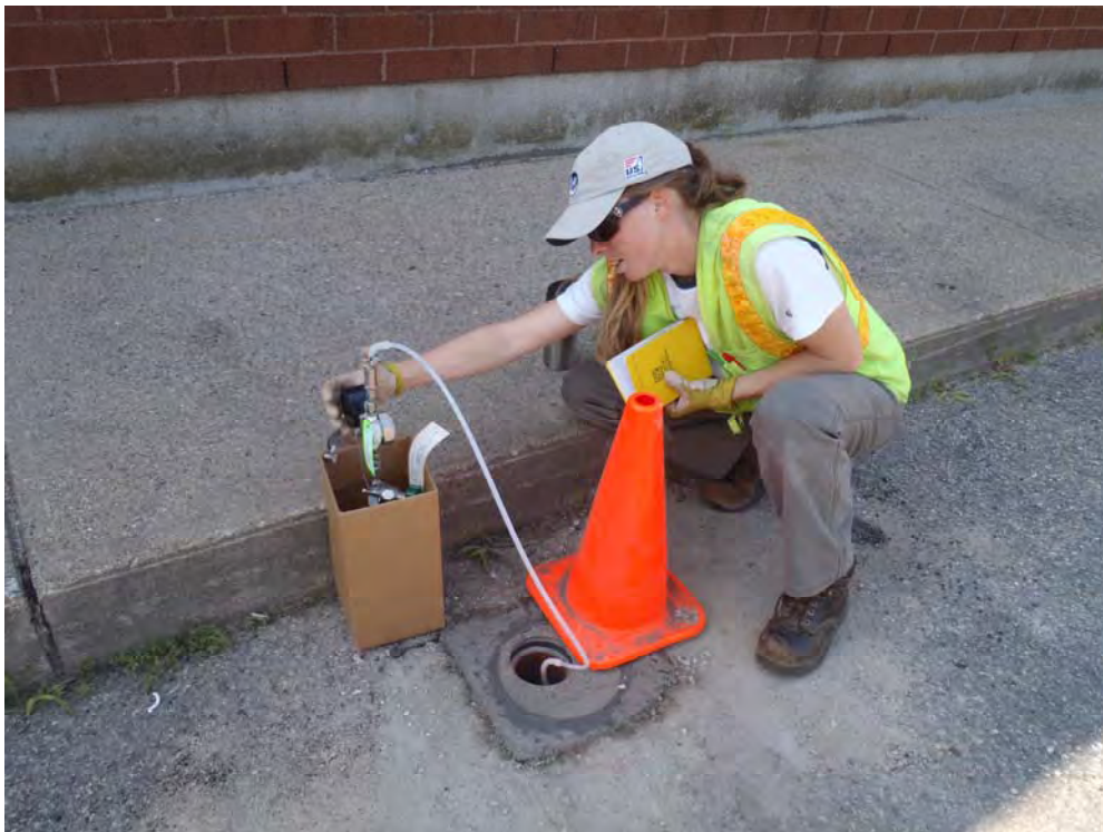
Photograph No. 37 Soil gas sample collection at SVP-1S in a 2.7L summa can with 30-minute regulator.
