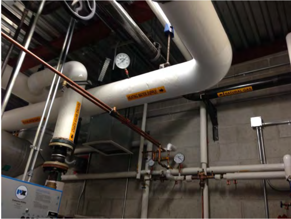
Photograph No. 22 Hot water and natural gas piping within the boiler room.
