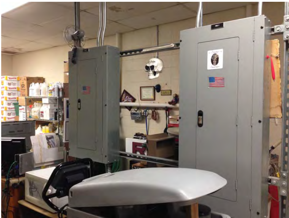
Photograph No. 20 Active circuit breakers in custodial storage area.
