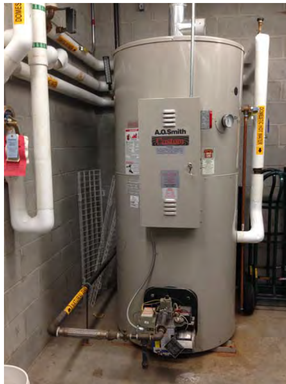
Photograph No. 21 Hot water heater in the boiler room.
