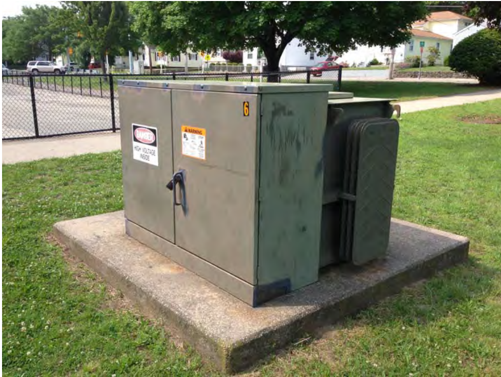
Photograph No. 3 Transformer on the west side of Varieur.
