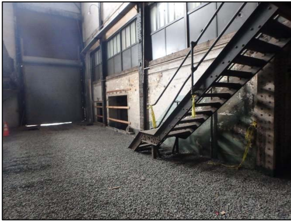
Photo 5 Overview of the turbine room on September 9, 2018, as viewed from the northwest.
