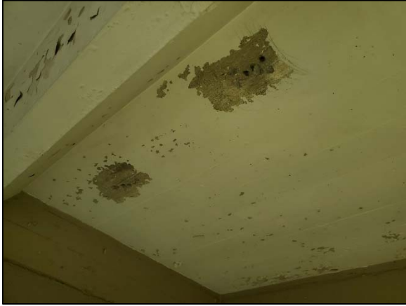
Photo 9 A view of paint and concrete ceiling samples collected from the second floor Office 1 on September 2, 2021.
