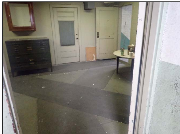
Photo 8 Overview of the second floor Office 1 room, where PCB Remediation Waste has been identified in the ceiling paint and concrete as well as the rubber floor matting, on April 29, 2021, as viewed from the northwest.
