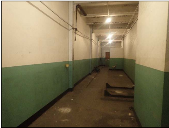
Photo 11 Overview of the third floor East Hallway, comprising PCB Remediation Waste, on April 29, 2021, as viewed from the north.
