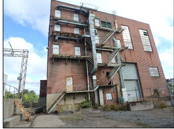
Photo 2 Overview of the south side of the Control House on September 9, 2018, as viewed from the south.
