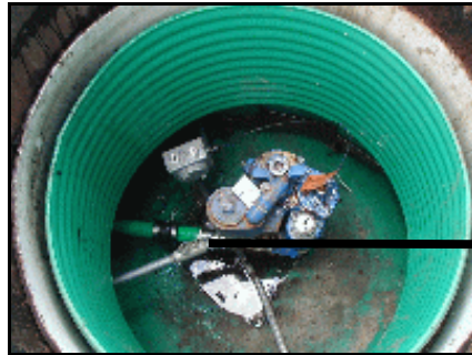
Sample Flexible Piping in a Sump
