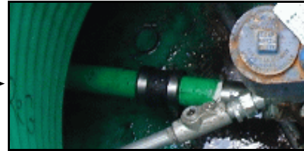
Closeup of Flexible Piping in a Sump
