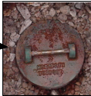
Closeup of Extractor Port
