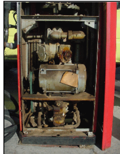
Example of a Suction Pump Inside a Dispenser
