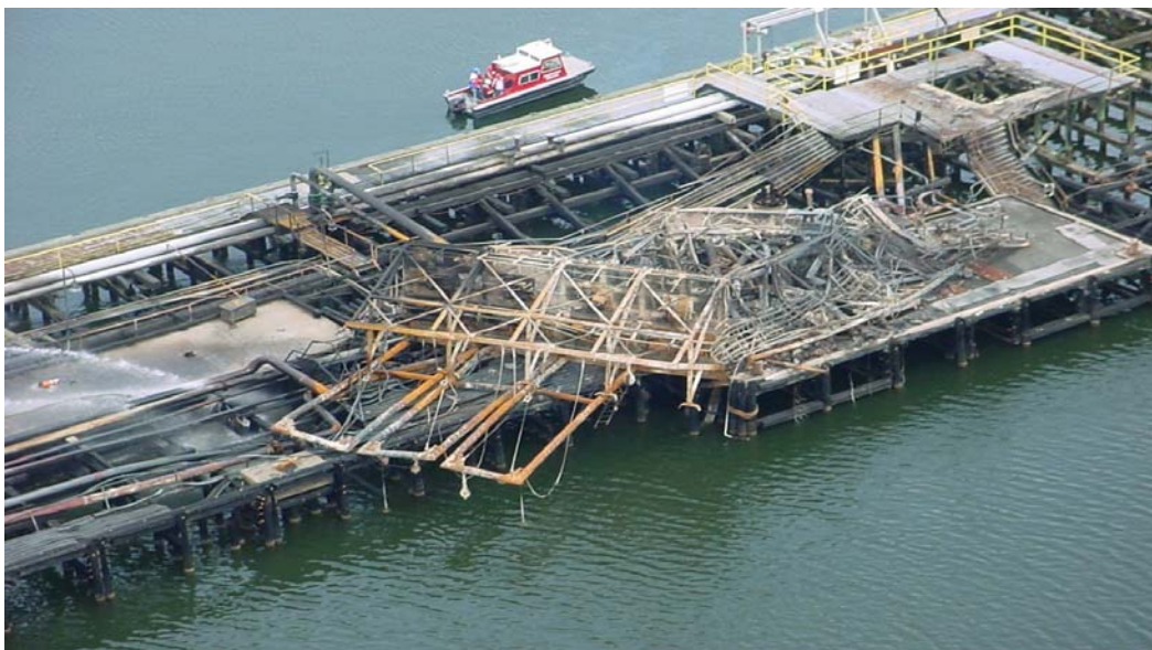
Figure 12. Aerial view of damage to Motiva dock.
