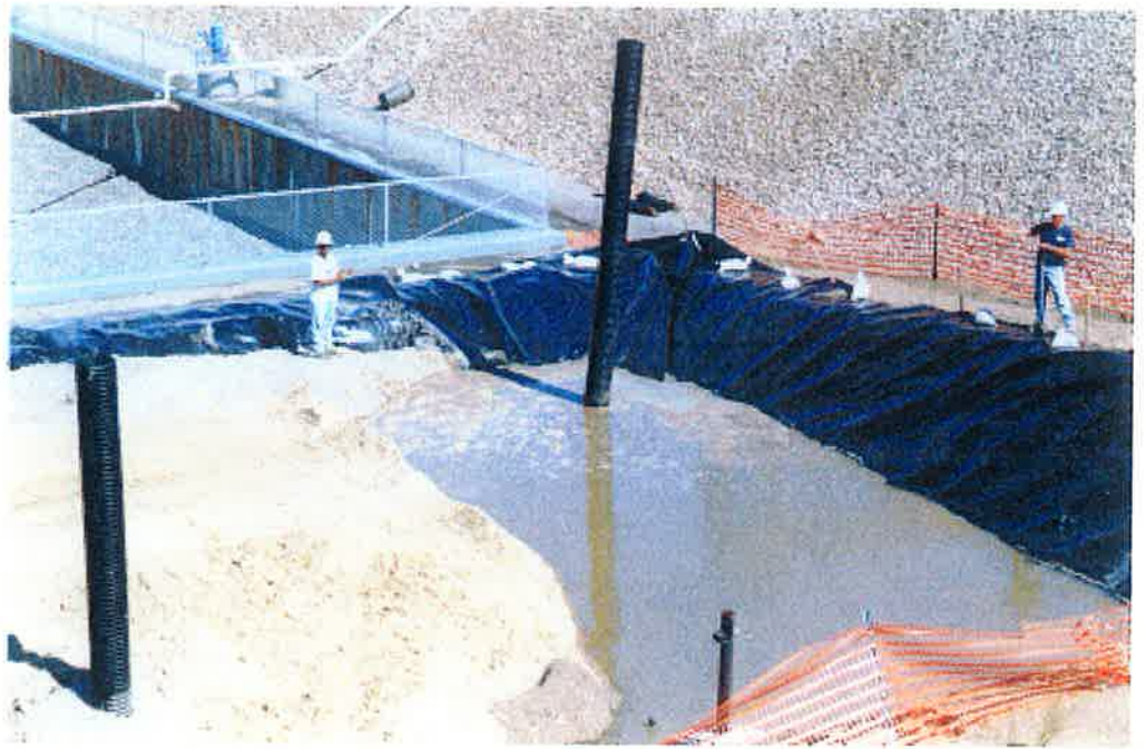
Backfill operations and installation of recovery wells in SALNG Area within dike.
