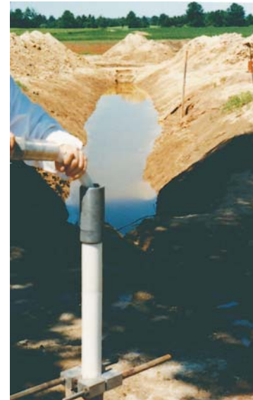
Underground oil pipeline leak assessment. Three 150 ft. (45m) installations. Two point rising head permeability tests were conducted in each interval of the Multilevel System. (See diagram showing contaminant distribution at left.)
