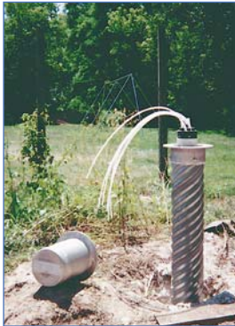
Waterloo Systems comprised entirely of stainless steel casing, packers and ports with Teflon-lined tubing were used to monitor contaminant flow in this bedrock application.
