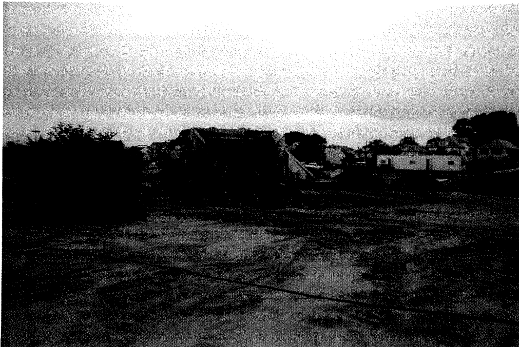
PHOTO 9 - General photo of concrete, wood and metal debris screened out of existing material
