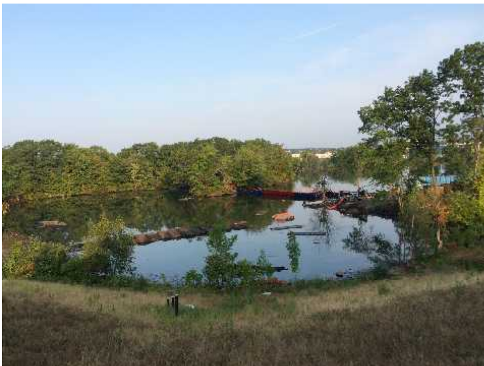
Photo 14 Second Inner Cove dewatering following dam breach
