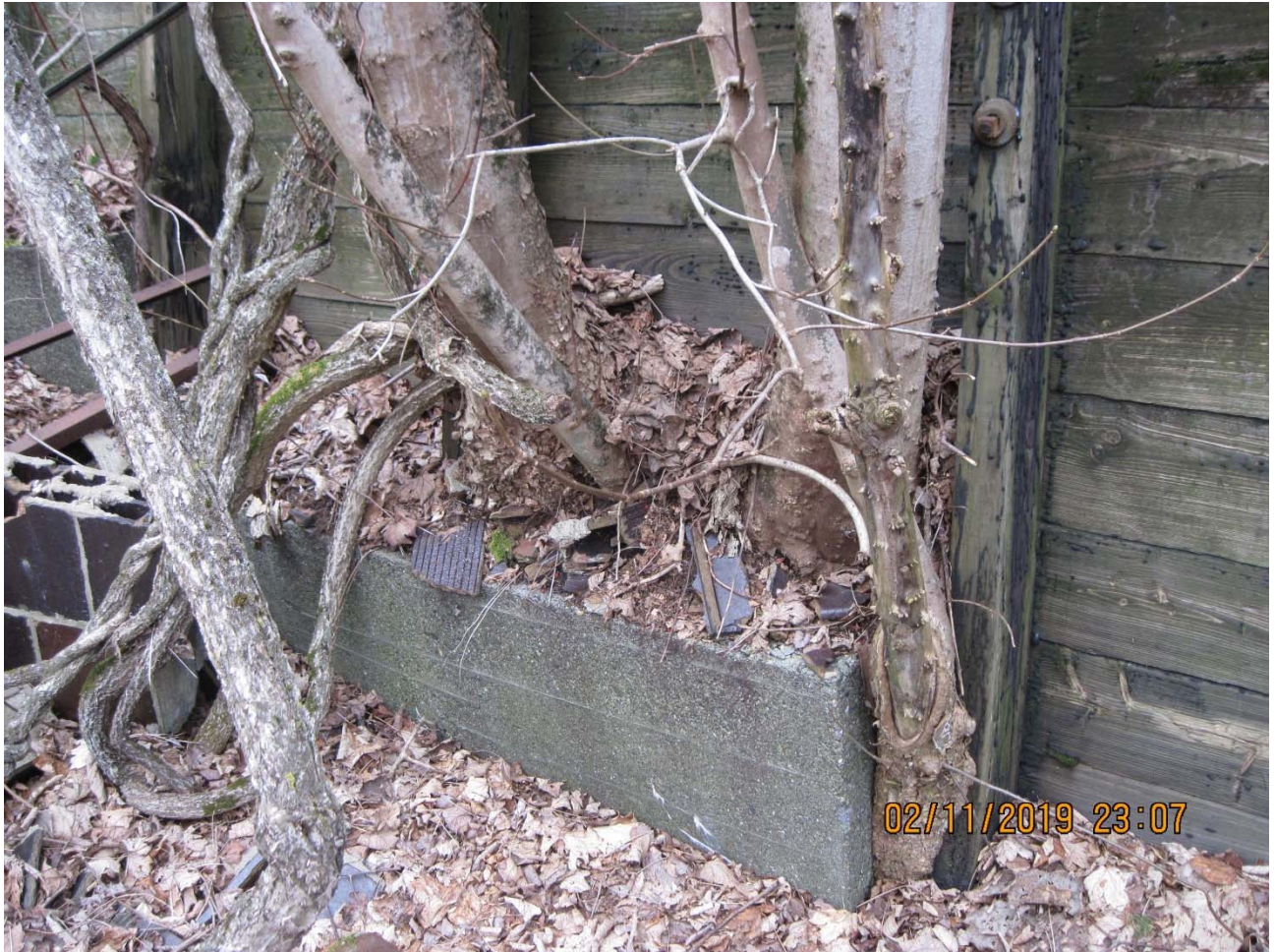
Photo #5: Vegetation Growing within Wall
