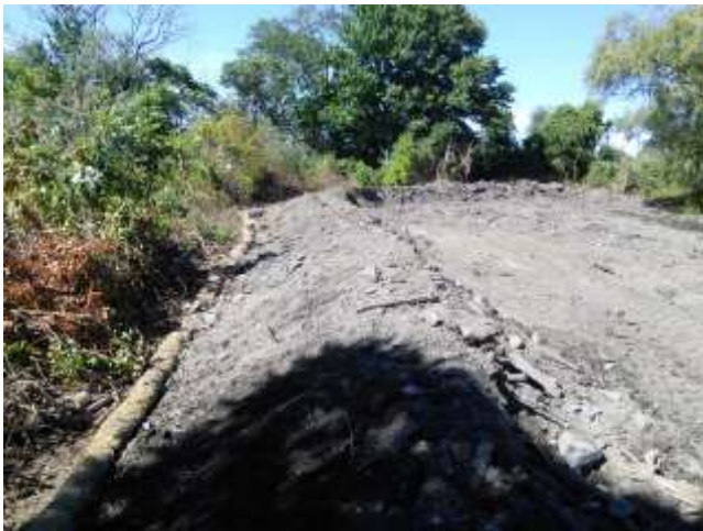
Photo 2: Looking north near property boundary showing bermed area and sedimentation controls (to left)
