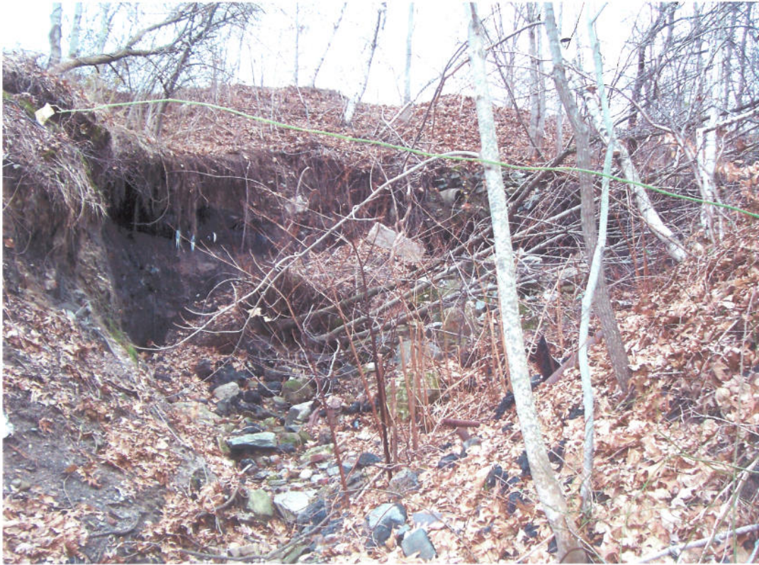
Photo 3 View looking southwest of washout area from bottom of riverbank.
