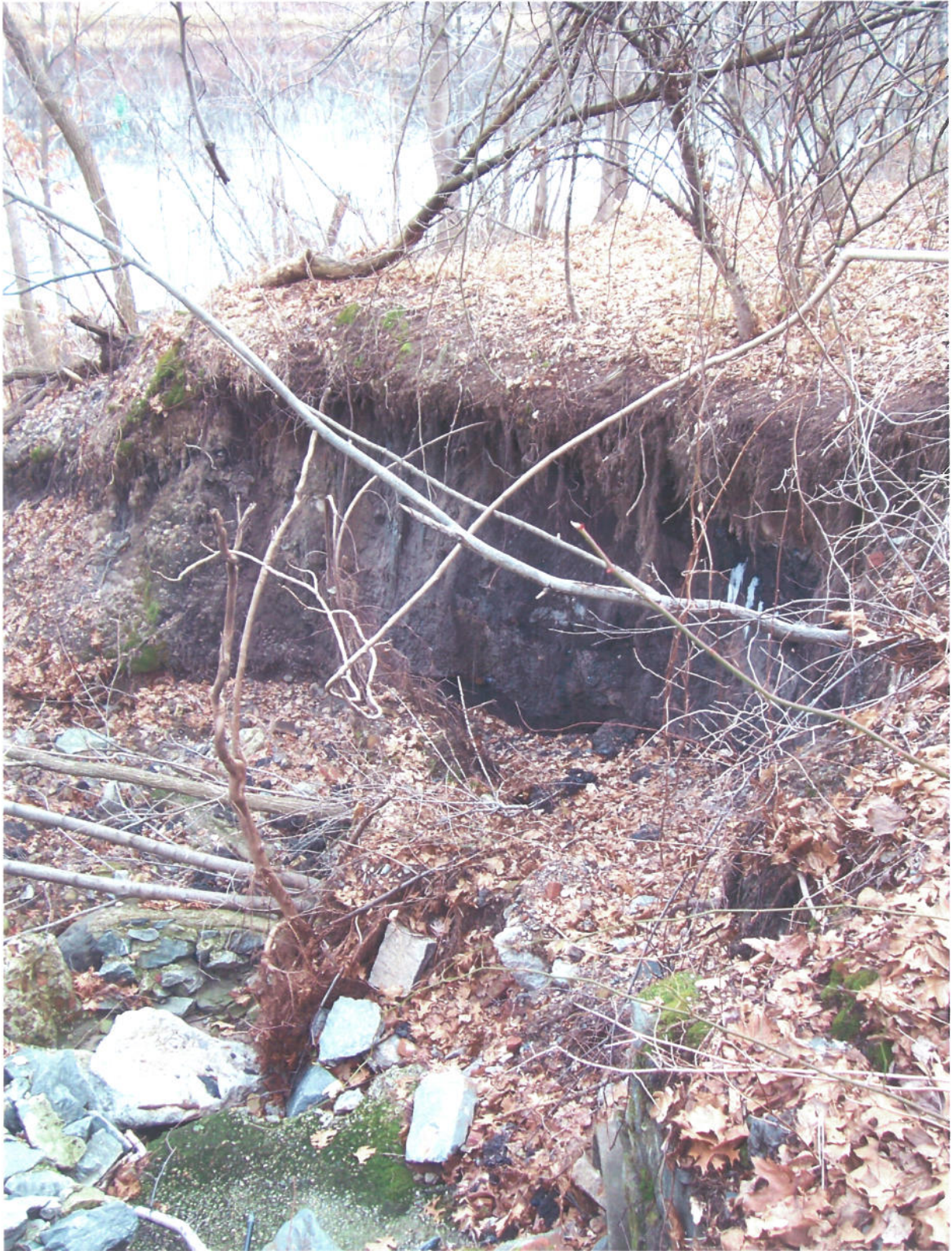
Photo 2 View of southern sidewall of South Washout Area.
