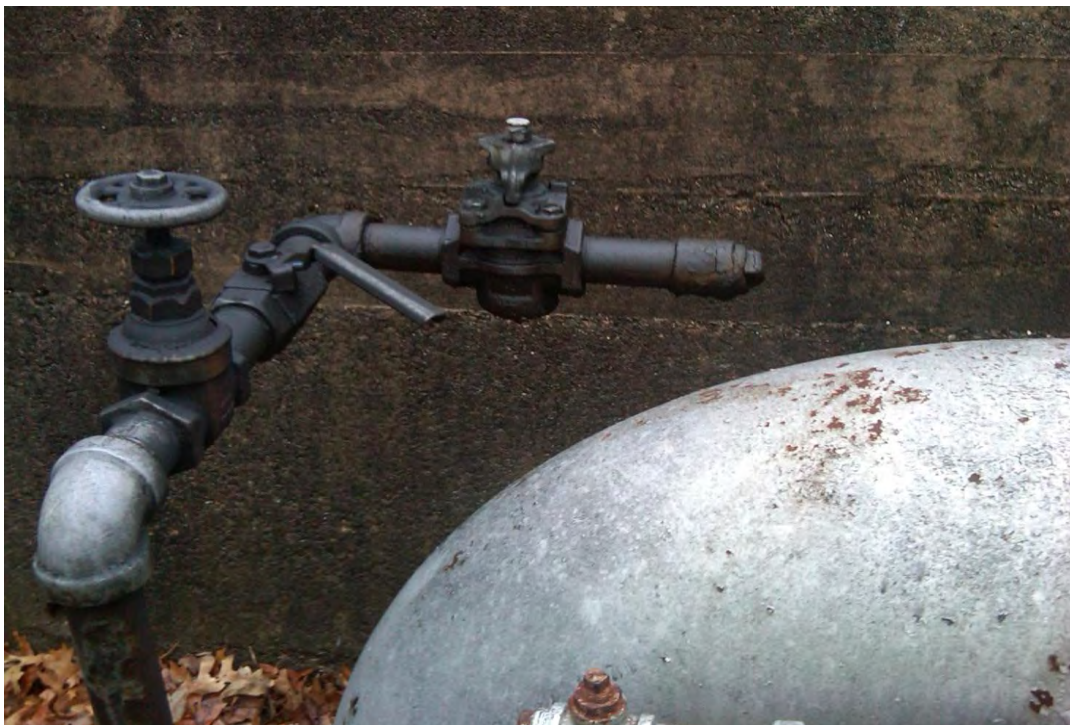
Photo 2: Photograph of metal riser pipe/valve assembly.
