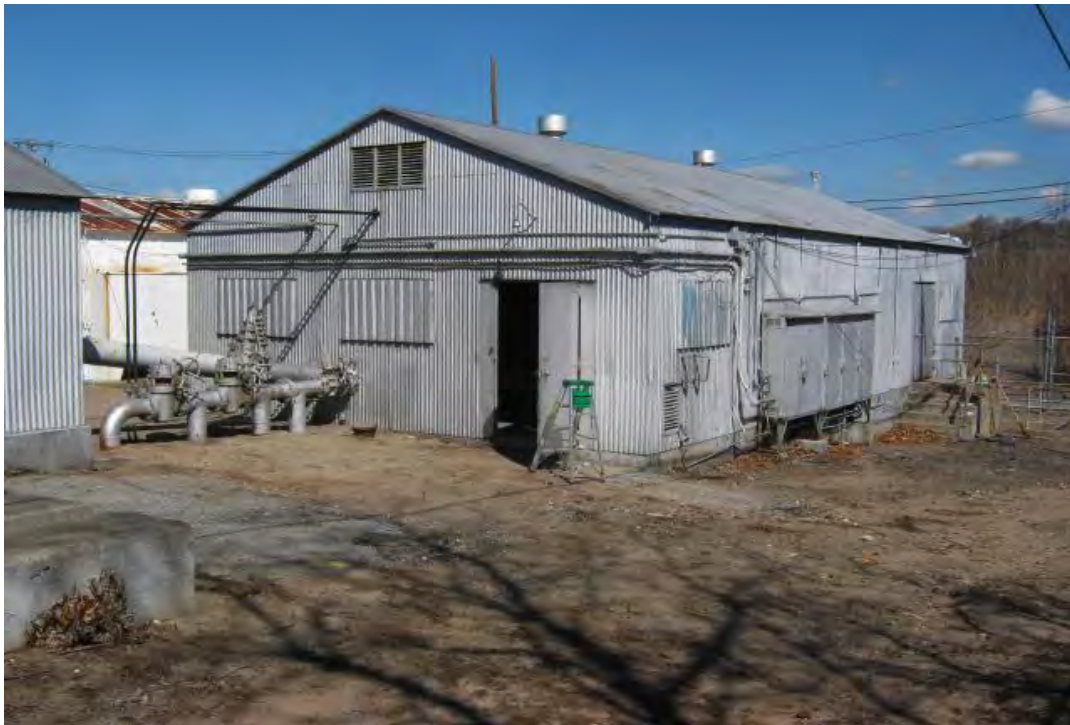
Photo 6: Photograph of natural gas regulator buildings looking south.
