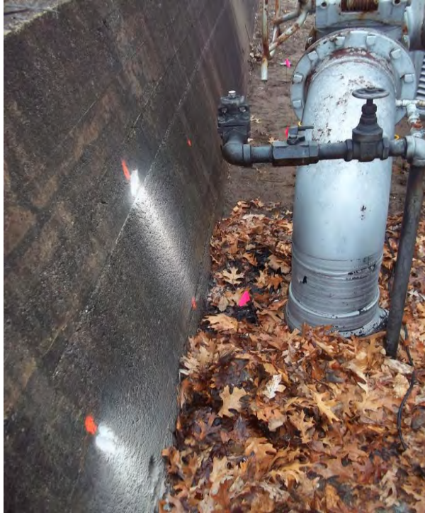
Photo 5: View looking north of retaining wall sampling proximate to metal riser pipe/valve assembly. Concrete samples (RW-1 to RW-4)
