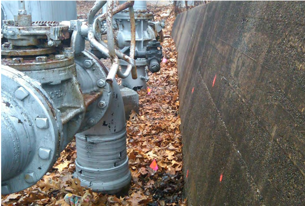
Photo 1: View looking towards south along retaining wall with metal riser pipe/valve assembly in foreground. Area of surface soil staining along base of retaining wall (area of disturbed leaf litter adjacent to riser). Soil samples (RB-E/SOIL-01 and GRSP-01)
