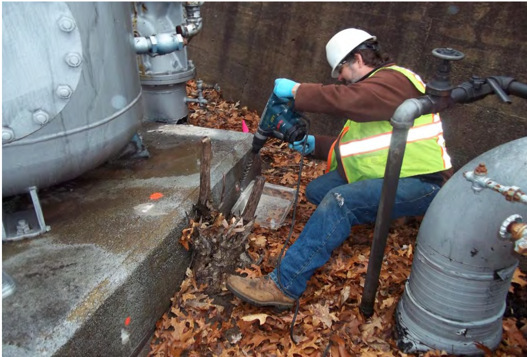
Photo 3: View of GZA personnel sampling the concrete pad proximate to metal riser pipe/valve assembly. Note the discoloration/staining present on the concrete pad. Concrete sample (CS-3)
