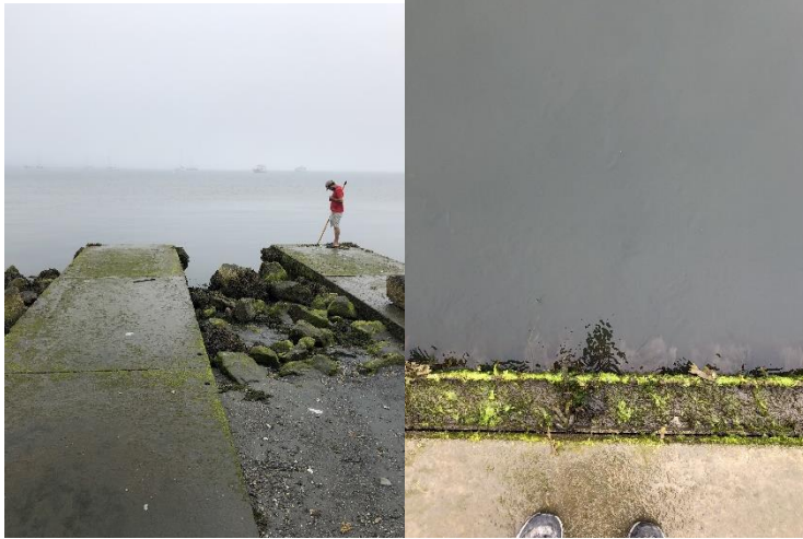
Figure 4: Source 4-550 view looking to receiving waters (left photo) downward view of exit of pipe (right photo).
