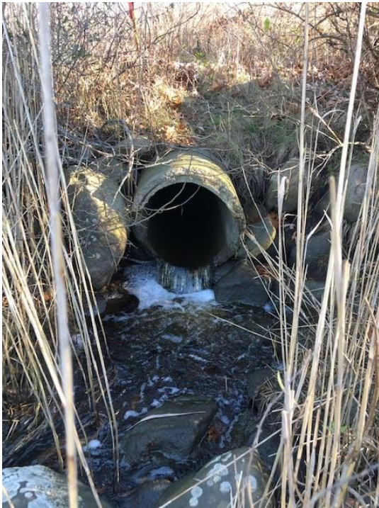
Figure 4: Source 10-200, a small stream flowing through a culvert at Kenyon Farm, Narragansett, RI.
