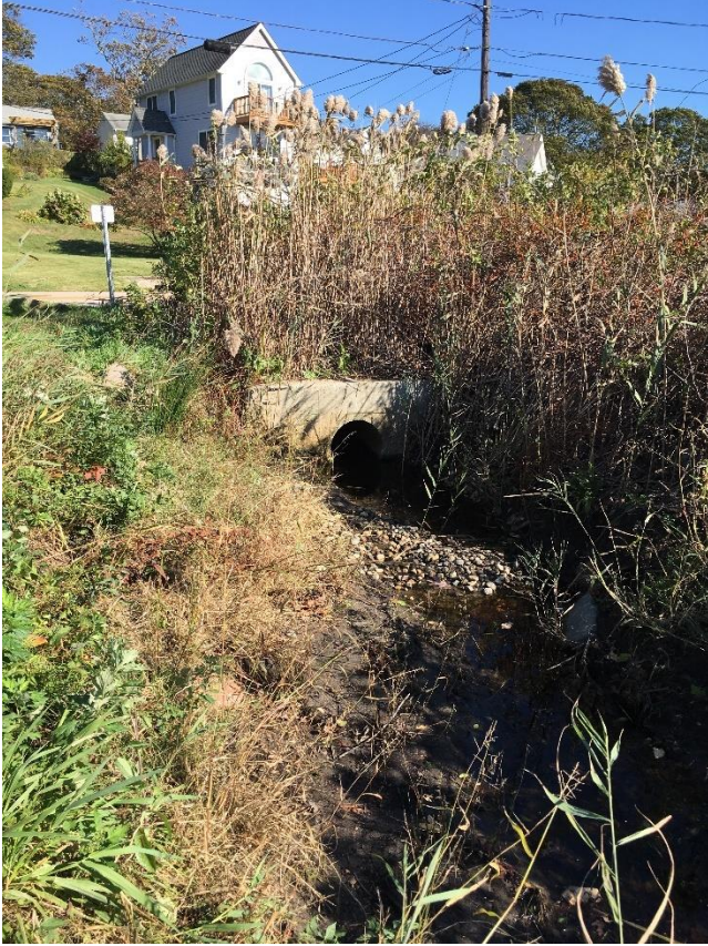
Figure 5: Source 10-11, a reinforced concrete pipe on Harbor Island, Narragansett, RI.
