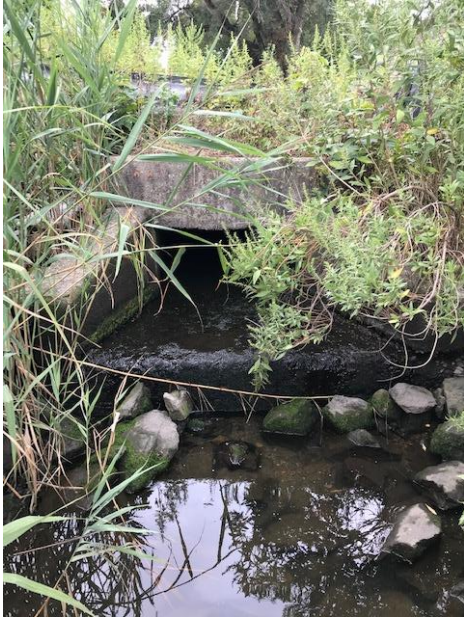
Figure 6: Source 2020-5-008, drainpipes at the extension of Parker Avenue, Warren, RI.
