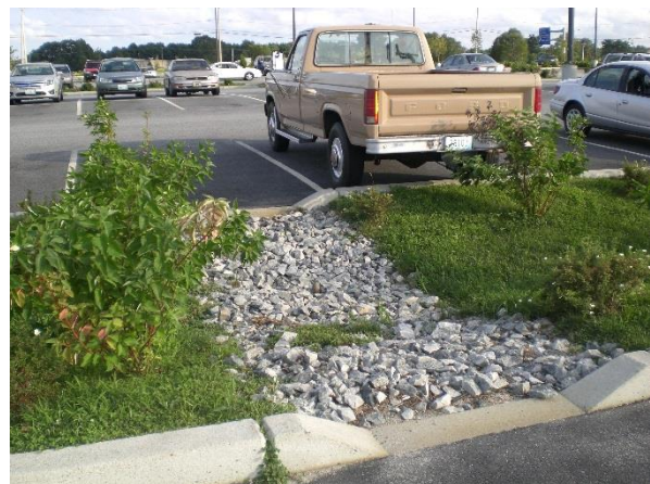
Bio-infiltration swale at a commercial parking lot in North Kingston. The curb cut allows stormwater to enter the system.
