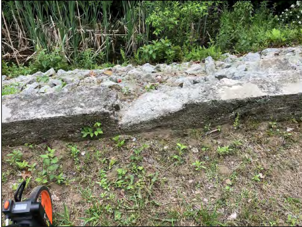
Photo No. 57: Spillway Section – Spalled and cracked concrete near STA 9+00.
