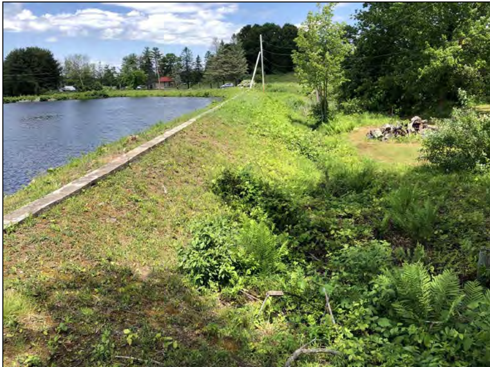
Photo No. 52: Pine Ledge Road to West Greenville Road Dam – Downstream slope from near STA 3+50 looking left.
