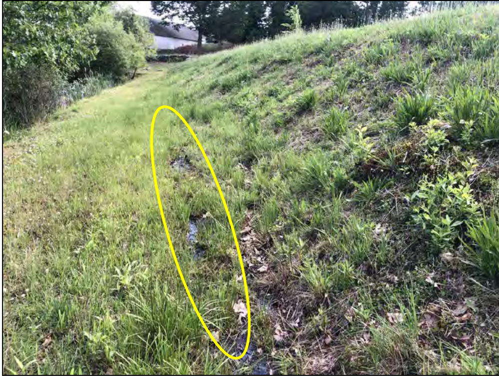
Photo No. 31: Bookers Dam - Downstream embankment from near STA 2+50 looking right. Note seepage areas along the toe of the slope.
