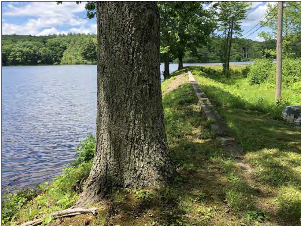
Photo No. 50: Pine Ledge Road to West Greenville Road Dam – Crest, concrete corewall, and upstream slope of the embankment right of Pine Ledge Road from near the right abutment looking left. Note the 30-inch tree located at the right abutment and the two trees in the background of the photo near STA 4+00.
