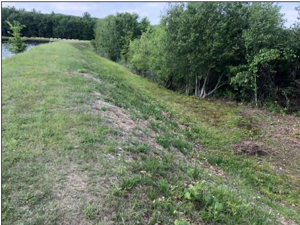
Photo No. 30: Bookers Dam - Downstream slope from near the right abutment looking left.
