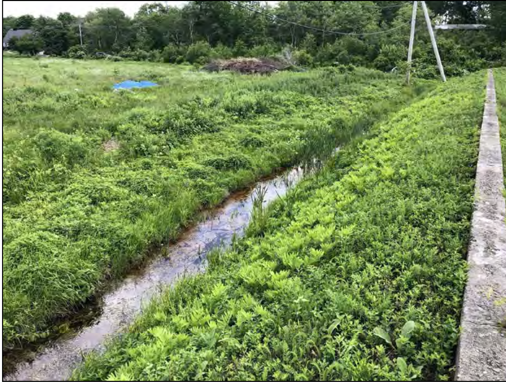
Photo No. 51: Pine Ledge Road to West Greenville Road Dam – Overview of the downstream slope from near STA 0+10 looking right. Note the orange stained seepage channel along the toe of the embankment.
