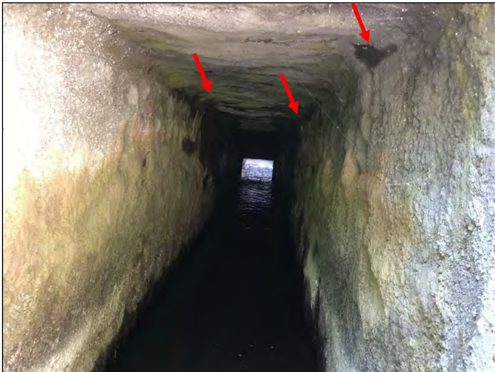
Photo No. 18: Main Dam - Interior of the outlet conduit as viewed from the downstream end looking upstream. Note the saturated wall and ceiling areas along the upstream portion of the conduit.
