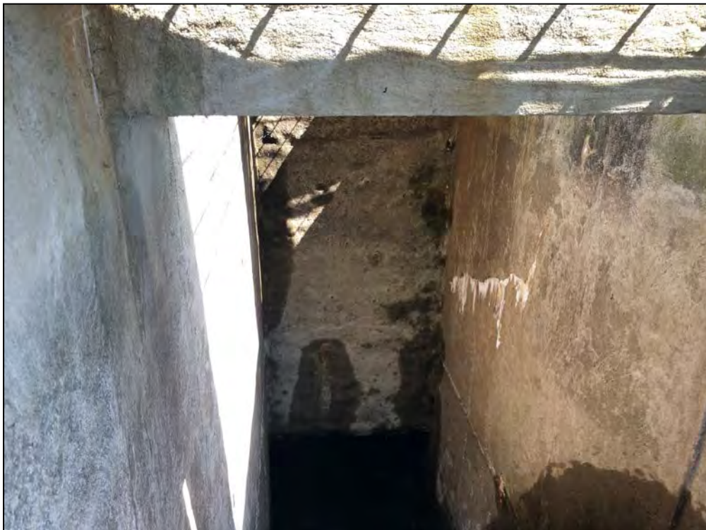
Photo No. 16: Main Dam - View of the upstream end of the outlet conduit. Note the hairline crack with efflorescence on the interior of the right wall of the intake structure and the saturated areas along the conduit upstream headwall.
