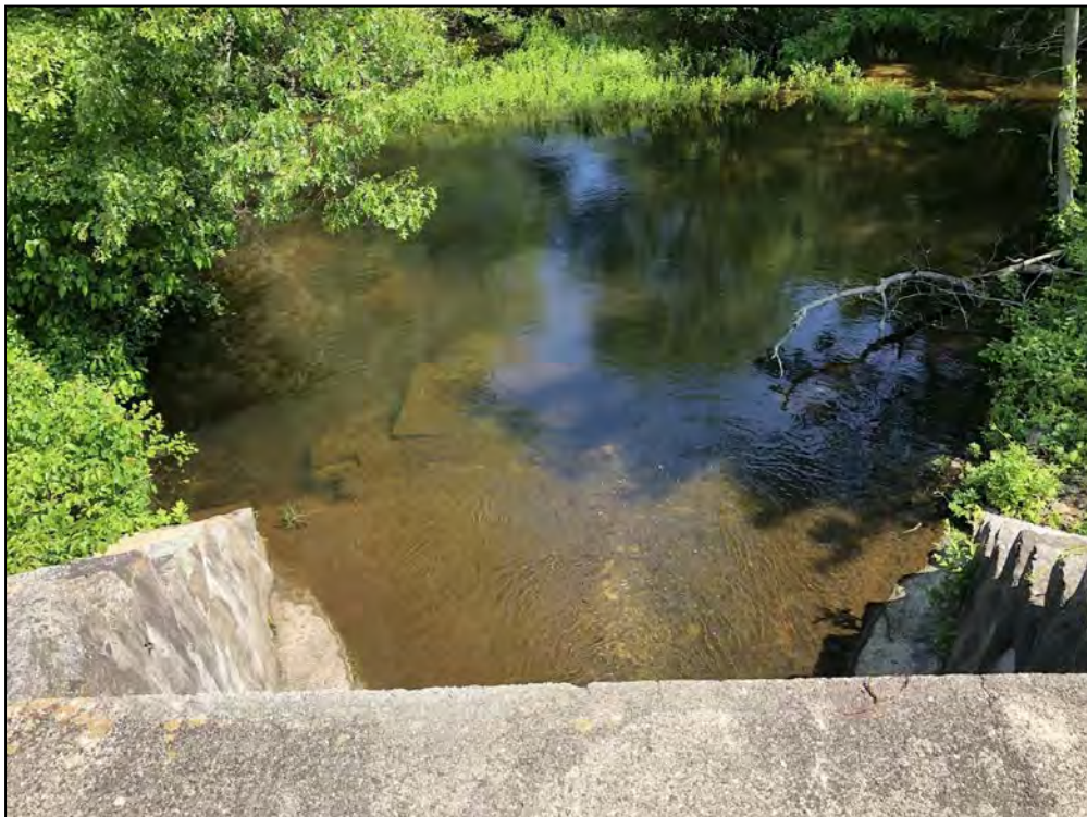
Photo No. 22: Main Dam - Overview of the downstream channel from the low-level outlet.
