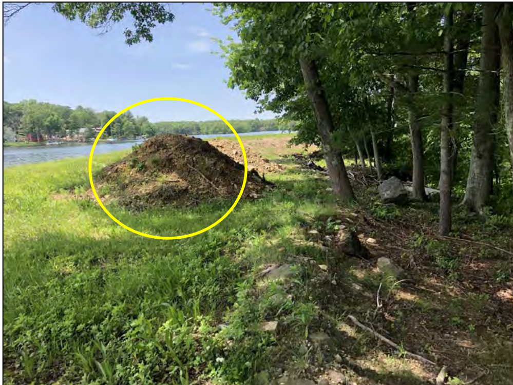
Photo No. 34: Bookers Dam - Downstream slope from near STA 9+50 looking left. Note stored material along the mid-slope.
