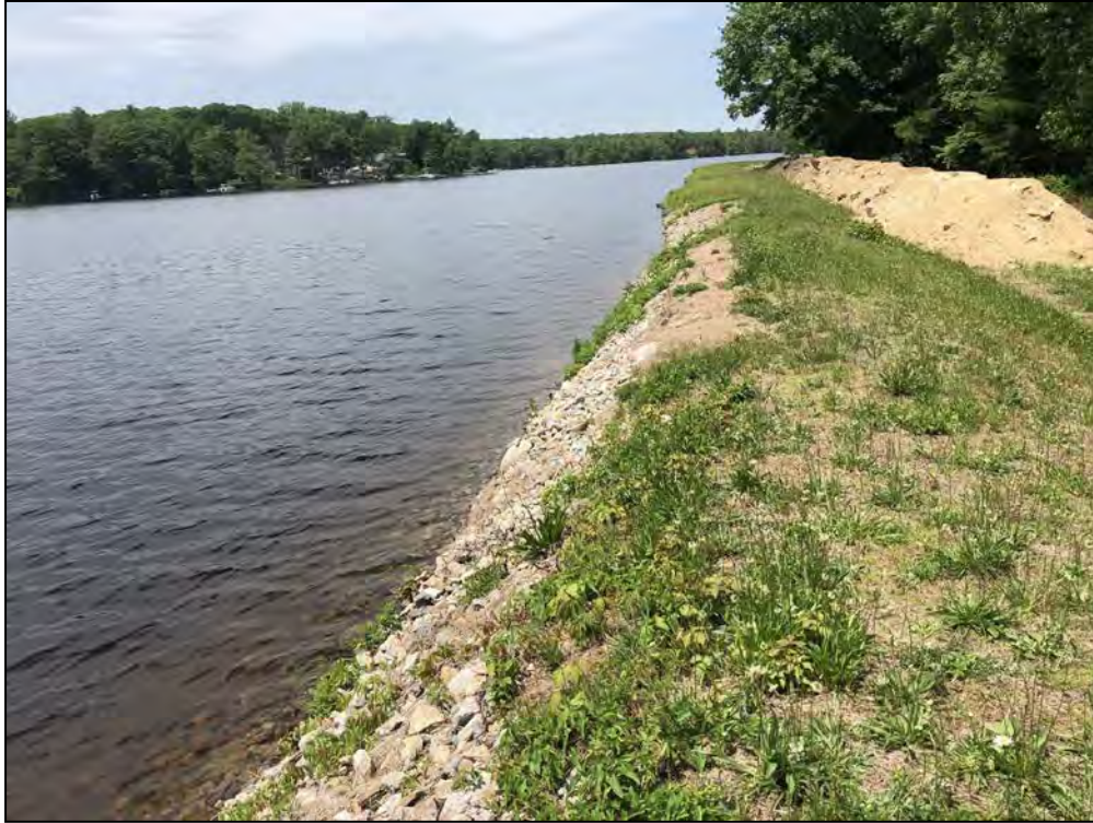
Photo No. 25: Bookers Dam - Upstream slope and crest from near STA 9+00 looking left. Note area of damaged slope and stored material along the downstream toe of the slope.
