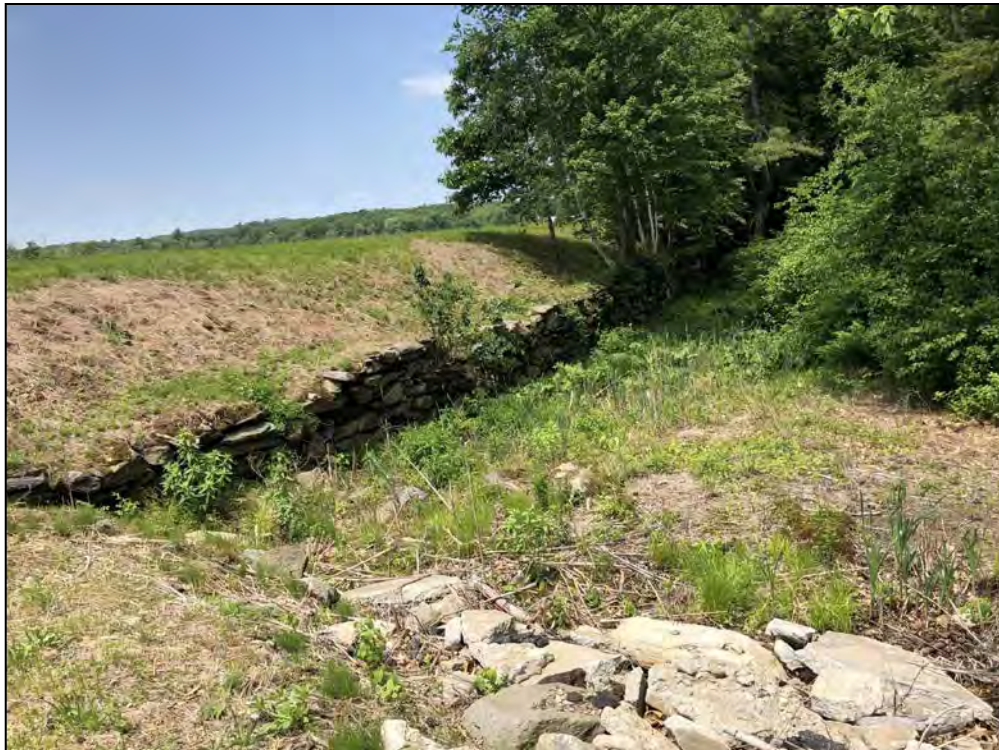
Photo No. 36: Bookers Dam - Downstream slope and stone masonry wall from STA 12+00 looking left.
