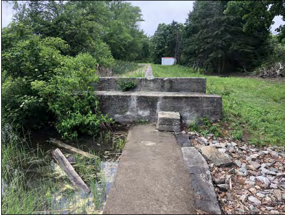
Photo No. 65 Spillway Section – View of the spillway weir and the spillway left channel wall.
