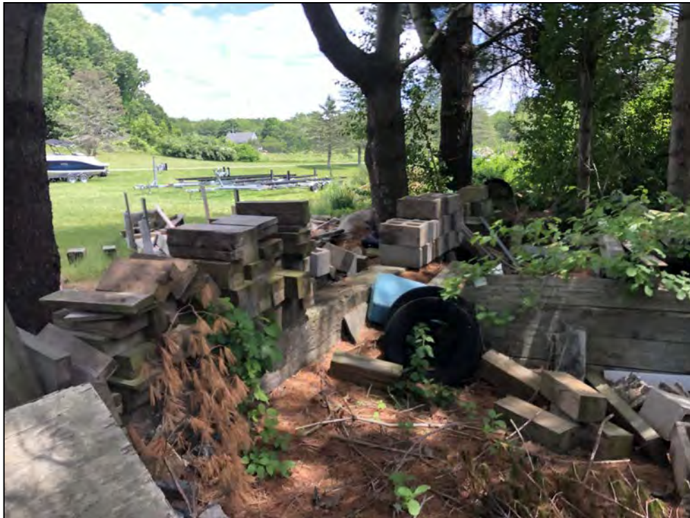
Photo No. 40: Marina Dam – Overview of the marina walls looking right towards pine ledge road. Note materials stored along and on top of the flood walls.
