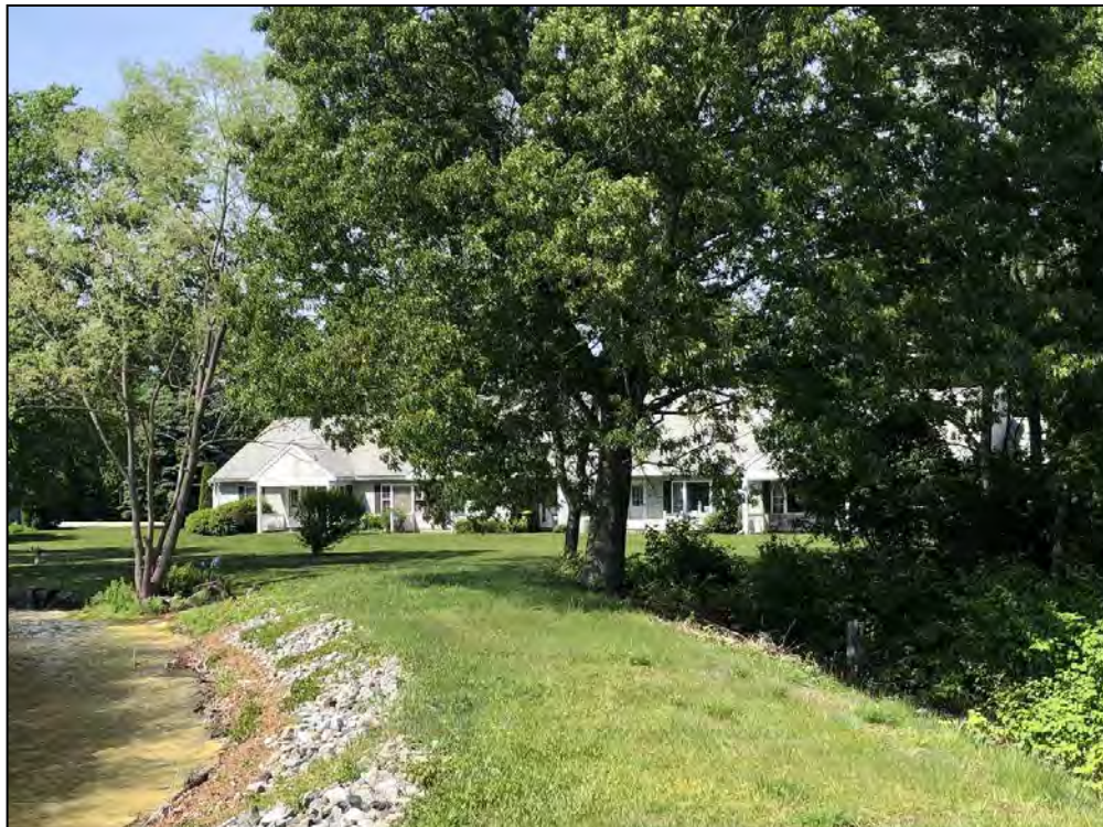
Photo No. 4: Main Dam – Crest at the left abutment. Note the 30-inch diameter tree at the downstream side of the crest. .
