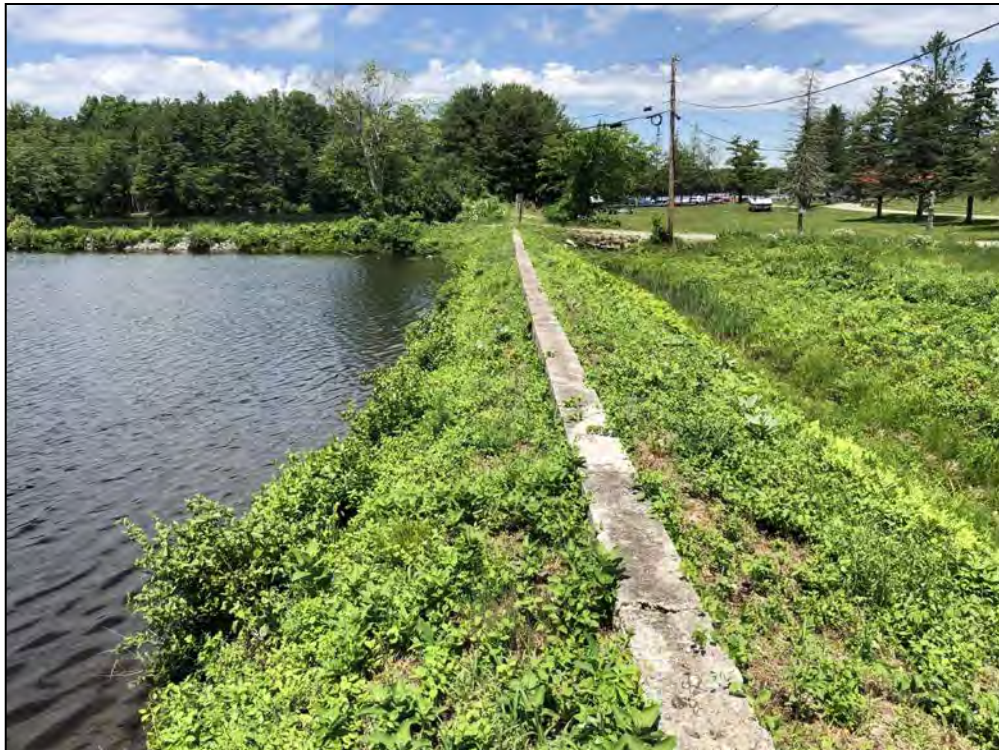
Photo No. 48: Pine Ledge Road to West Greenville Road Dam – Crest, concrete corewall, and upstream slope of the embankment right of Pine Ledge Road from near STA 1+30 looking left.
