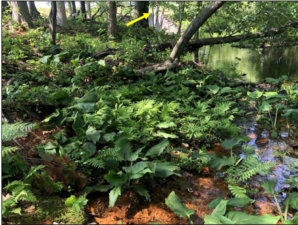
Photo No. 13: Main Dam - Seepage at the toe of the wooded slope 100 feet downstream and right of the outlet structure (arrow).
