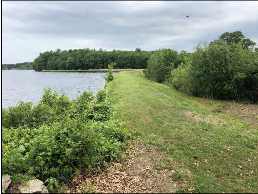
Photo No. 27: Bookers Dam - Crest from near the right abutment looking left.
