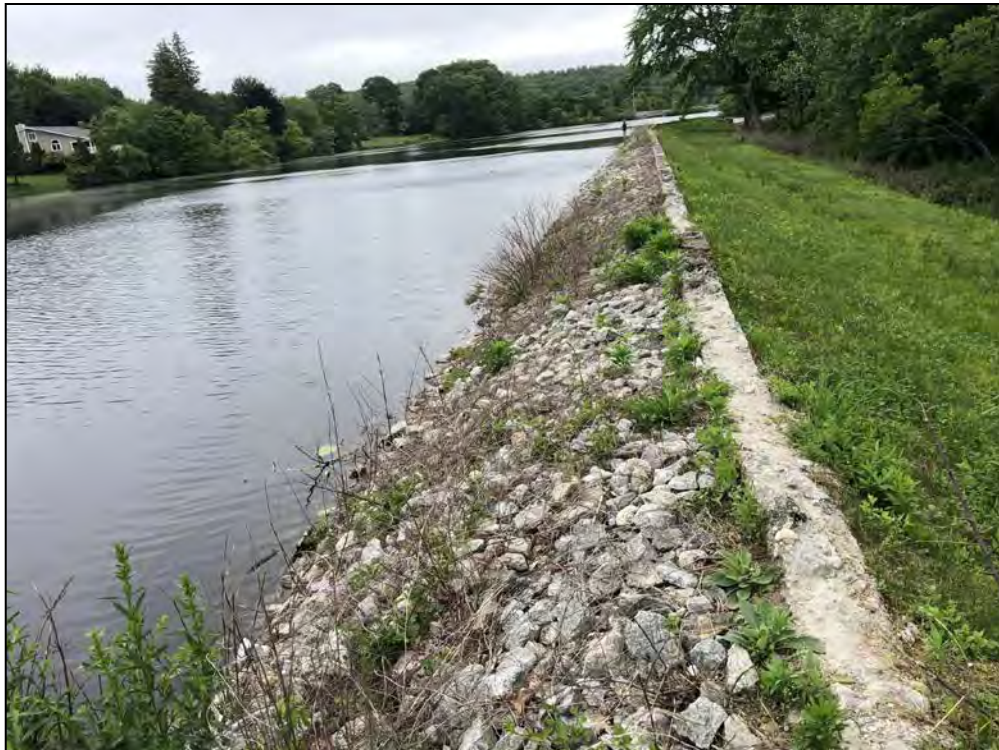
Photo No. 56: Spillway Section – Upstream slope and crest from near STA 2+50 looking left.
