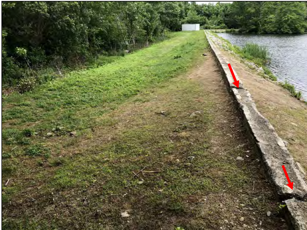
Photo No. 62: Spillway Section – Downstream slope from near the left abutment looking right. Note through cracks along the corewall.
