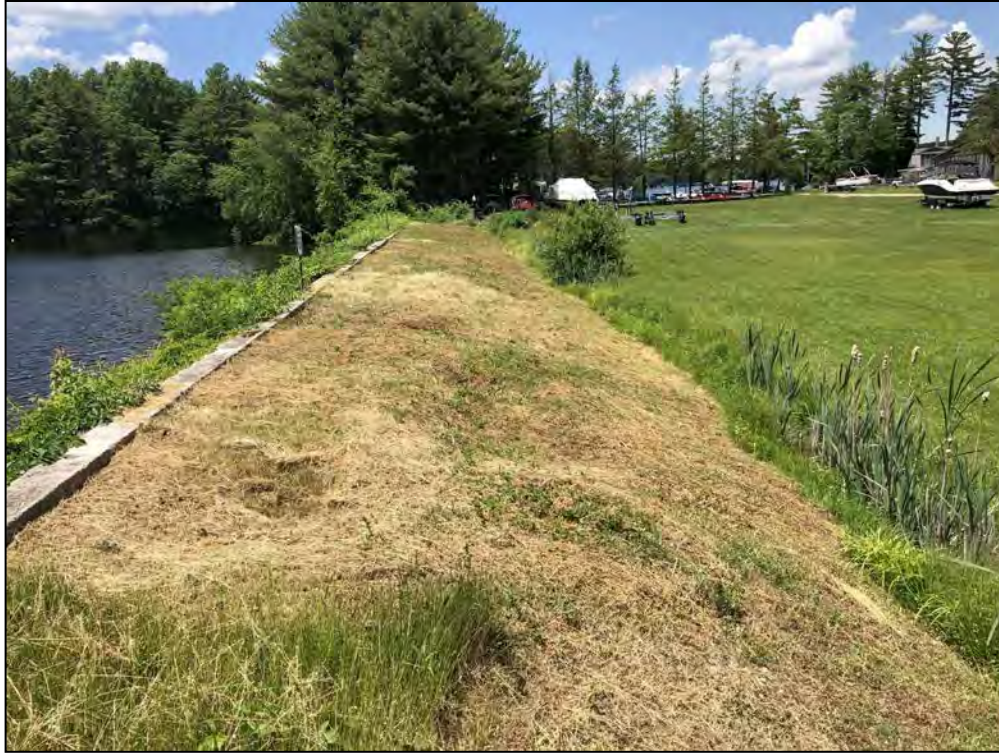
Photo No. 45: Pine Ledge Road to West Greenville Road Dam – Crest and downstream slope of the embankment left of Pine Ledge Road. Note the vertical irregularities along the downstream slope.
