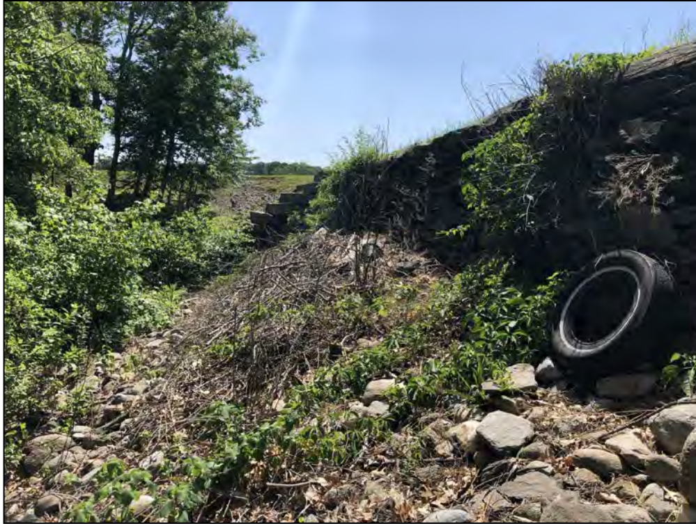
Photo No. 9: Main Dam - Area downstream of the downstream wall from near STA 1+30 looking right.
