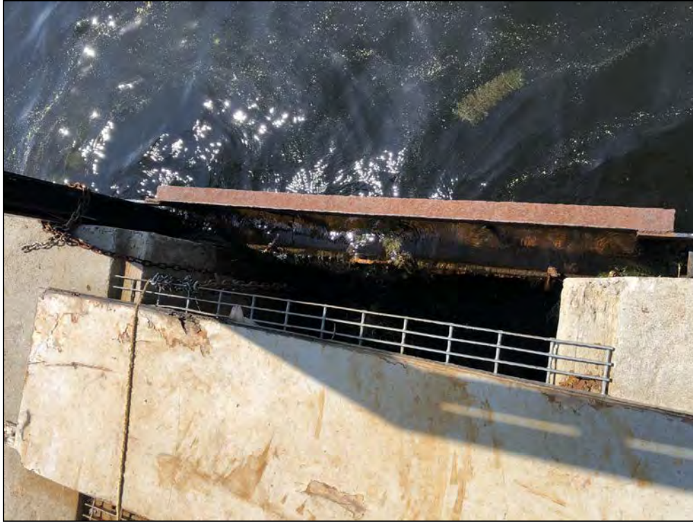
Photo No. 15: Main Dam - Upstream end of the intake to the outlet structure.
