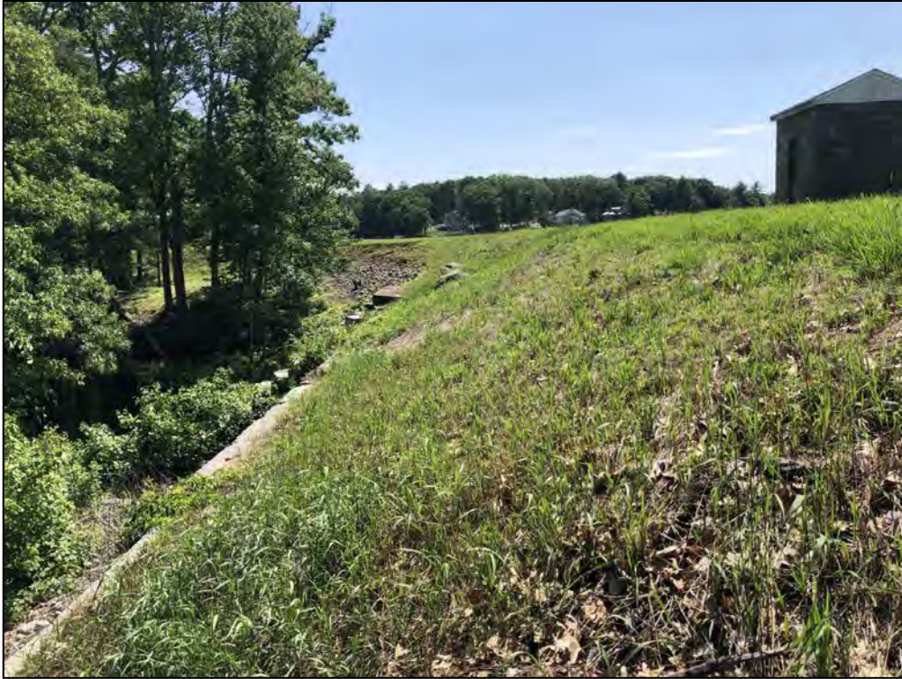
Photo No. 7: Main Dam - Downstream side of the crest from left of the low-level outlet looking right.
