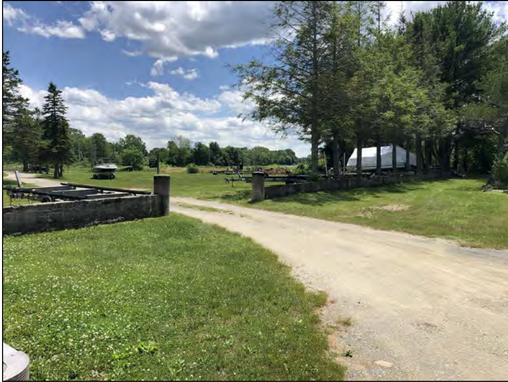
Photo No. 41: Marina Dam – View of the floodwalls at the Marina from the upstream side looking downstream. Note the area of the access road through the floodwalls is lower than the floodwalls.
