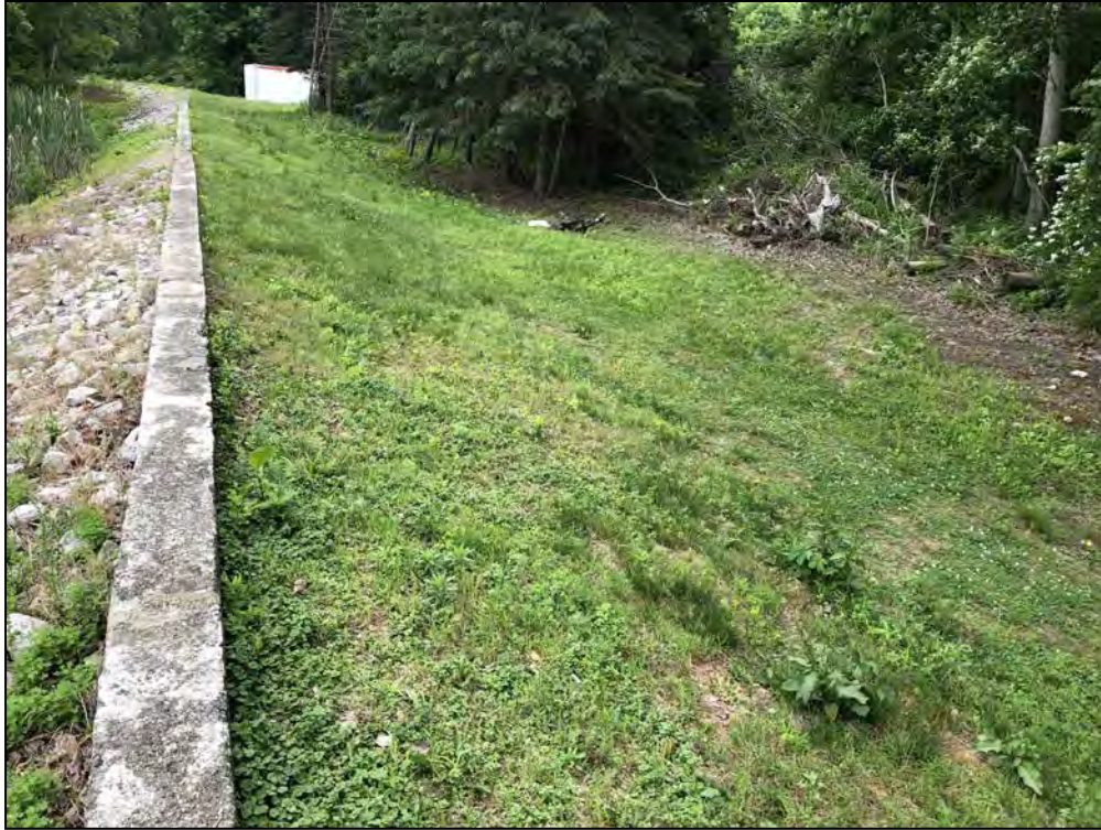
Photo No. 61 Spillway Section - Downstream slope from left of the spillway looking left.
