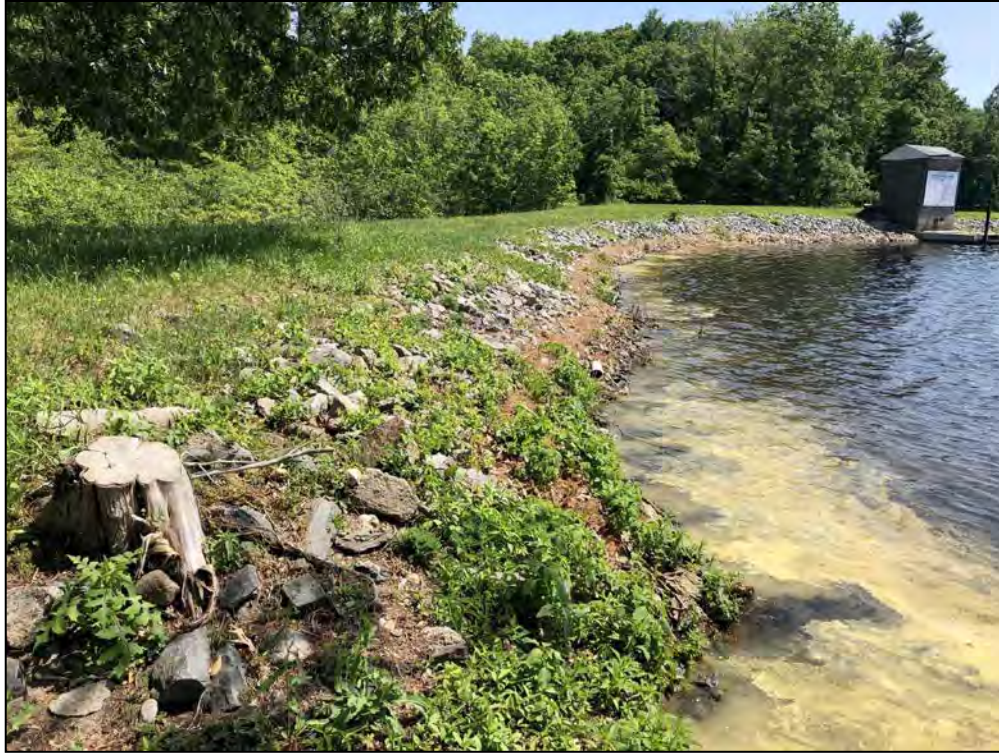
Photo No. 1: Main Dam - Upstream side of the dam from near the left abutment looking right.
