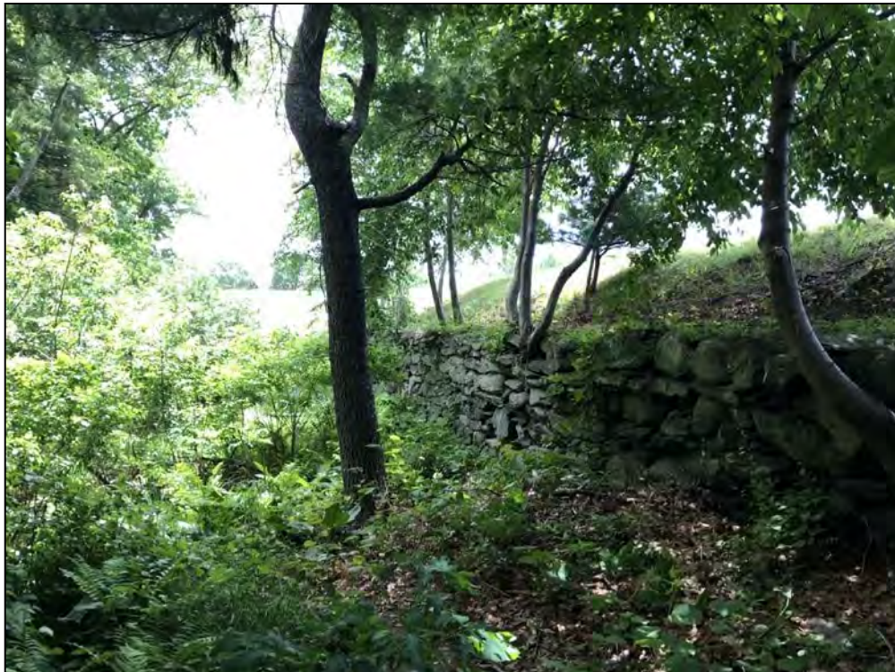
Photo No. 38: Bookers Dam - Downstream stone masonry wall viewed from near the left abutment looking right.
