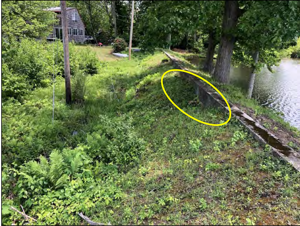
Photo No. 53: Pine Ledge Road to West Greenville Road Dam – Overview of the downstream slope from near STA 3+75 looking right. Note the eroded area of the downstream slope near STA 4+00 exposing the corewall.
