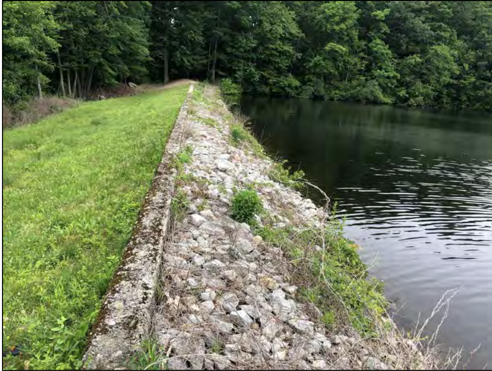
Photo No. 55: Spillway Section – Upstream slope and crest from near STA 2+50 looking right.
