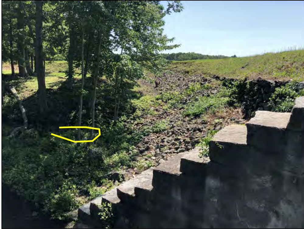
Photo No. 11: Main Dam - Downstream side of the embankment right of the outlet structure. Note the location of the previously reported seepage.
