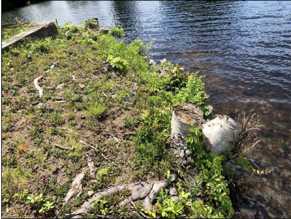
Photo No. 49: Pine Ledge Road to West Greenville Road Dam – Tree stumps along the upstream slope near STA 3+25.
