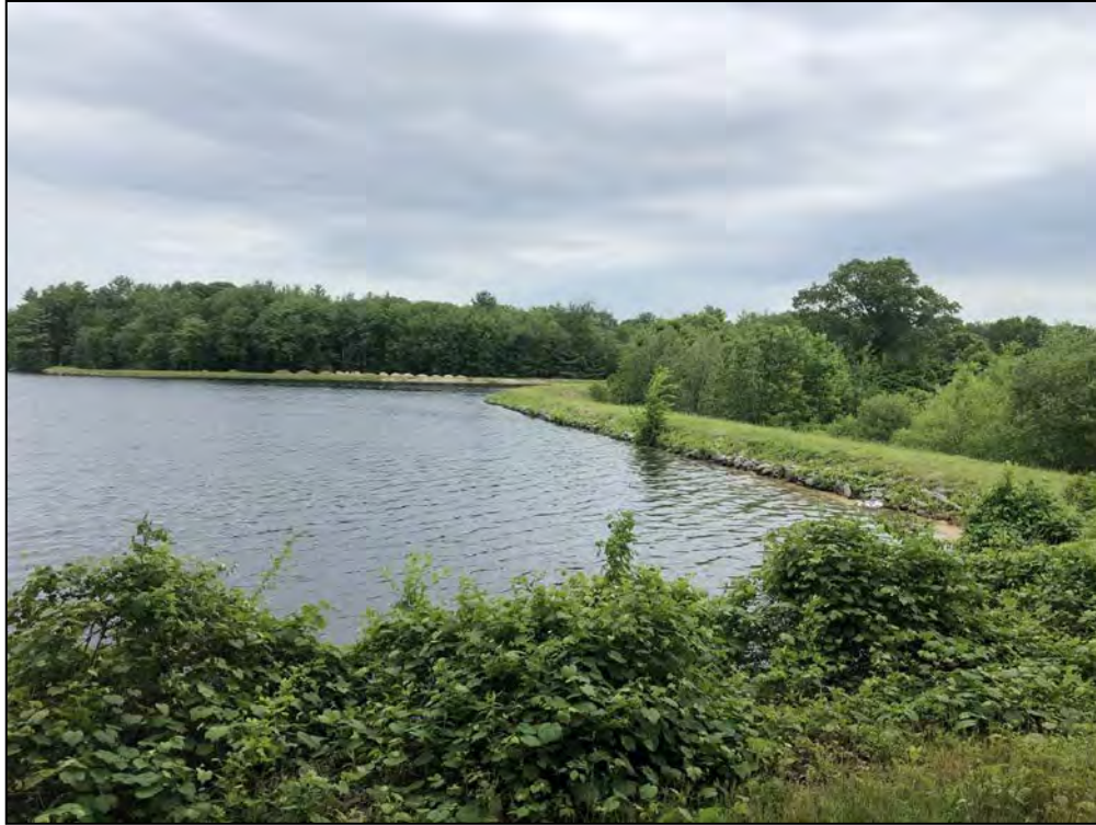
Photo No. 23: Bookers Dam - Overview of the upstream side of the dam from the right abutment looking left.
