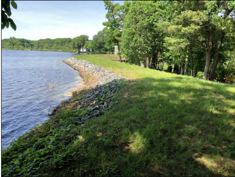
Photo No. 3: Main Dam - Upstream slope from the right abutment looking left.
