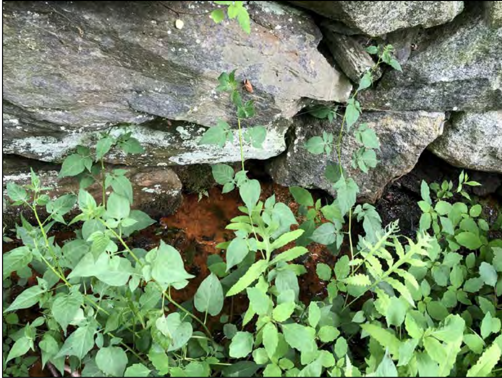
Photo No. 37: Bookers Dam – Seepage along the base of the downstream stone masonry wall near STA 13+25.
