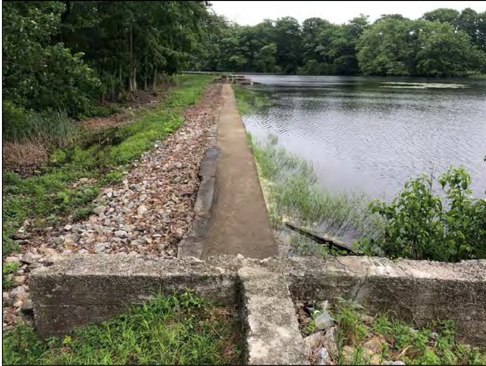
Photo No. 63 Spillway Section – Crest of the spillway section from the spillway left channel wall looking right.
