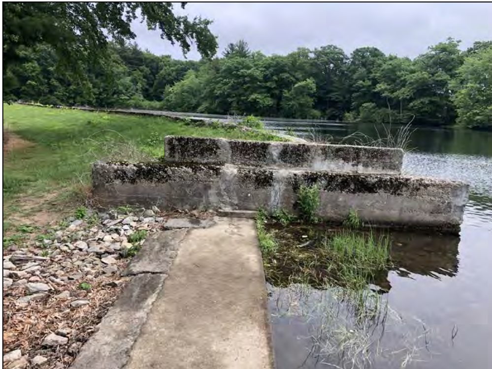
Photo No. 64: Spillway Section – View of the spillway weir and the spillway right channel wall.
