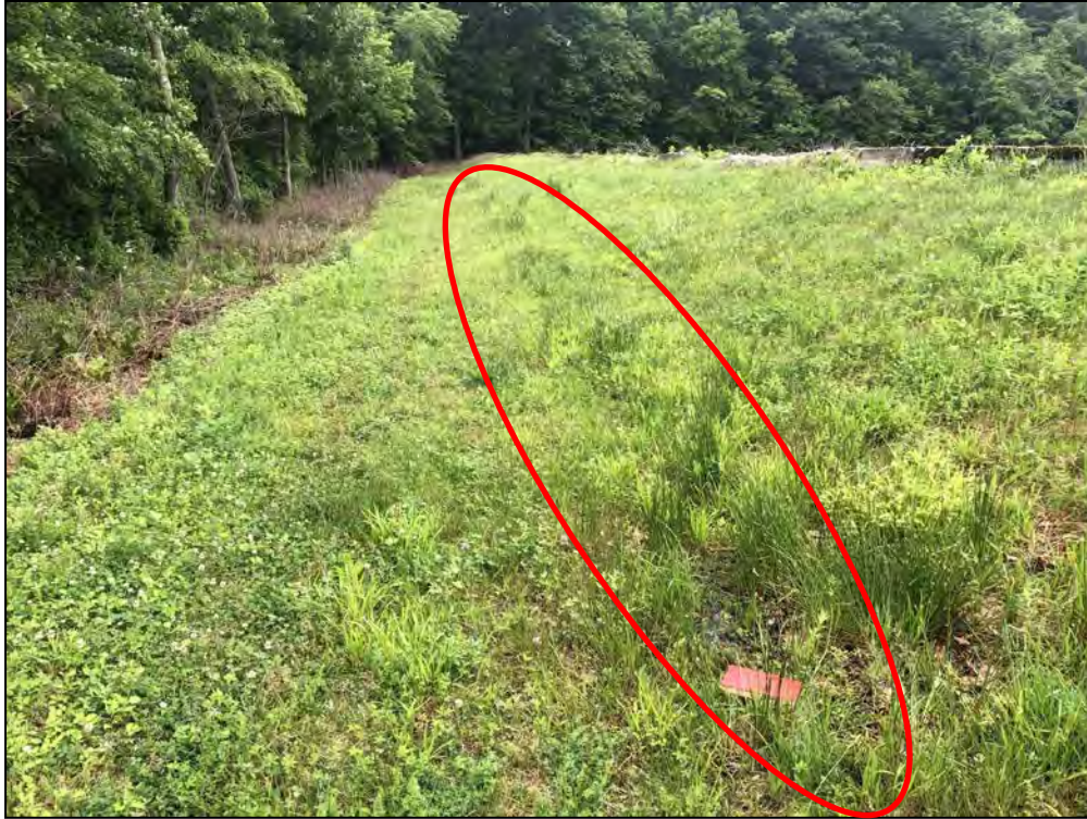
Photo No. 59: Spillway Section – Downstream slope from near STA 2+50 looking right. The locations of the saturated areas are evidenced by tall grass at the toe of the slope.
