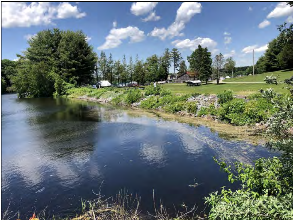
Photo No. 44: Pine Ledge Road to West Greenville Road Dam – Upstream side of the dike from Pine Ledge Road looking left.
