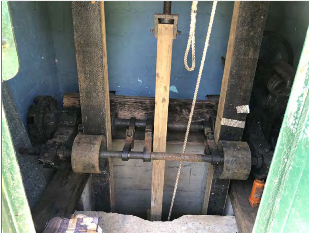
Photo No. 17: Main Dam - Gate controls within the interior of the outlet structure.
