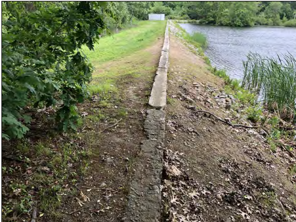
Photo No. 58: Spillway Section – Upstream slope and crest from near the left abutment looking right.
