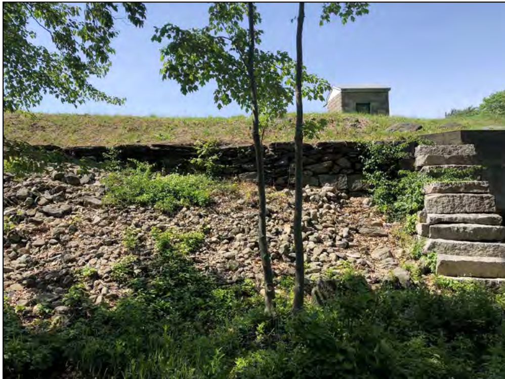
Photo No. 10: Main Dam - Downstream wall and area right of the low-level outlet wall.
