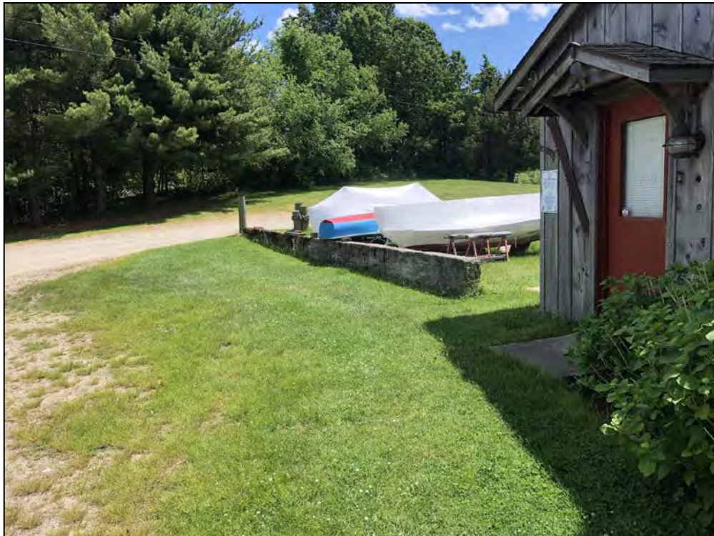
Photo No. 42: Marina Dam – Overview of the floodwalls left of the storage building.
