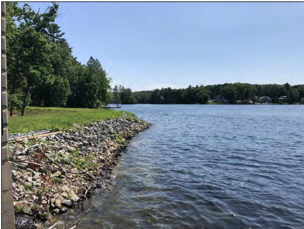
Photo No. 2: Main Dam - Upstream side of the dam from near the gatehouse looking left.
