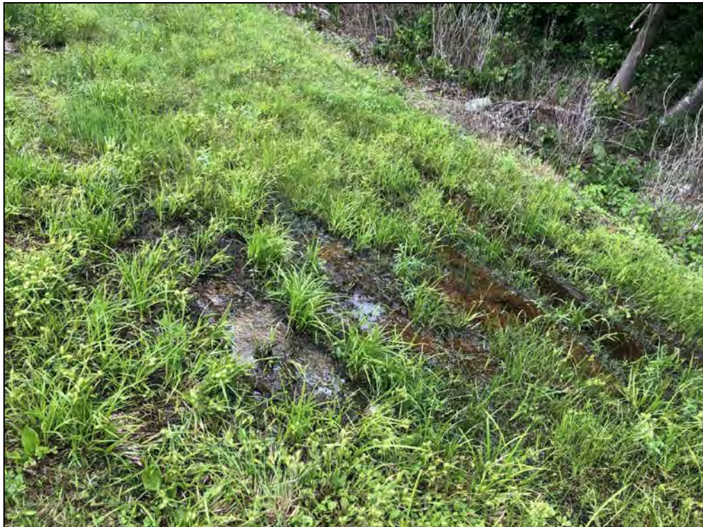
Photo No. 60: Spillway Section – Tire rutting with seepage near STA 1+70 along the toe of the slope.
