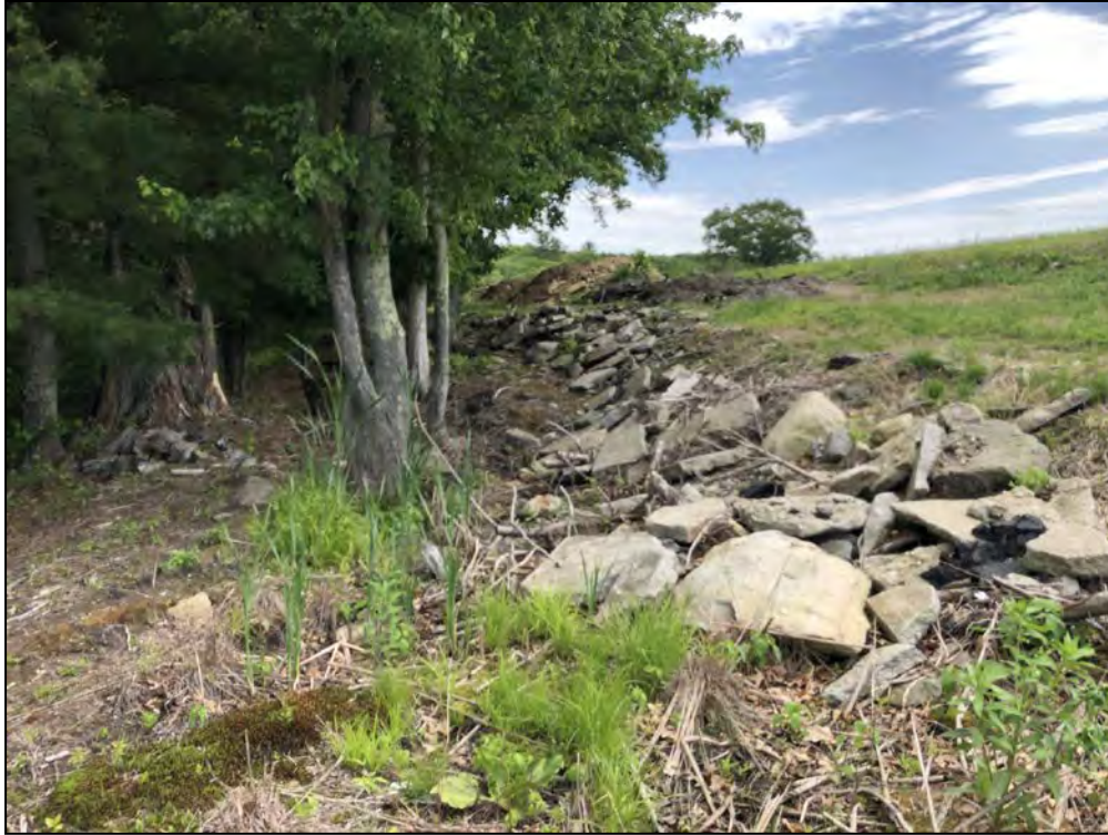
Photo No. 35: Bookers Dam – Concrete debris dumped along the downstream slope near STA 12+00.
