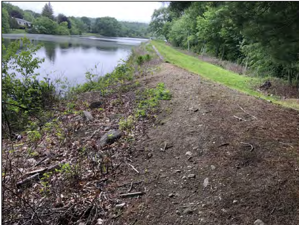
Photo No. 54: Spillway Section – Upstream slope from the right embankment looking left.
