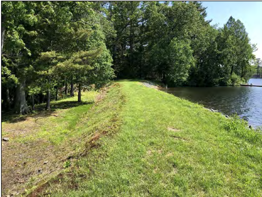
Photo No. 6: Main Dam – Crest from right of the low-level outlet looking right.
