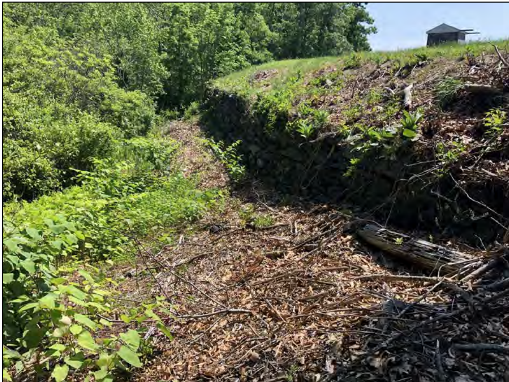
Photo No. 8: Main Dam - Area downstream of the downstream wall from near the left abutment looking right.
