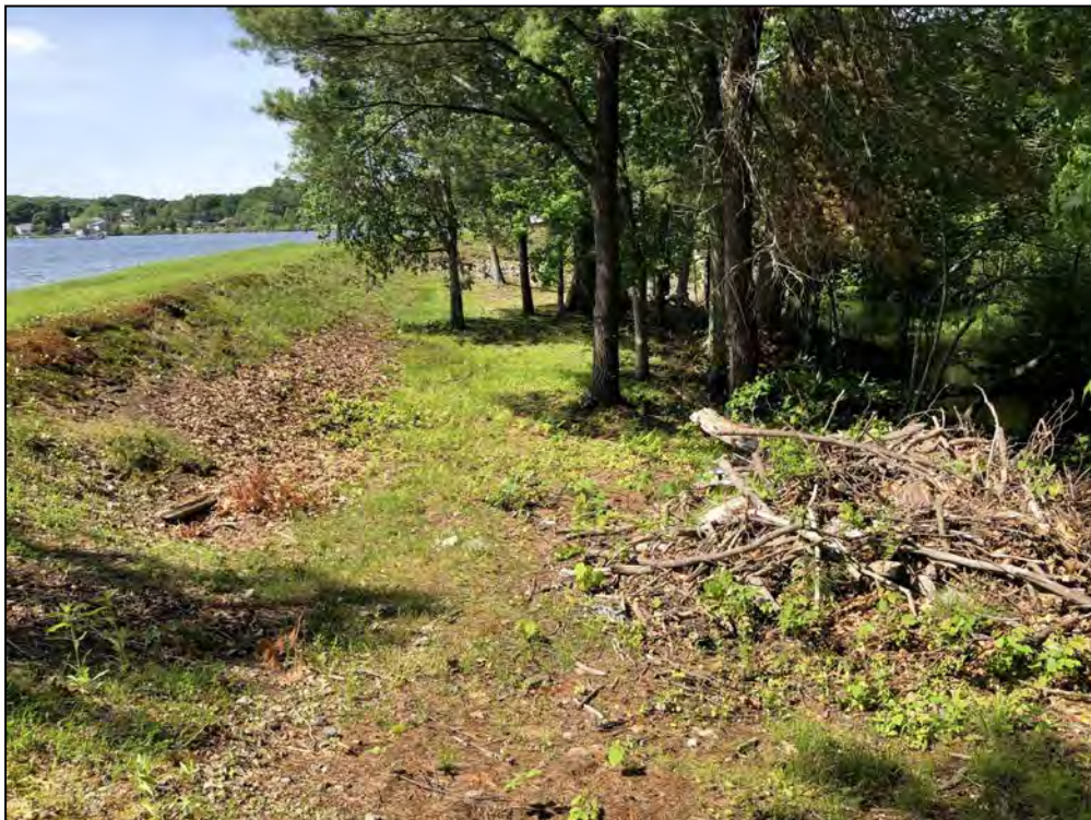
Photo No. 12: Main Dam - Downstream side of the embankment from near the right abutment looking left.
