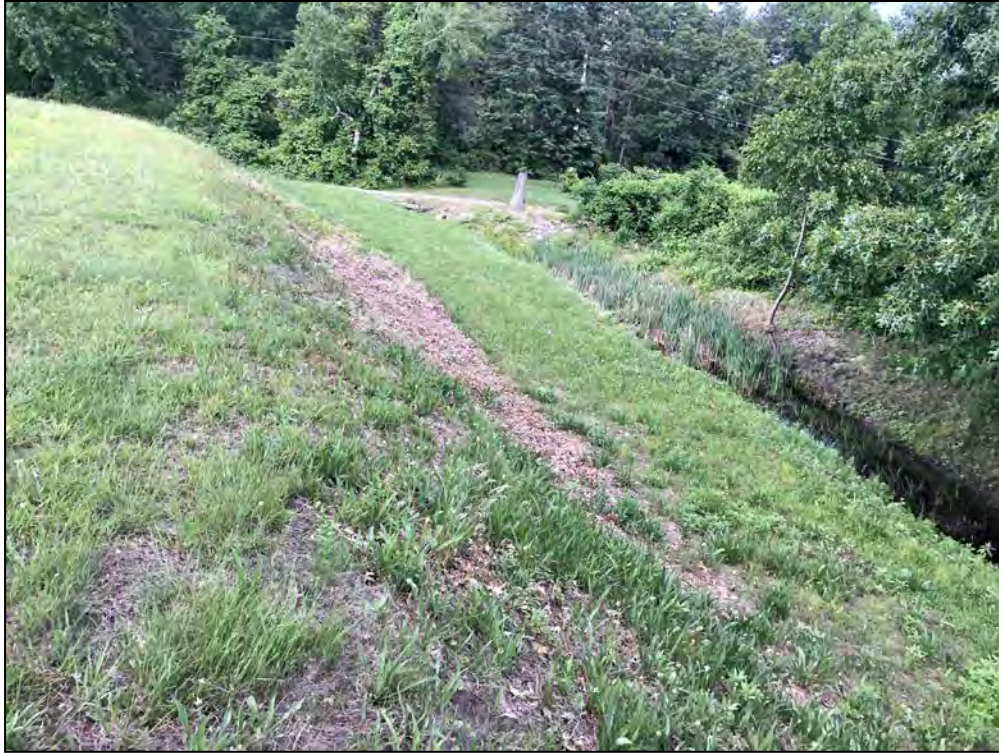
Photo No. 33: Bookers Dam - Downstream slope from near STA 6+00 looking left. Note the seepage channel along the downstream end of the embankment.
