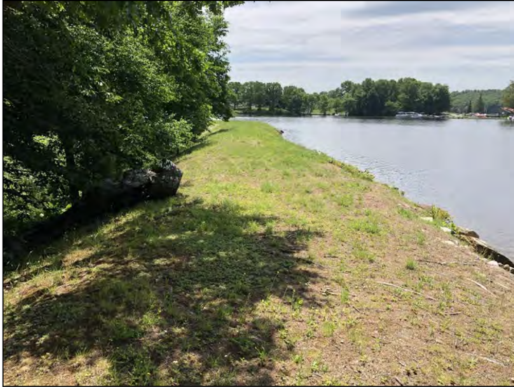
Photo No. 29: Bookers Dam - Crest from near the left abutment looking right.
