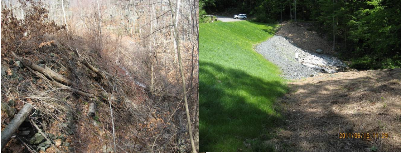
Same view of downstream slope of Limerock Dam (No. 295), Lincoln, before and after work
