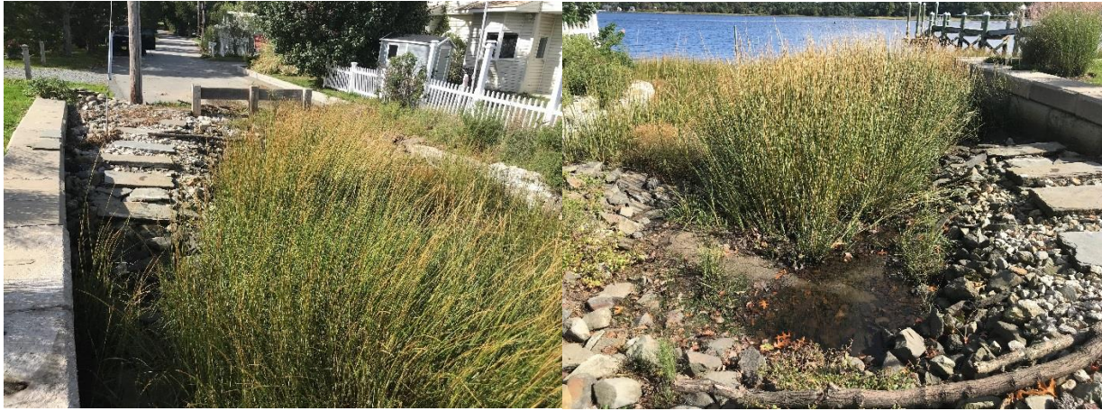
Figure 2: Source 5-030, an 18” corrugated metal pipe at the end of Smith Street, Warren, RI. View inland (left photo) and view toward the Kickemuit River (right photo). No detectable flow was present when examined on 10/16/2018.
