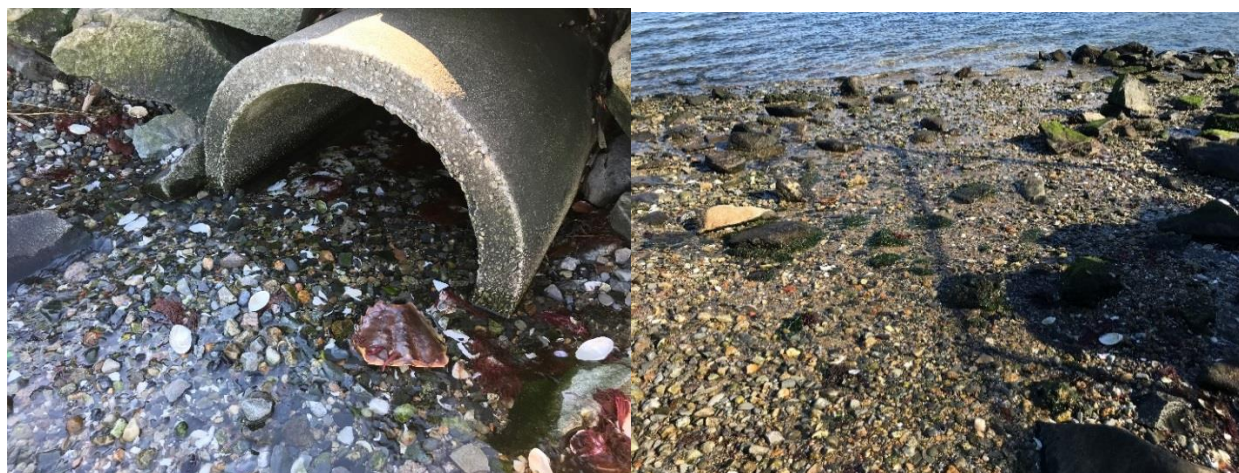
Figure 3: Source 16-001 showing discharge out of 24” RCP (left) and trickle flow across narrow beach to receiving waters (right image). Photos taken 10/22/2018.
