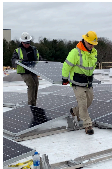
Rooftop Solar Array
