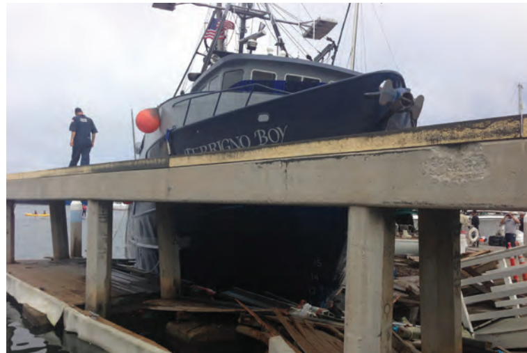
Figure 4: Damage to pier, pilings, and floating dock at Ventura Harbor Boatyard. PHOTO BY COAST GUARD
