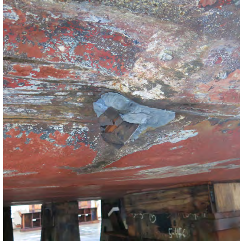
Figure 57: Breached hull on the fish-processing vessel Gordon Jensen 's port side.
