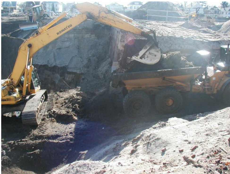
Photo 4. View south. Removal of NAPL soils near concrete bunker at west end of excavation.
