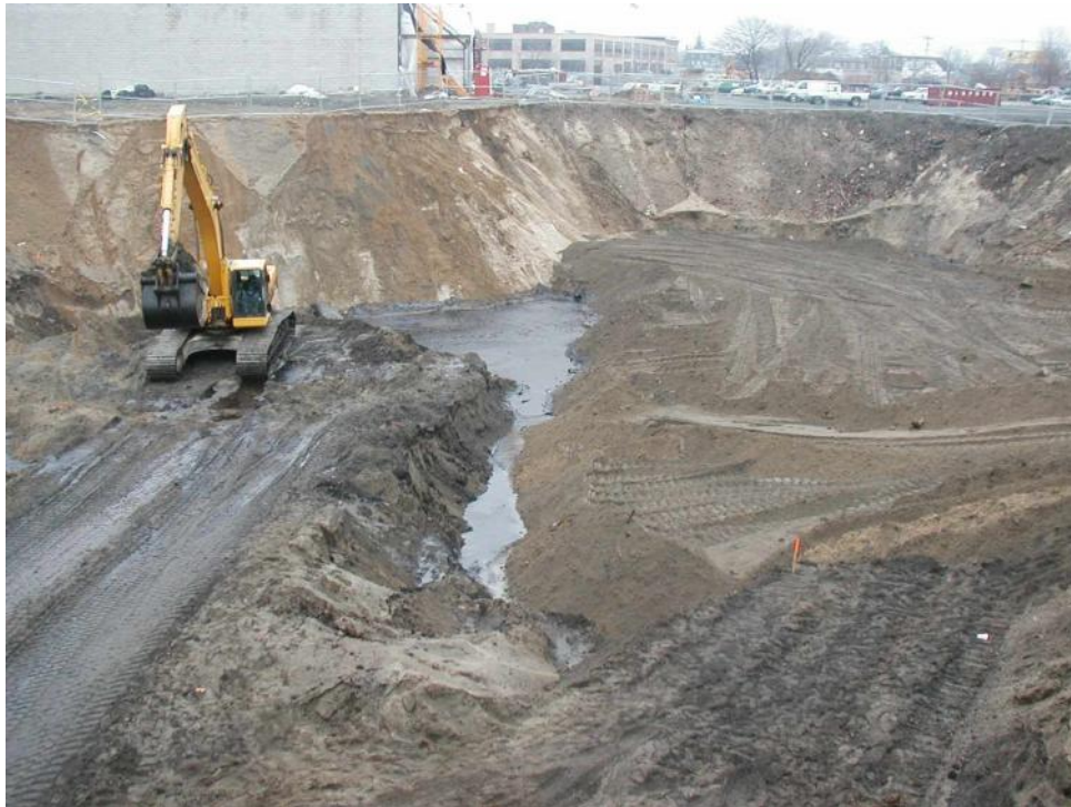
Photo 1. NAPL excavation looking east. Clean backfill on right side, excavation of NAPL soils on the left.
