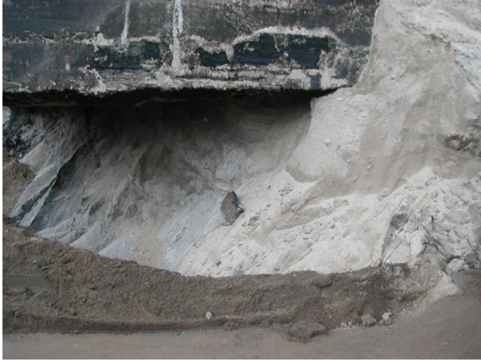
Photo 9. Clean soil beneath bunker. Note crack developing in bunker wall just to the right of top center in the photo.
