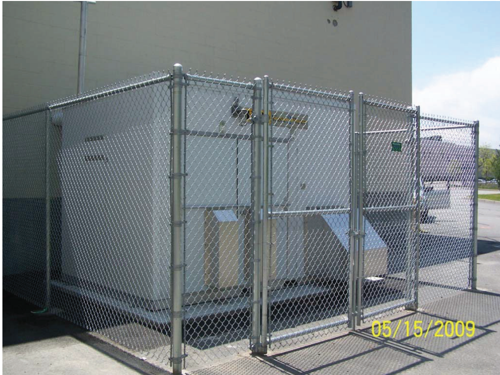
ASD Enclosure Inside 8 ft Chain Link Fence
