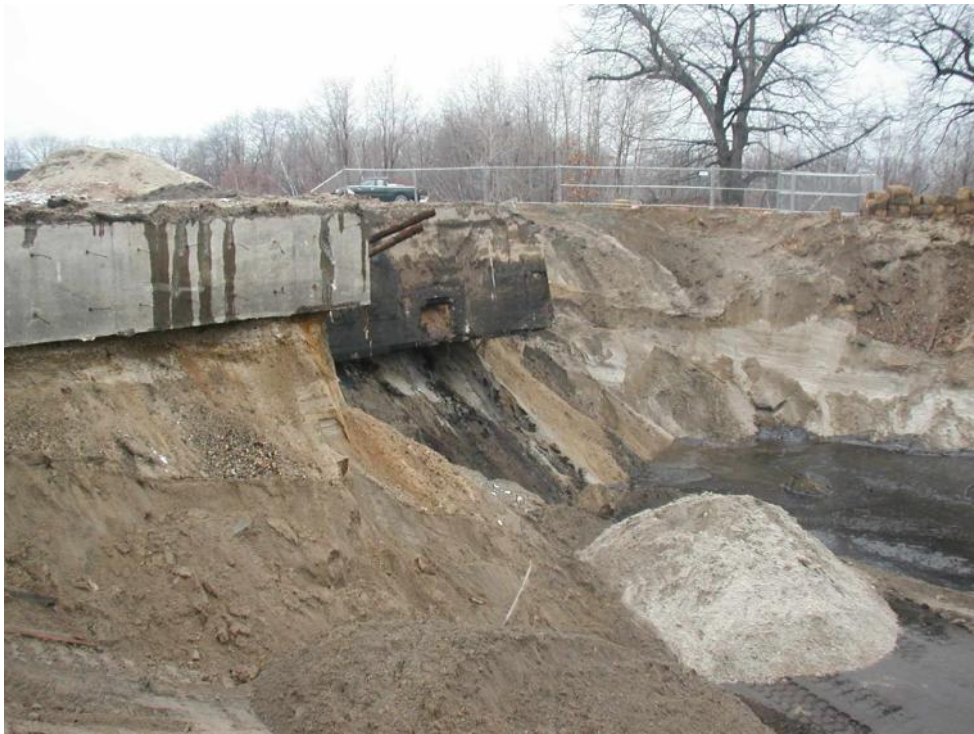
Photo 8. View towards northwest with much of the soil on east side of concrete bunker removed.
