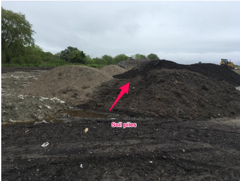
Soil piles located at end of road
