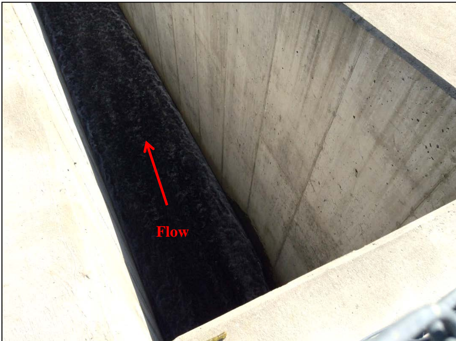
Photo No. 42: The primary spillway by-pass outlet discharge channel as viewed from the gate control looking downstream after the gate was opened.
