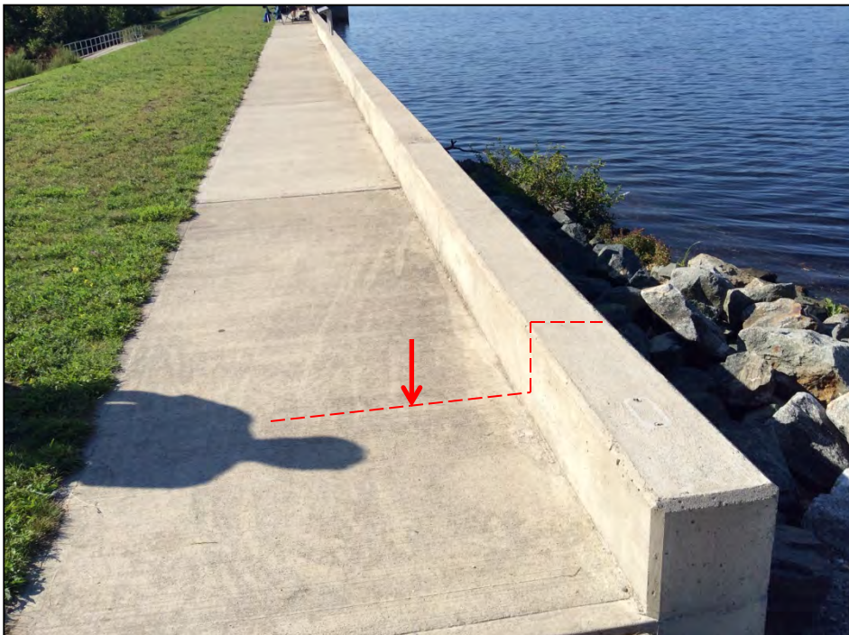
Photo No. 4: Continuous hairline crack along the sidewalk and through the upstream wall as viewed from the left abutment looking right.
