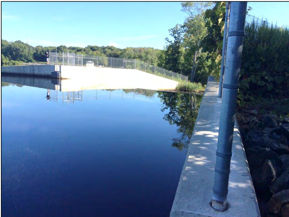
Photo No. 38: The primary spillway approach as viewed from the right looking downstream from the water line.
