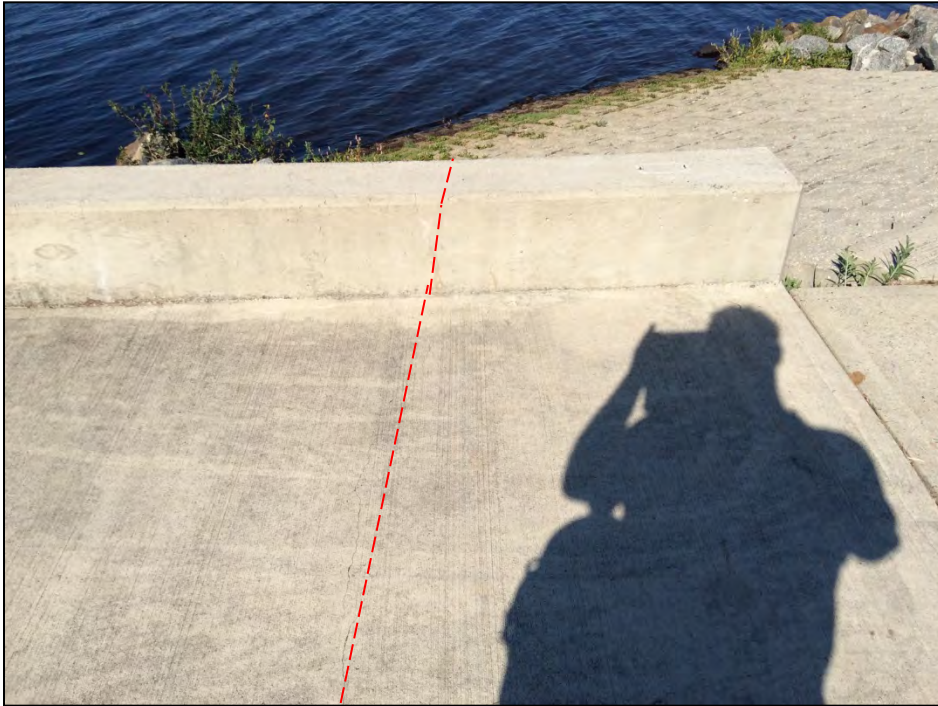
Photo No. 5: View of the cracks along the sidewalk and upstream wall at the left-most wall section (near the left abutment) looking upstream.
