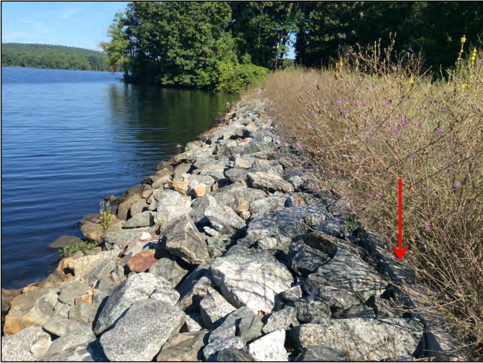
Photo No. 27: Right Dike: The upstream slope as viewed from near station 17+40 looking left. Note the concrete wall at the top of the riprap.
