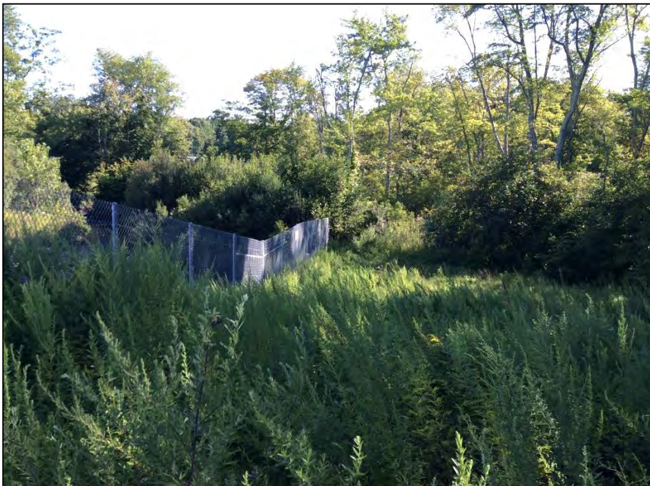
Photo No. 16: The downstream slope right of the primary spillway as viewed from the crest looking downstream. Note the tall grass and weeds.
