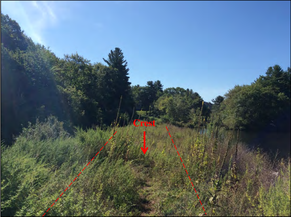
Photo No. 30: Right Dike: The crest as viewed from the left abutment.
