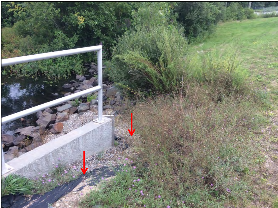
Photo No. 58: Erosion behind the right side of the low level outlet downstream headwall. Photo looking right and slightly downstream. Erosion is typical along both sides except there is more bare ground on the left side.
