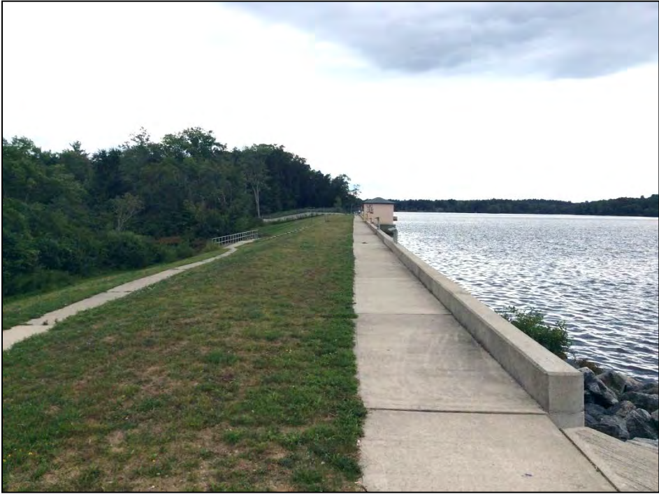
Photo No. 11: An overview of the crest as seen from the left abutment.
