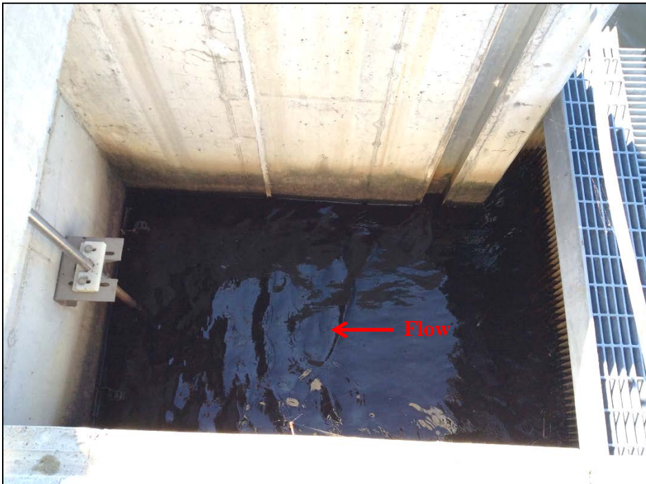
Photo No. 48: The primary spillway by-pass outlet approach as seen from the left.
