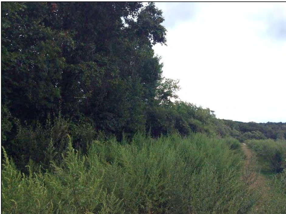
Photo No. 22: Left Dike: The downstream slope as seen from the left abutment. Note the thick overgrowth of tall grass weeds that limited access for a visual inspection.
