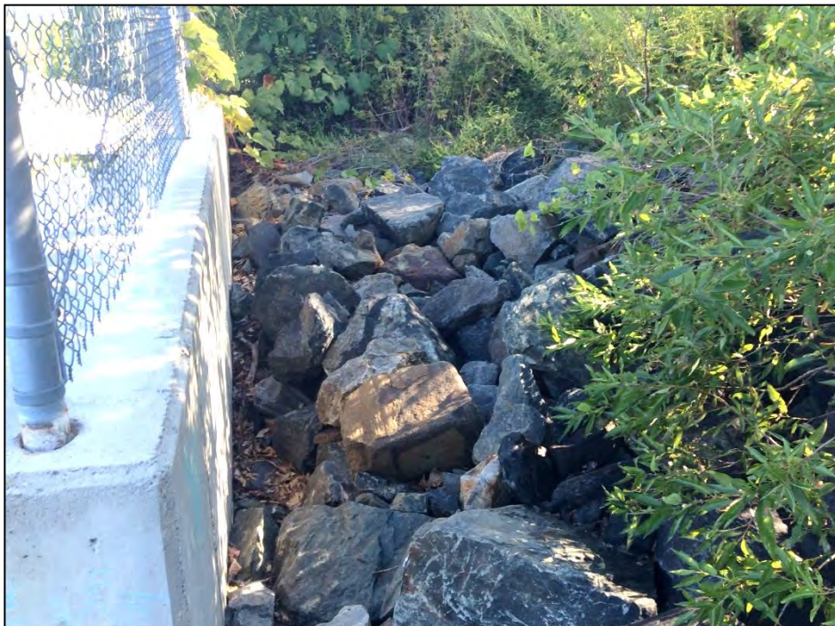
Photo No. 10: An eroded area behind the primary spillway left upstream wingwall looking downstream.
