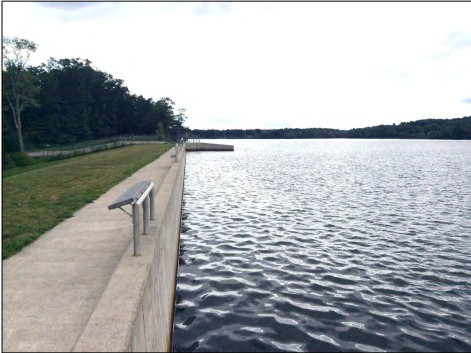
Photo No. 7: The upstream side as seen from right of the gatehouse looking right.
