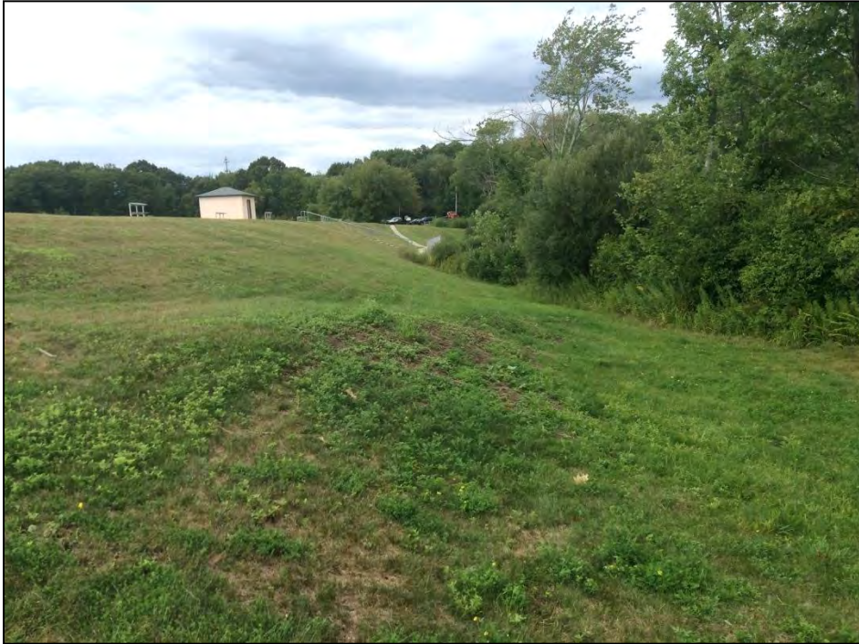
Photo No. 15: The downstream slope as seen from near station 10+00 looking left.
