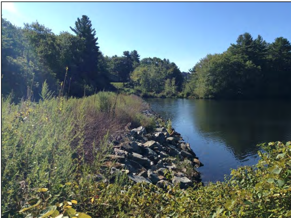
Photo No. 26: Right Dike: The upstream slope as viewed from the left abutment of the right dike.
