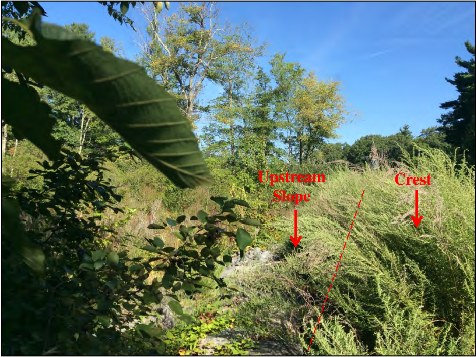
Photo No. 29: Right Dike: The upstream slope as viewed from the right abutment.
