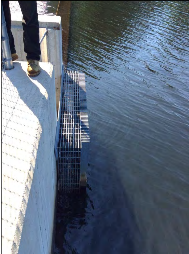
Photo No. 49: The trash rack at the outlet approach as viewed from the left.
