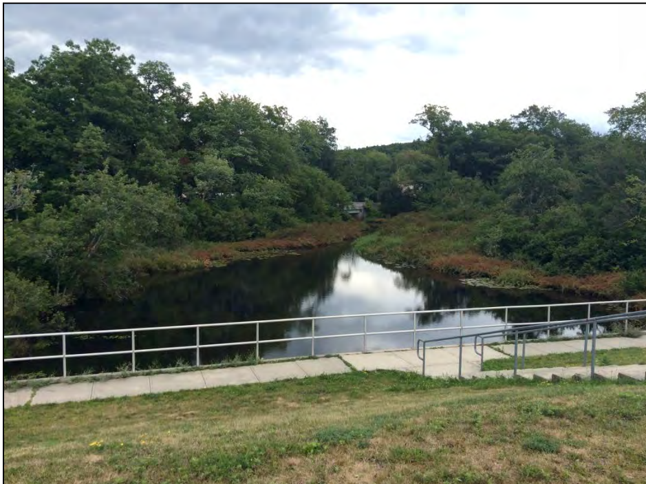
Photo No. 56: The low level outlet discharge channel as seen from the crest.
