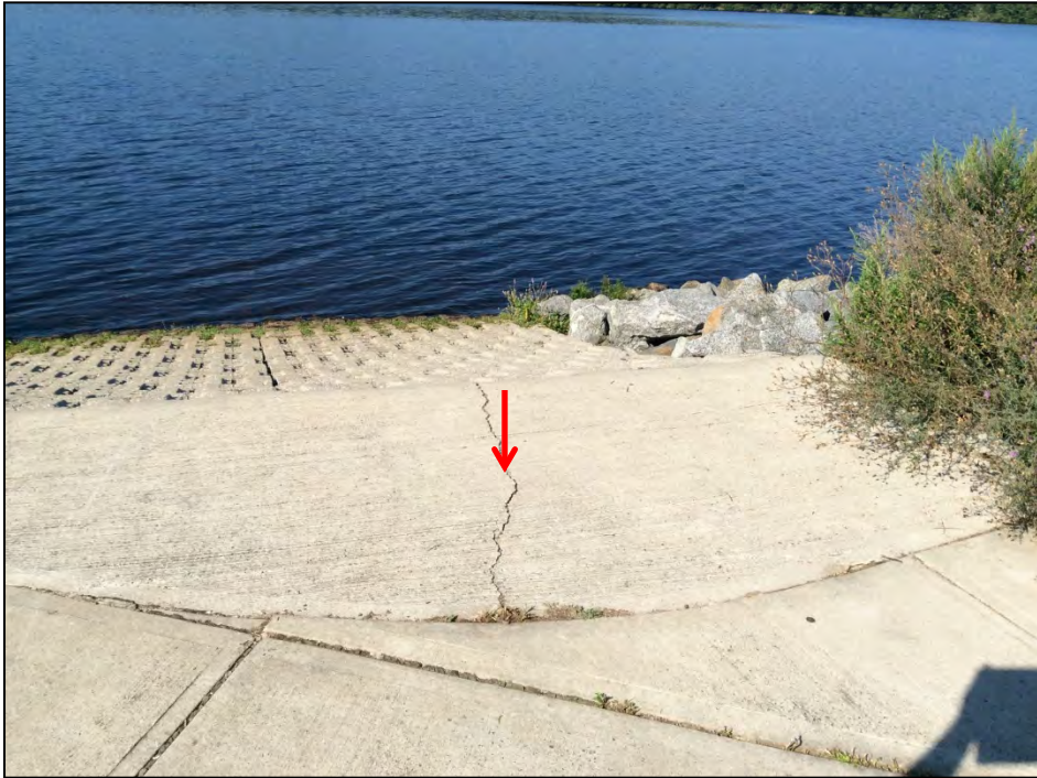
Photo No. 3: A crack within the concrete at the top of the boat ramp located near the left abutment. The width of the crack was measured at 1/4 inch wide.
