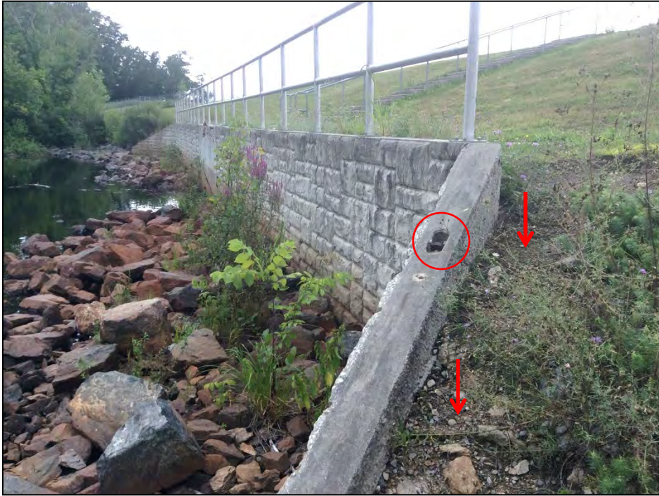
Photo No. 59: Overview of the low level outlet downstream headwall as seen from the left. Note the erosion behind the wall. The circled area is a former lifting eye used for installing the pre-cast wall section.
