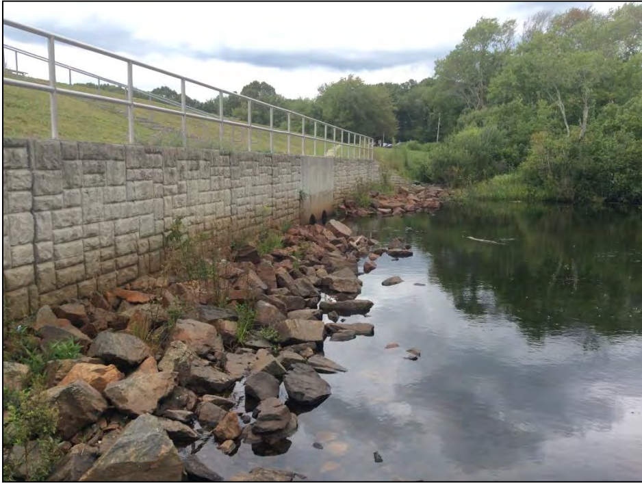
Photo No. 57: The low level outlet downstream headwall as viewed from the right. Note the staining within the riprap and along the wall.
