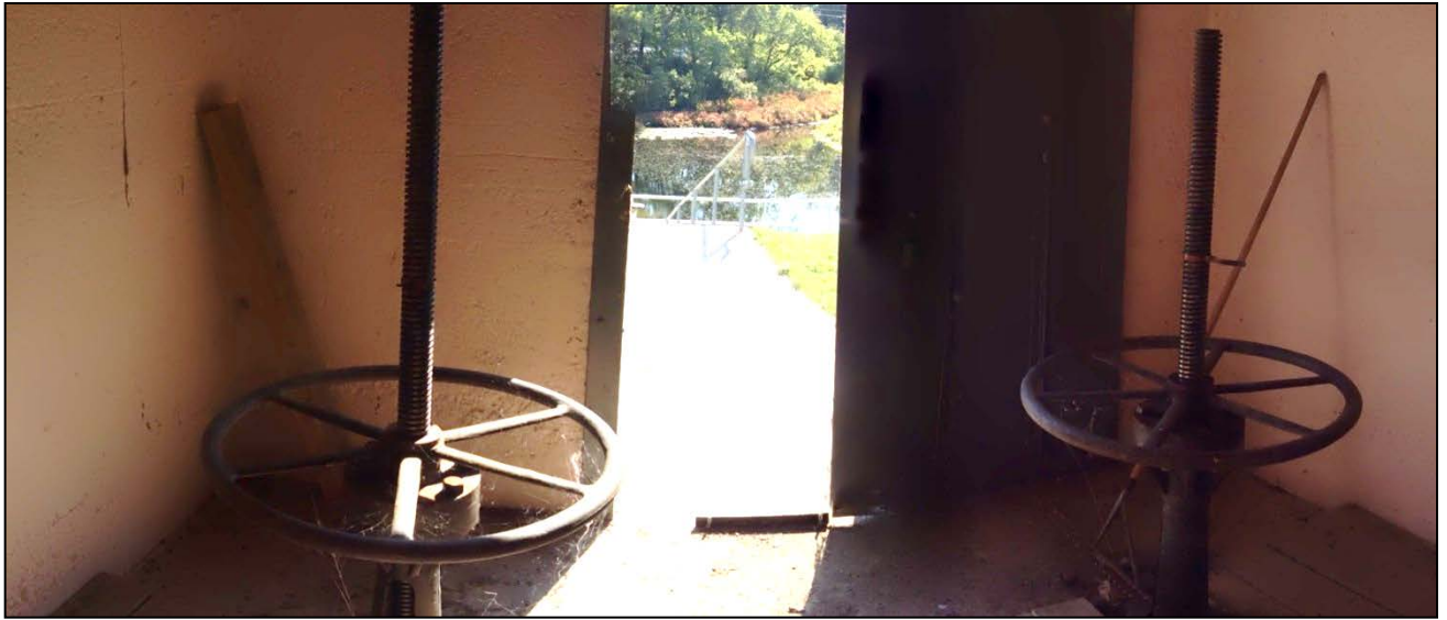
Photo No. 55: The hand wheels that control the two gates within the original gatehouse. Photo looking downstream.
