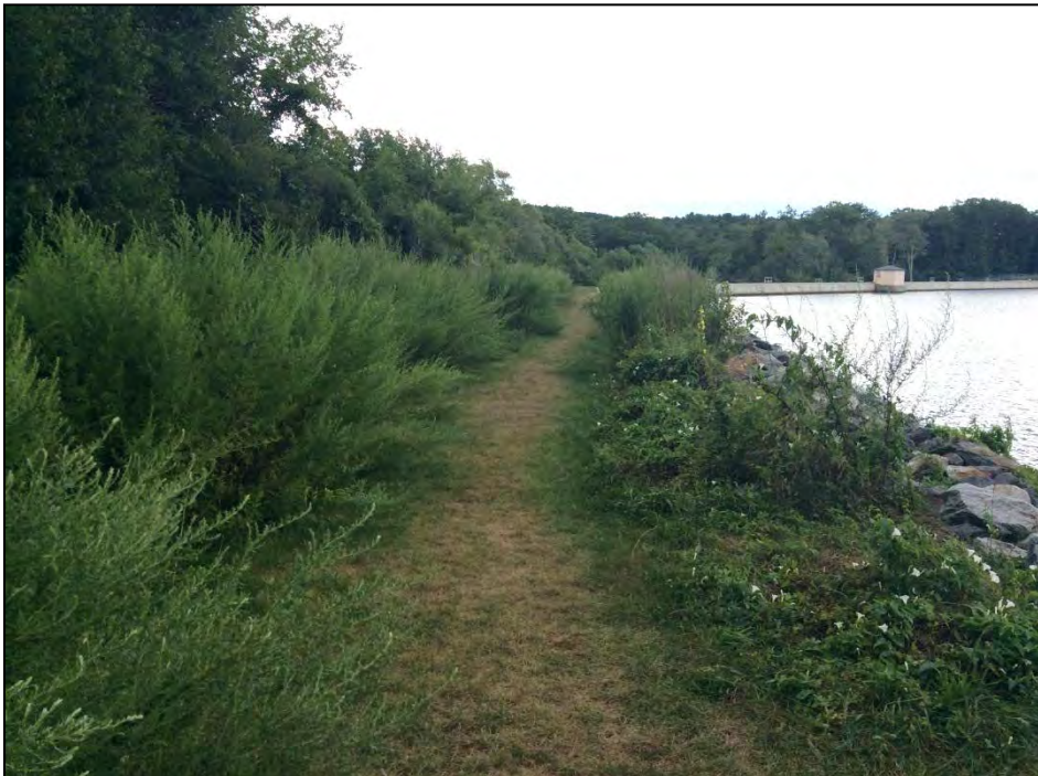
Photo No. 20: Left Dike: An overview of the crest as seen from the left abutment. Note the vegetation along both the upstream and downstream shoulders, limiting inspection.
