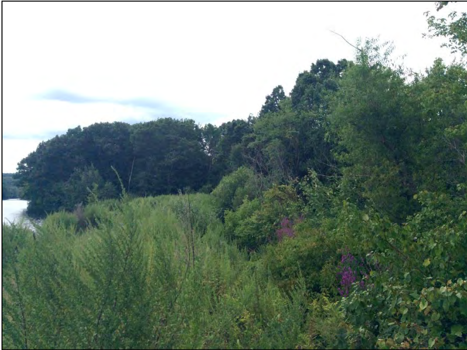
Photo No. 23: Left Dike: The downstream slope as viewed from the right abutment. Note the thick overgrowth.
