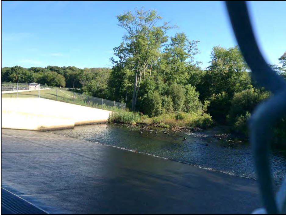
Photo No. 41: The primary spillway discharge apron as viewed from the embankment crest right of the spillway looking downstream and slightly left.
