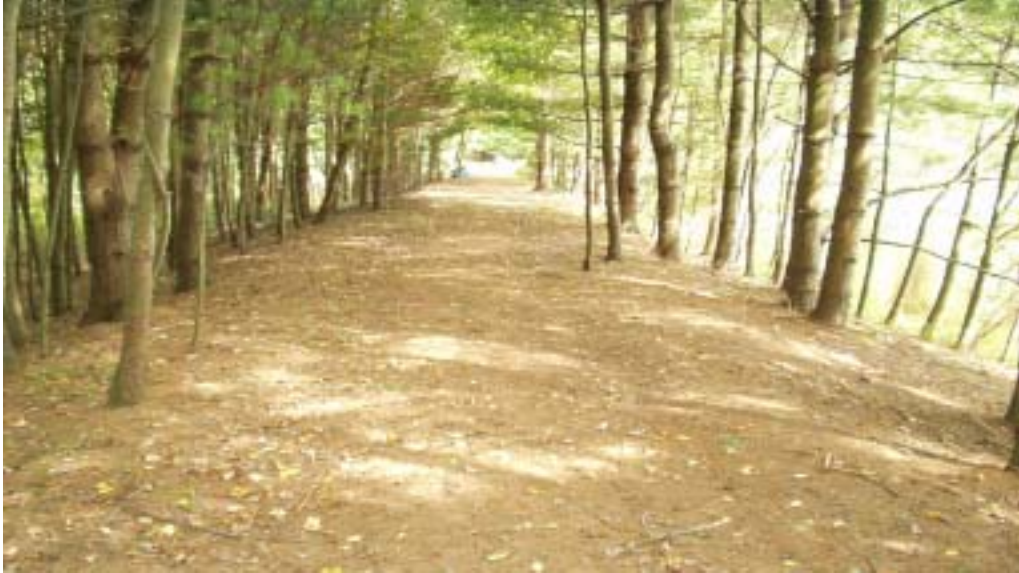
Improperly vegetated embankment at T. Wright Farm Pond Dam (No. 587), Gloucester
