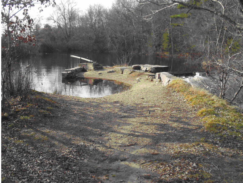
Eroded Embankment at Coventry Reservoir Dam (No. 176), Coventry
