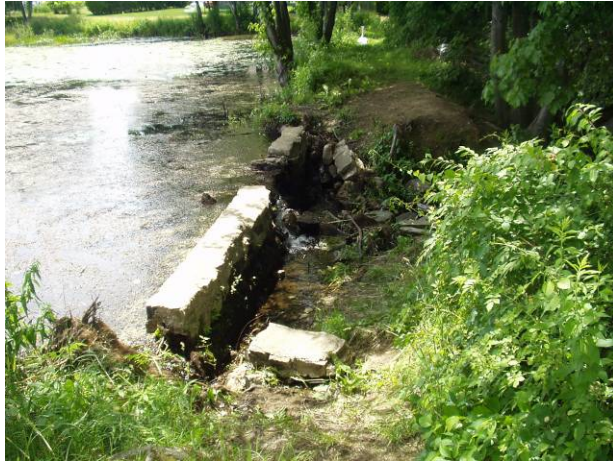
Spillway prior to repair (pond on left)
