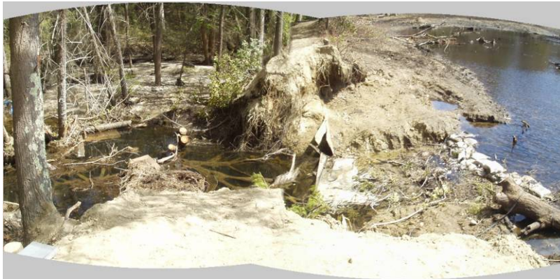
Breach in New Dam (No. 397), Gloucester
