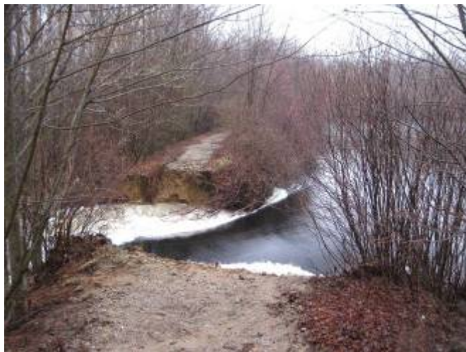
Breached section of Blue Dam (No. 229) in Hopkinton
