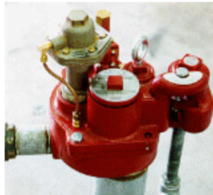
Figure 3 STP with Line Leak Detector
