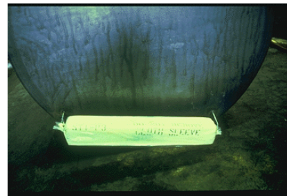
Figure 12 Sacrificial Anode Attached to UST
