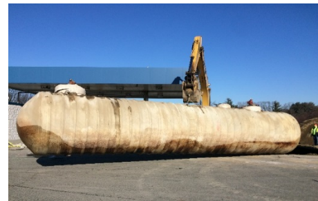
Figure 1 FRP Tank, Warwick, RI
