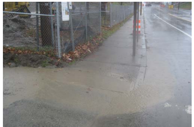
Sediment-filled runoff from a RIDOT construction site
