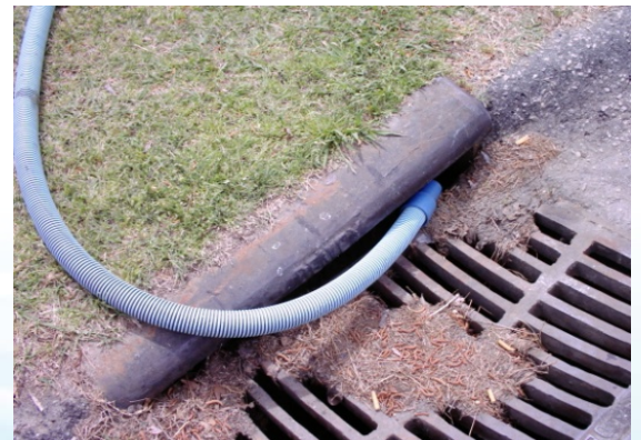
Sump pump connection to a storm drain
