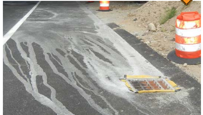
Concrete washout pollution, an example of an illicit discharge, is flowing directly into a storm drain on this RIDOT site.
