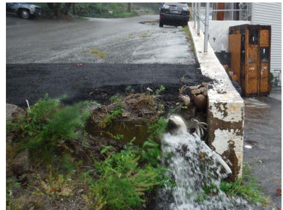
Stormwater discharge to roadway system found during construction. If allowed to remain, additional flow must be managed.
