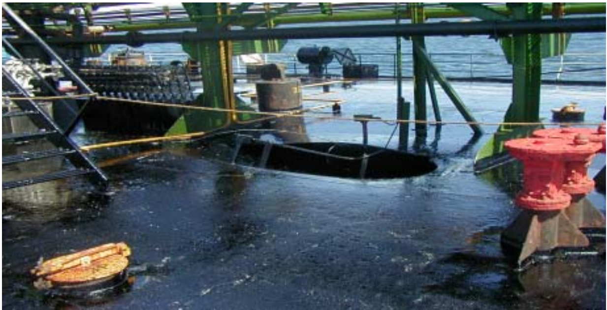
Asphalt Victory: Deck implosion and oil staining.
