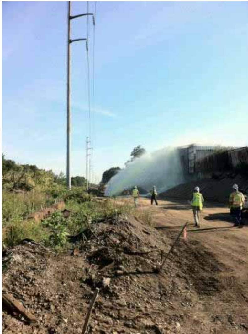
Figure 9 Capitol Pipeline shooting diesel 100 feet in the air.
