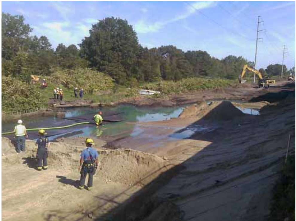
Figure 10 pumping the free oil on the ground at the break site.
