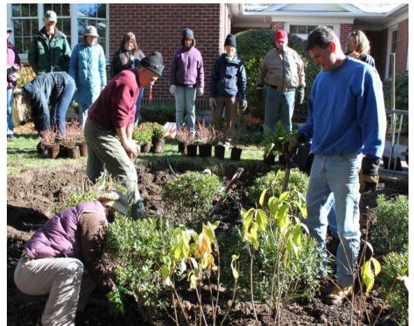
Fall 2011 RI Residential Rain Garden Training participants install a 200 square foot garden at the Louttit Library to collect, treat, and infiltrate 1 inch of runoff from a portion of the roof.
