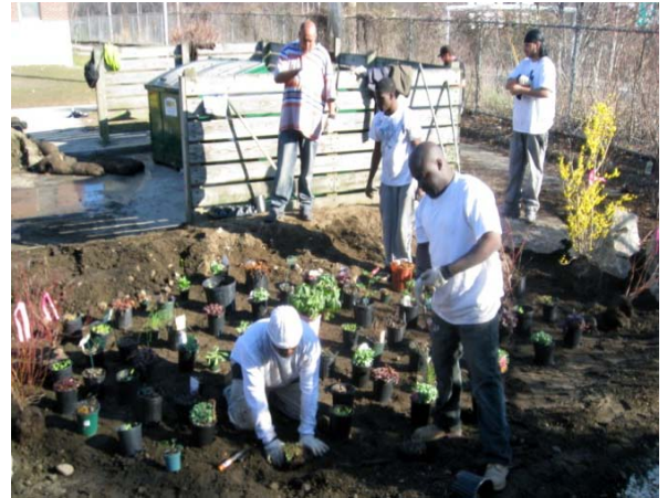
Providence GroundWorks trainees install a 320-square foot rain garden in the Manton Heights Housing Development to collect, treat, and infiltrate runoff from a portion of an adjacent parking lot.
