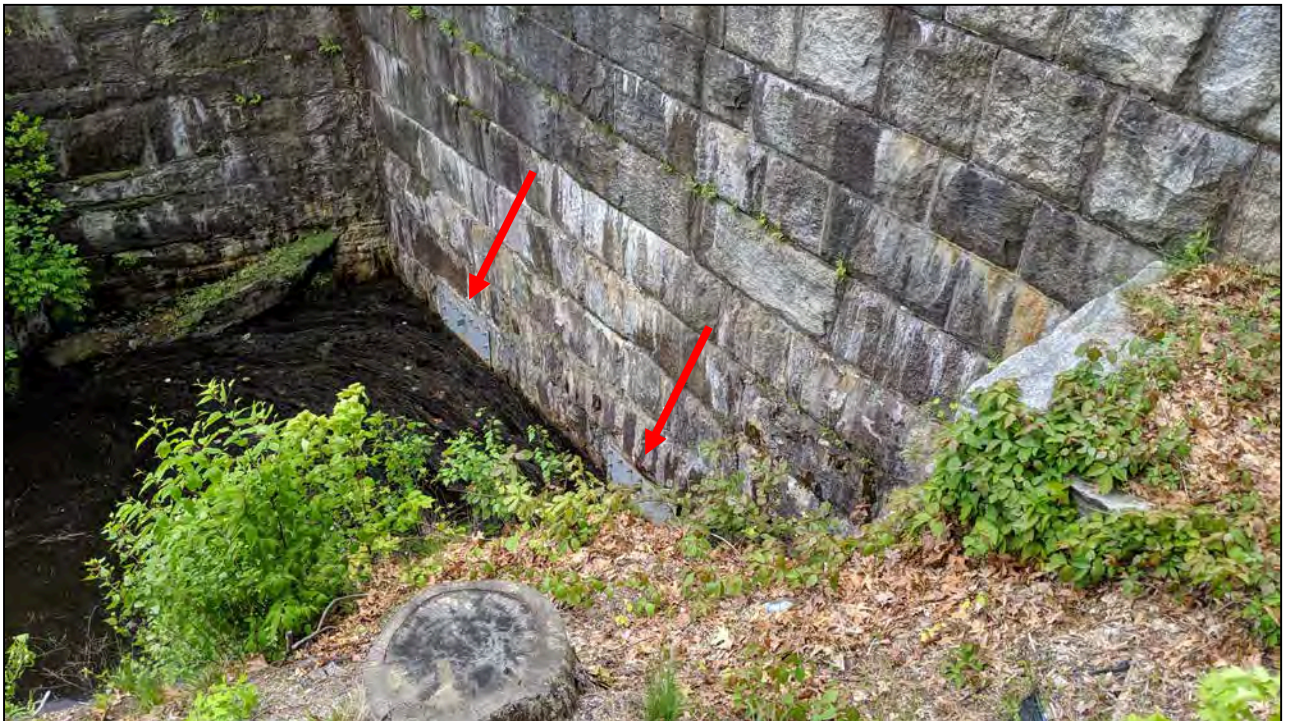
Photo No. 10: Plugged downstream outlets of the low-level outlet
