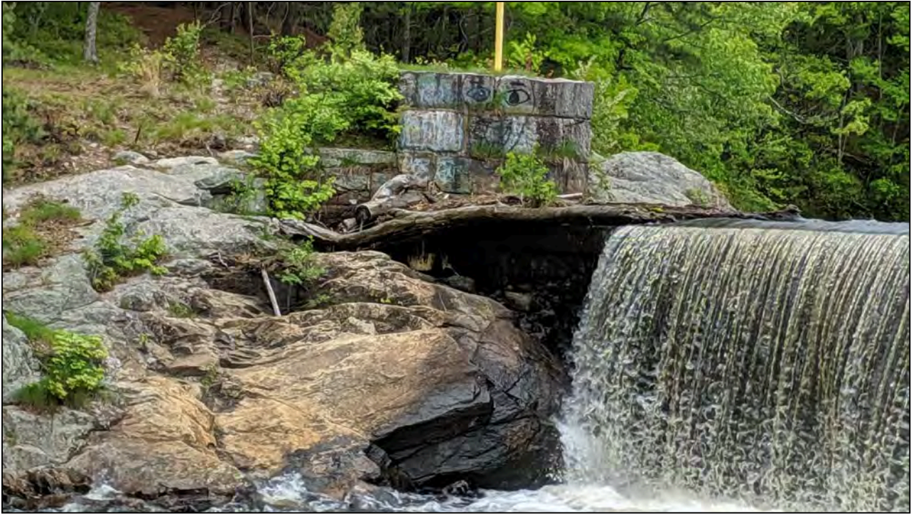
Photo No. 9: Right abutment contact and downstream face of the primary spillway. Note debris spanning the spillway crest and downstream bedrock outcrop. Staining on the bedrock outcrop indicates that high flows have passed over the debris without removal.
