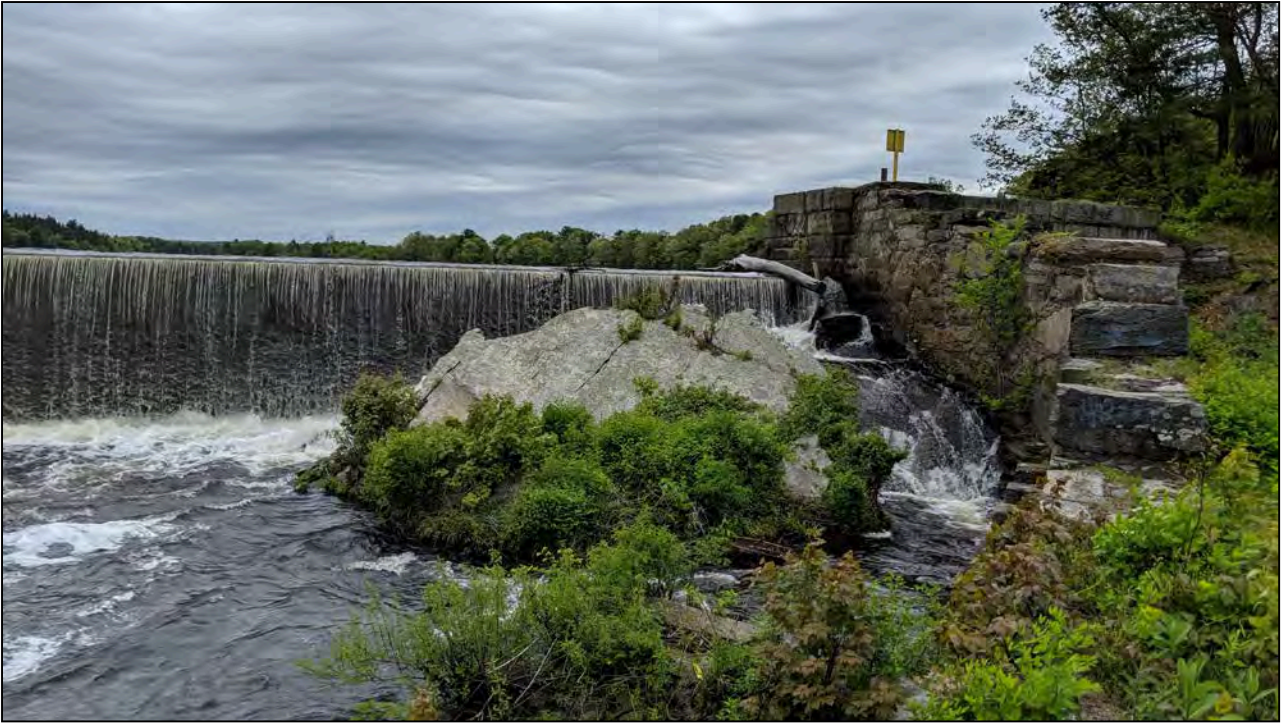
Photo No. 7: left downstream face of the primary spillway and left downstream channel wall. Note the tree trunk lodged on the crest, the bedrock outcrop in the immediate downstream area, and the vegetation growing from the downstream channel wall..
