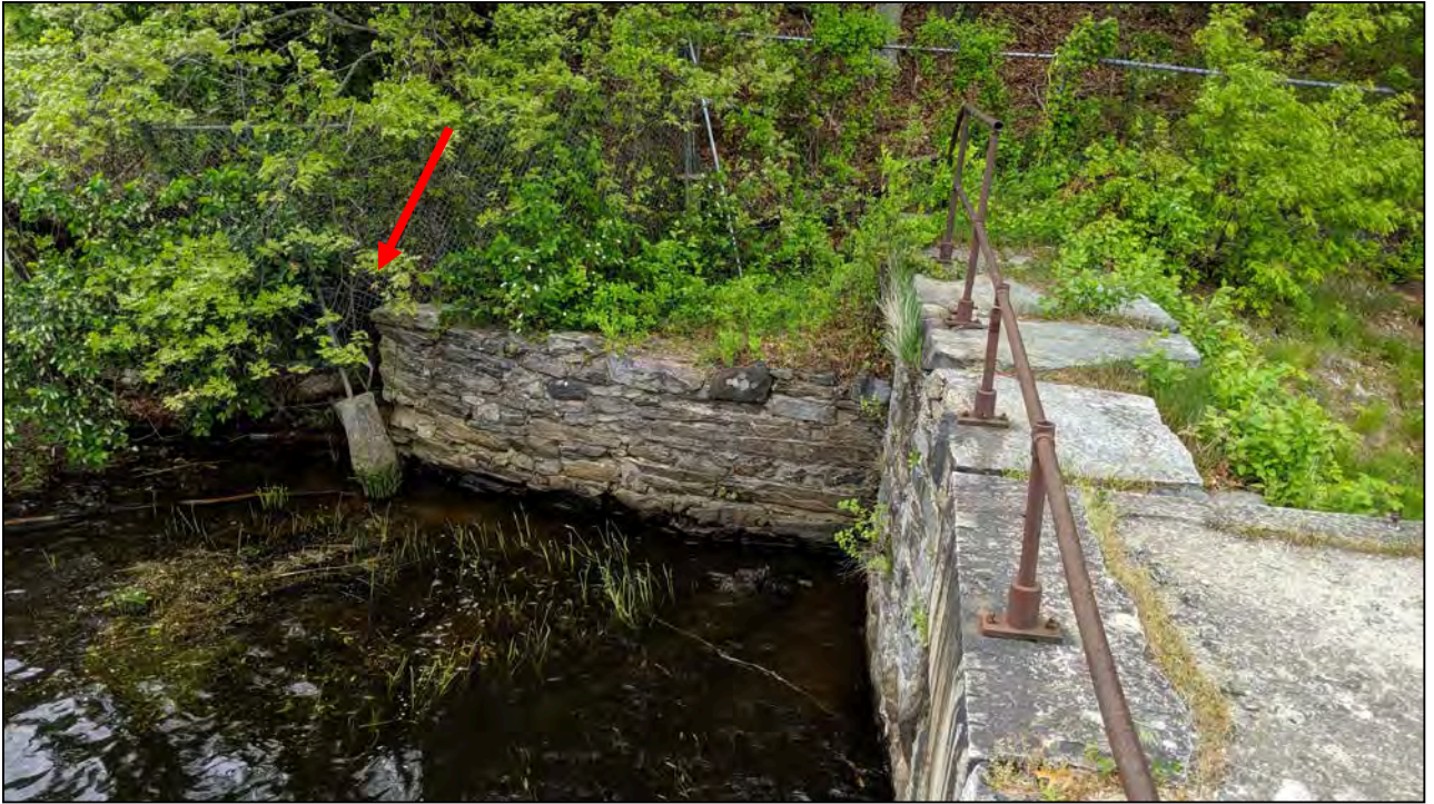
Photo No. 1: Upstream left abutment contact. Note collapsed fence post due to erosion behind the wall.
