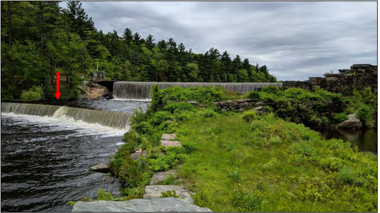
Photo No. 15: Primary spillway discharge channel from the downstream area looking upstream. The arrow indicates the downstream toe dam (Slatersville Upper Intermediate Dam RI#045).
