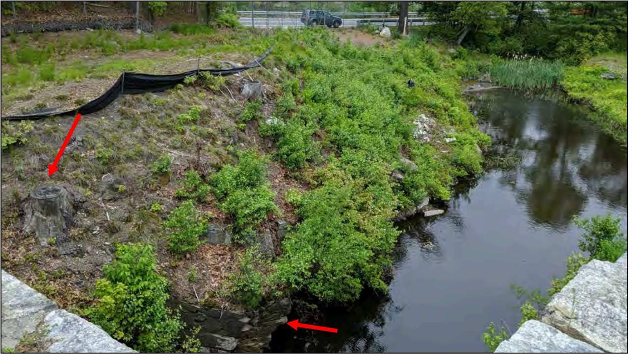
Photo No. 13: Low-Level outlet discharge canal and left canal slope. Note bedrock outcrop and stumps along the slope..
