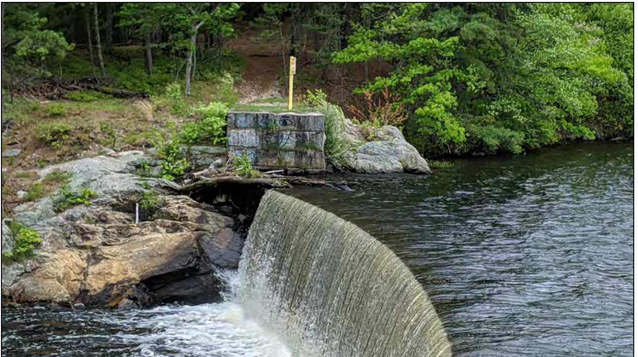
Photo No. 4 : Right abutment as viewed from the left side of the primary spillway.
