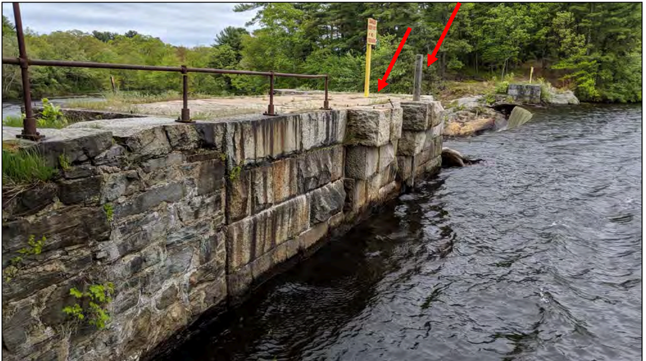
Photo No. 2: Upstream wall between the left abutment and primary spillway. Arrows indicate the low-level outlet gate stem (right) and former operator locations (left & right).
