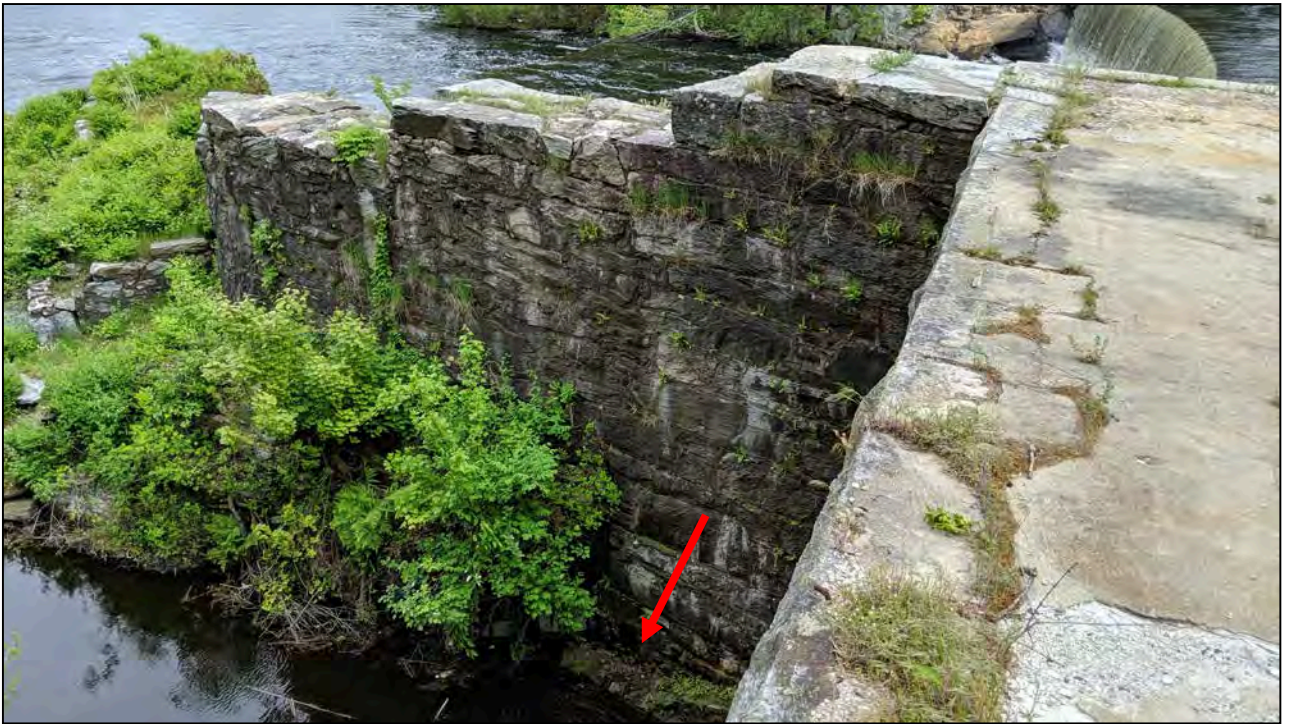
Photo No. 11: Downstream right channel wall for the low-level outlet/left channel wall for the primary spillway. The arrow indicate the location of observed trace seepage from the wall.
